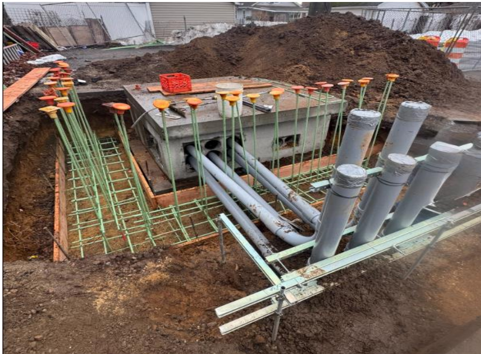
Hempstead IAQ – Paterson Transformer Pad
