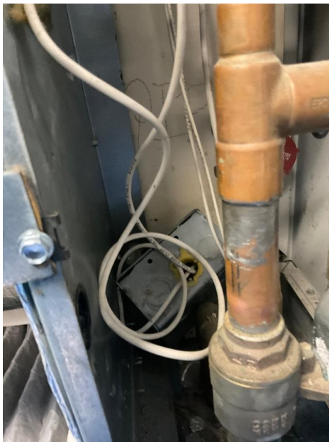
Junction Box.v2.jpg; Added on 6/14/2023 8:18:38 PM by danhailey@cm3inc.com
