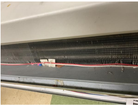
Wiring.v2.jpg; Added on 6/12/2023 9:43:49 PM by danhaihey@cm3inc.com
