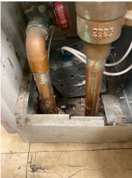
Junction Box.v2.jpg; Added on 6/13/2023 8:06:01 PM by danhainey@cm3inc.com
