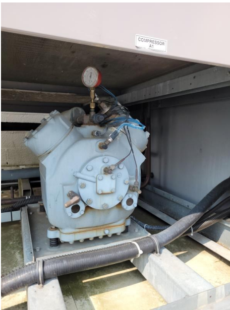
Compressor1.v2.jpg; Added on 5/24/2023 10:45:45 AM by danhainey@cm3inc.com
