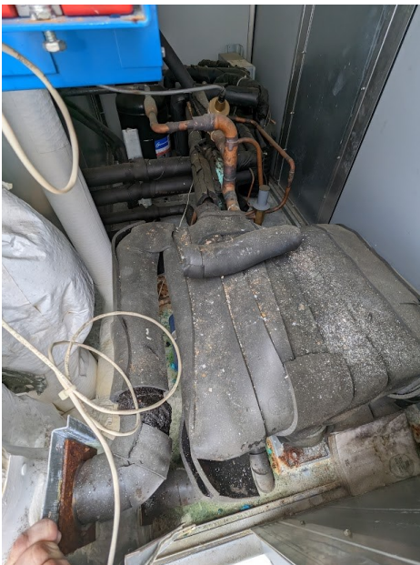
05871674_ERU5Leak2.jpg; Added on 7/7/2023 9:00:05 AM by dmychaluk@cm3inc.com
