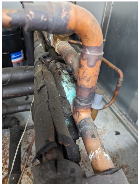
05949779_ERU5leak5.jpg; Added on 7/7/2023 9:00:05 AM by dmychaluk@cm3inc.com
