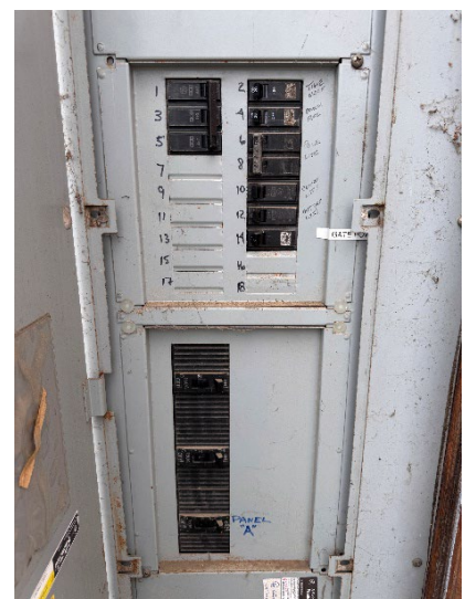
Figure 5: Parking Lot Main Distribution Panel
