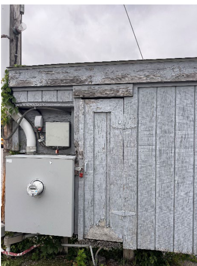
Figure 3: Service in Parking Lot
