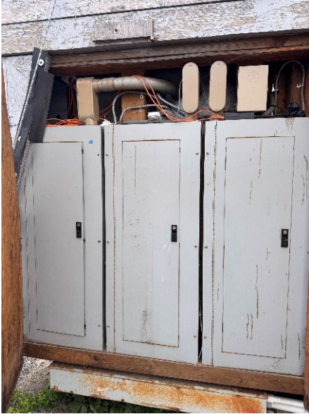
Figure 6: 150A Service Panels Feeding Parking Lot Equipment
