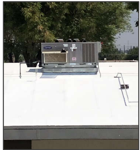
New HVAC Units
