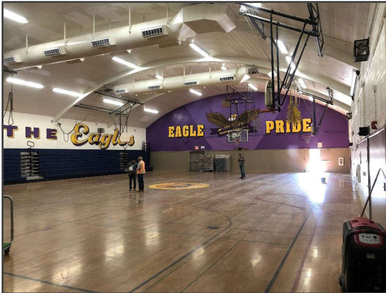
Existing Gym with new HVAC
