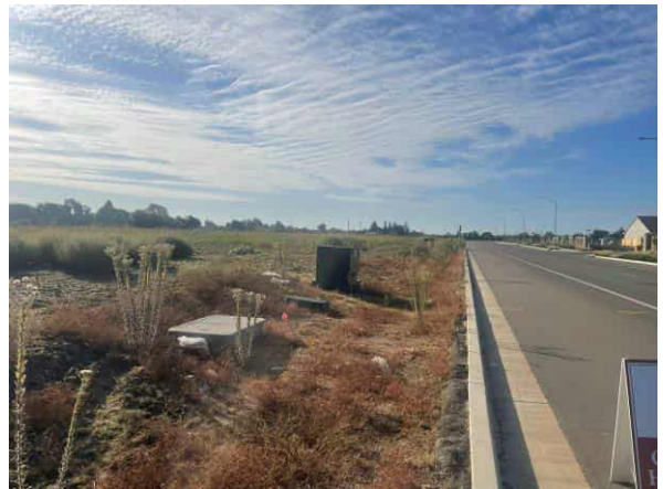
Photo #4 View of the pad-mounted transformer on the western boundary.
