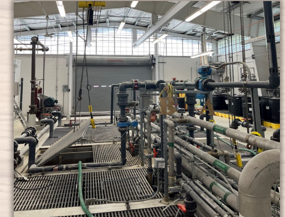
WASTEWATER TREATMENT FACILITY – 4,300 sq. ft (2009)
