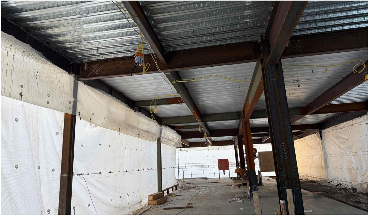
Temporary lights, L2
