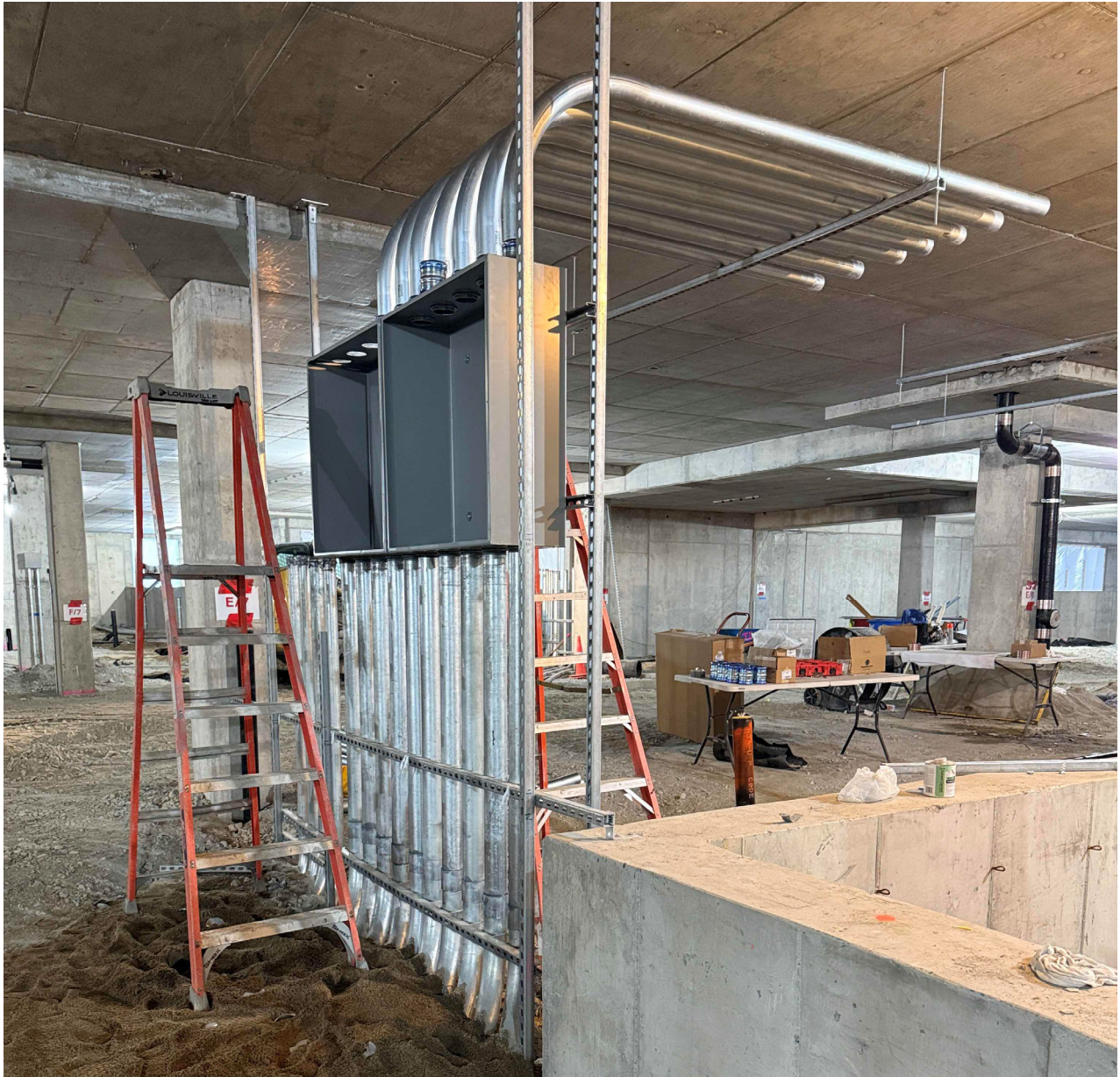
Electrical Conduit/Boxes, Building A - Garage Level
