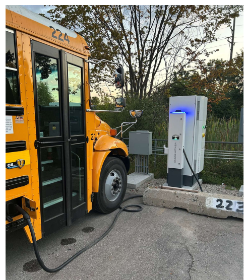
Bus EV Charging Station
