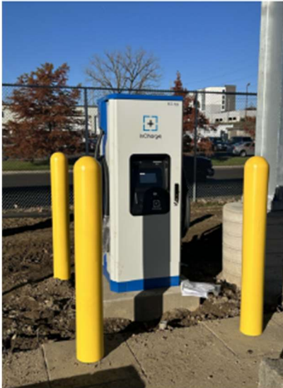
New EV Charging Station
