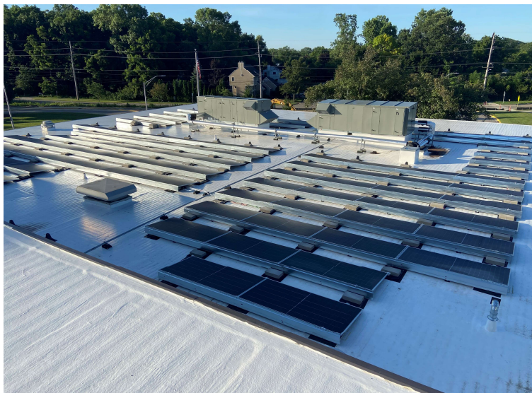
Clague Middle School Solar Array
