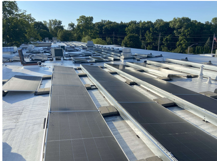
Clague Middle School Solar Array
