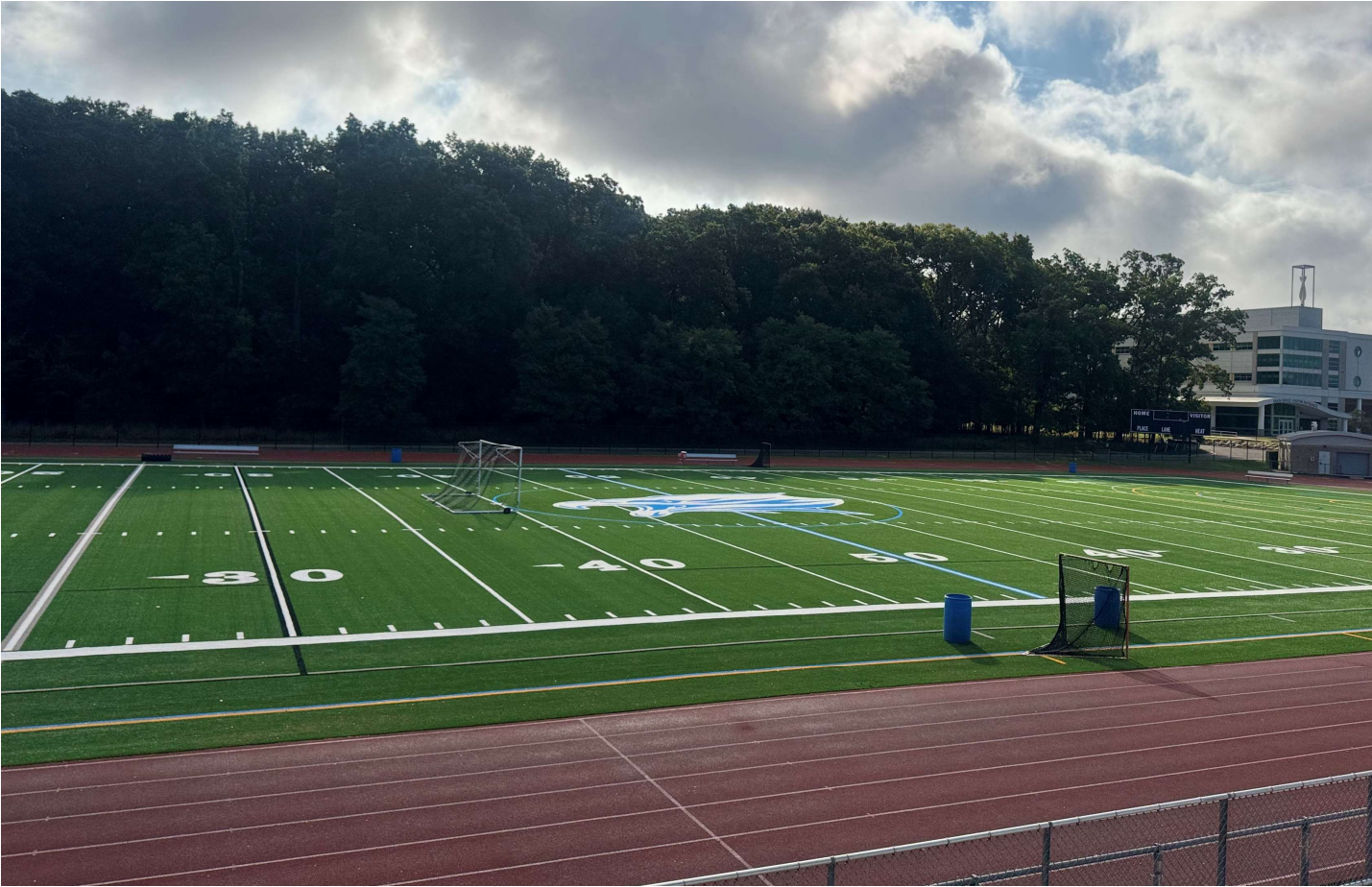
Skyline High School Synthetic Turf Replacement and Track Repair at Practice Field
