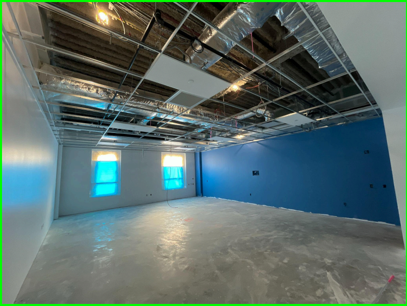
Photo 1: Interior fitout and finishes have started at the 2nd floor classroom space
