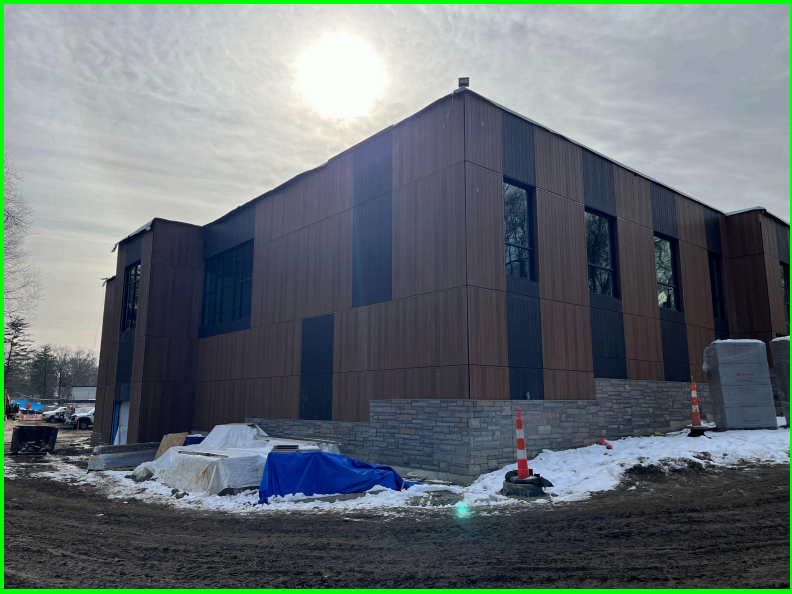
Photo 2: Exterior façade is being installed along the north east corner of the building
