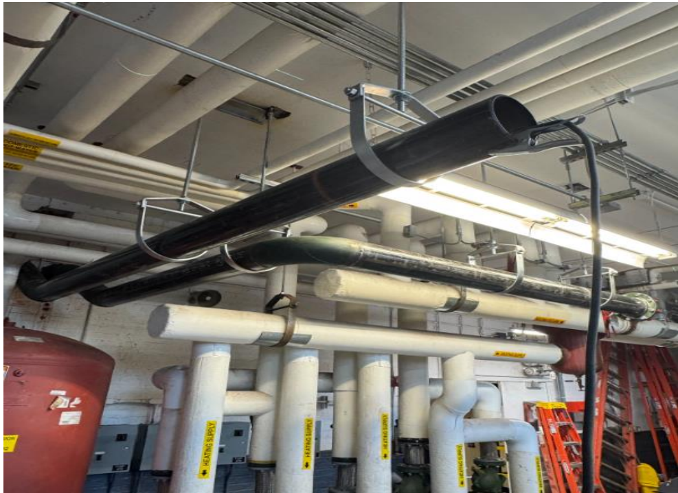
Hempstead IAQ – Prospect ES Chilled Water Piping
