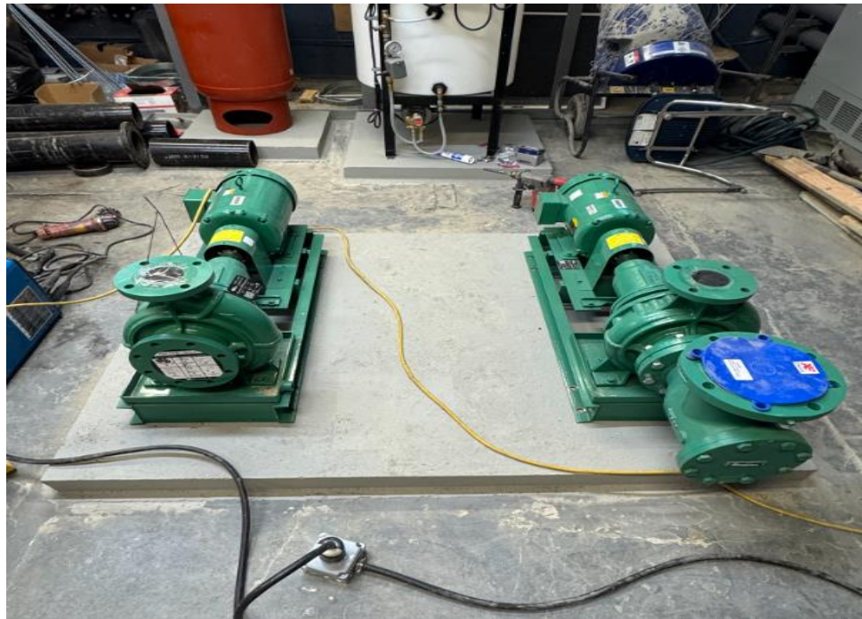
Hempstead IAQ – Chilled water system
