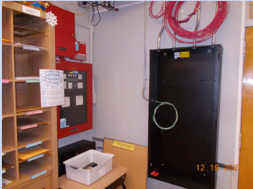
A new fire alarm main panel has been installed at Brunner Elementary School.
