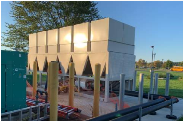
2017 CIP and 2020 CIP Air Conditioning – PEC, IEC, MS, HS
