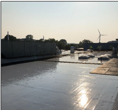
MCB White Roof
