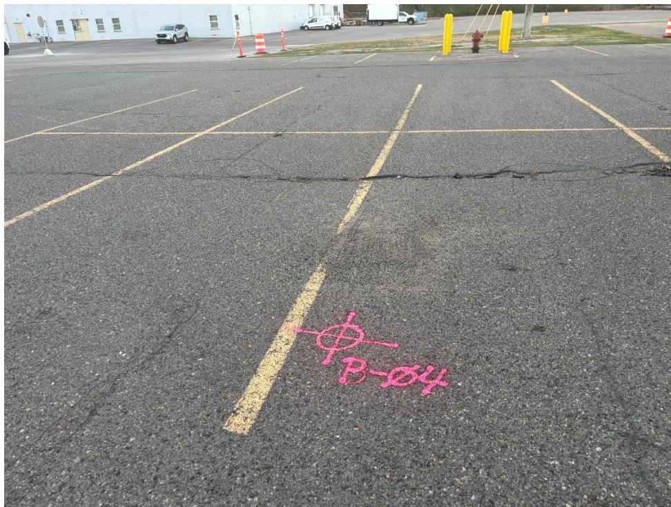
Photo No. 4 – Existing pavement conditions at B-04 looking south. Pavement distresses consisting of medium-severity transverse cracking and low-severity fatigue (alligator) and longitudinal cracking.
