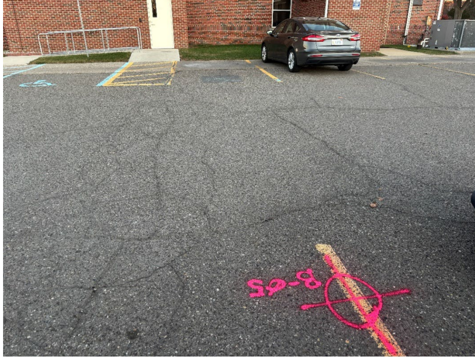
Photo No. 5 – Existing pavement conditions at boring B-05 looking east. Pavement distresses consisting of medium-severity fatigue (alligator) cracking and low-severity transverse and longitudinal cracking.
