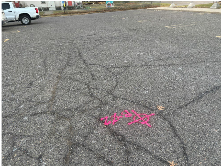
Photo No. 2 – Existing pavement conditions at boring B-02 looking south. Pavement distresses consisting of high-severity fatigue (alligator) and medium-severity transverse cracking.
