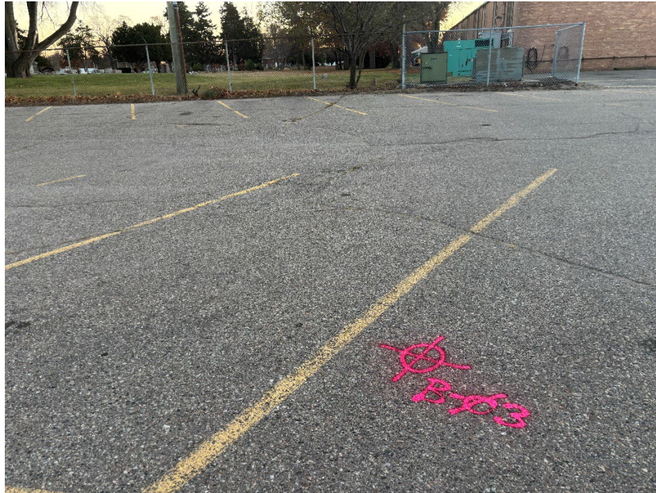
Photo No. 3 – Existing pavement conditions at boring B-03 looking south. Pavement distresses consisting of low-severity fatigue (alligator) and transverse cracking.
