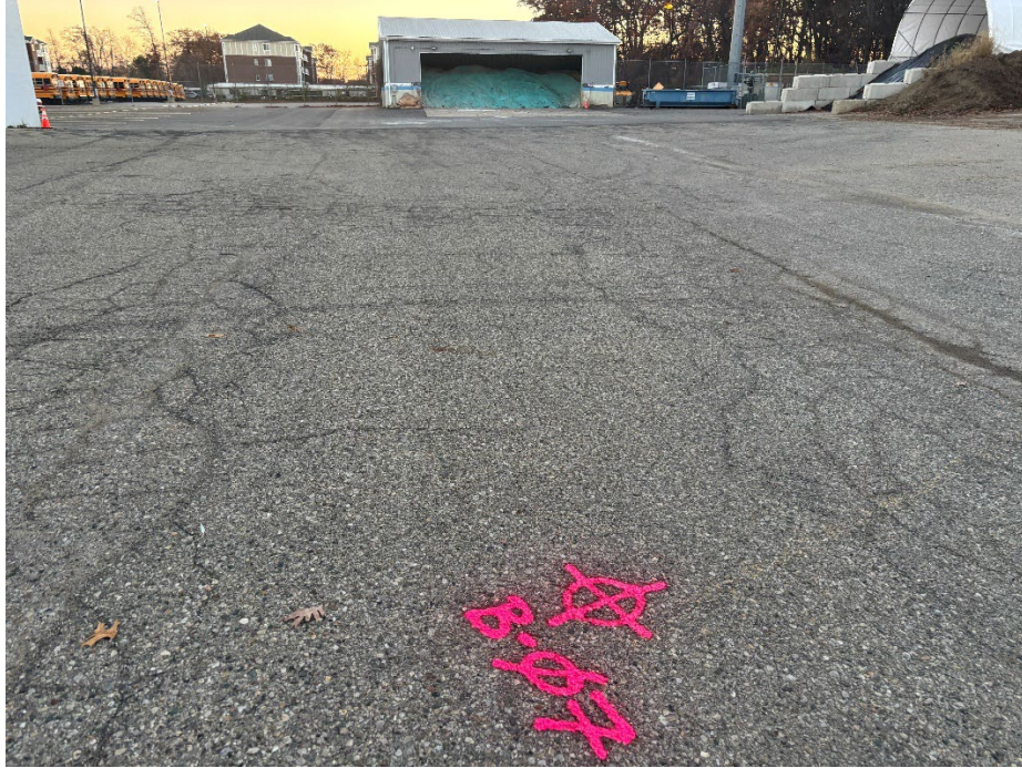
Photo No. 7 – Existing pavement conditions at boring B-07 looking south. Pavement distresses consisting of high-severity fatigue (alligator) and longitudinal cracking and medium-severity transverse cracking.
