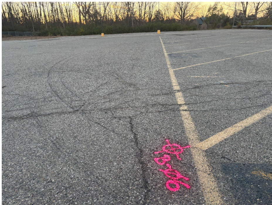
Photo No. 6 – Existing pavement conditions at boring B-06 looking west. Pavement distresses consisting of medium-severity fatigue (alligator) and low-severity longitudinal and transverse cracking.
