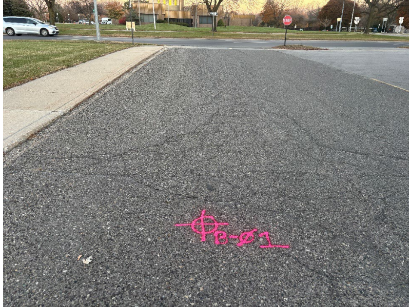
Photo No. 1 – Existing pavement conditions at B-01 looking east. Pavement distresses consisting of medium-severity fatigue (alligator) and low-severity longitudinal cracking.
