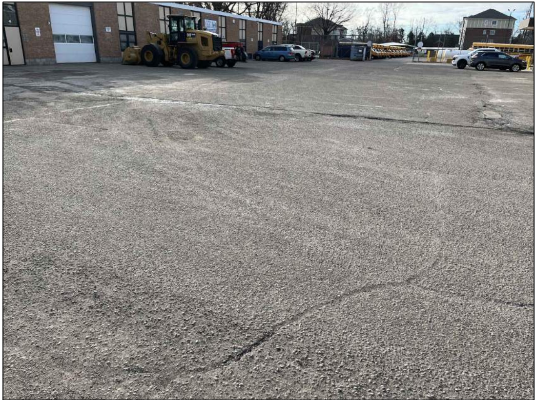
2 Block Cracking - Potholes NTS
