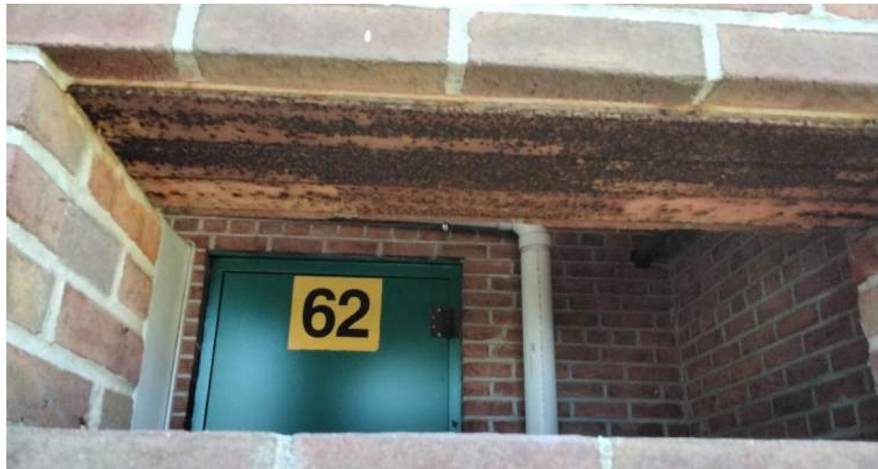
Typical corroded steel lintel.
