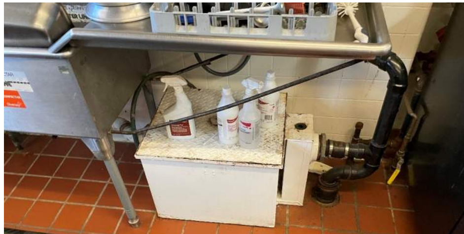
Undercounter grease waste interceptor.
