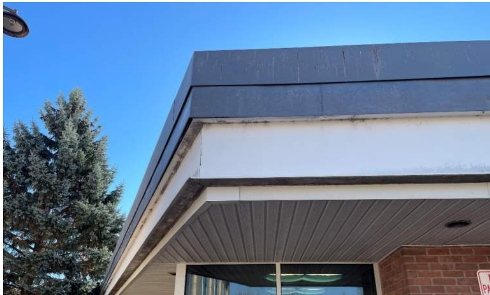
A typical roof eave at the perimeter of a low-slope roof system.
