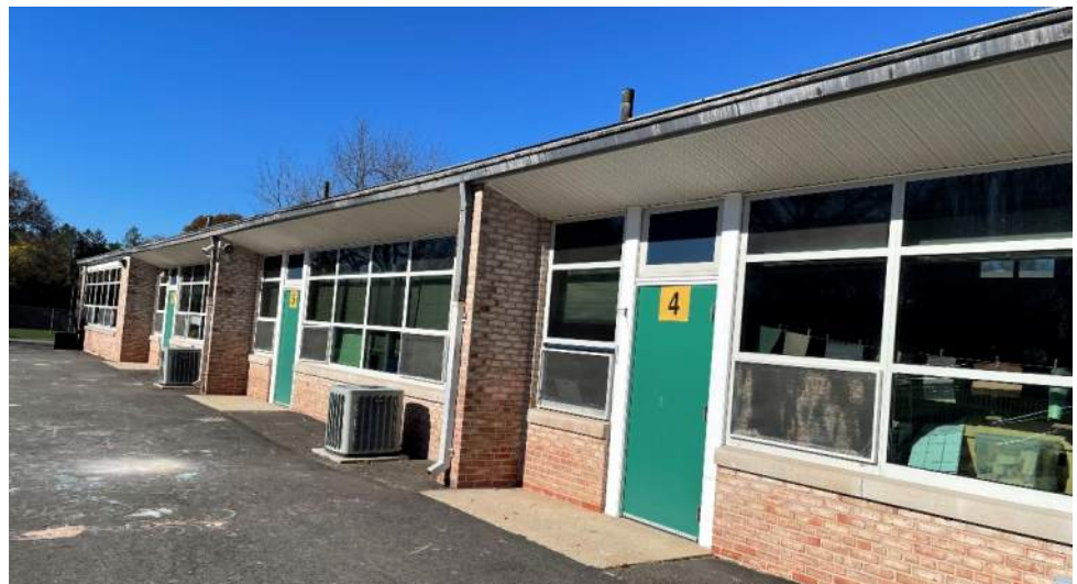
An alternative exit door configuration with flush landing transition to a paved exterior walk surface.
