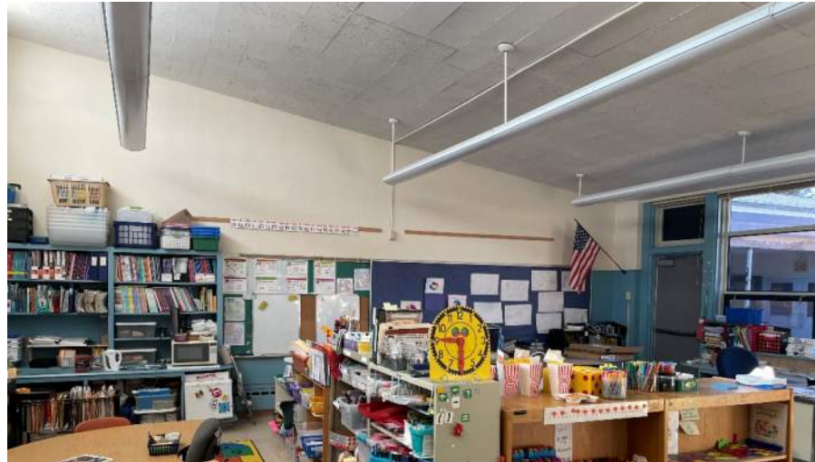
Direct applied 12-inch square acoustic ceiling tiles over a vaulted classroom ceiling.
