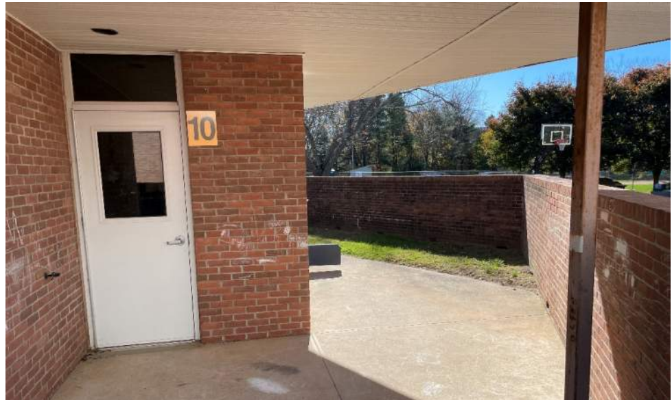
Exterior classroom doors fitted with level handles to facilitate re-entry.
