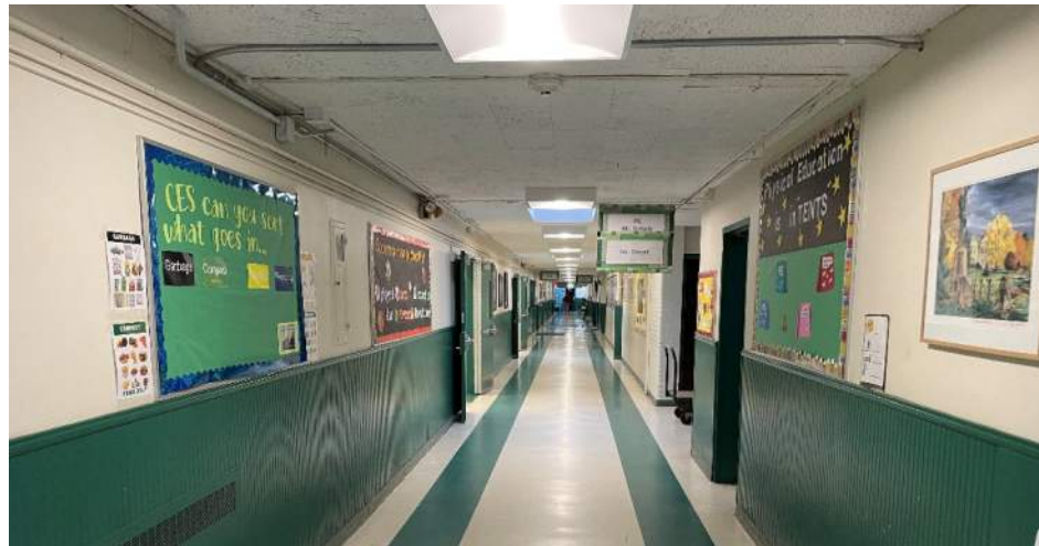
A central corridor within the original school with resilient floor finish and base. A painted wood wainscot has been installed in this portion of the school to protect the wall surfaces.
