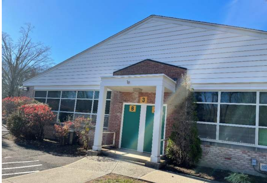
An example of a non-accessible building exit.
