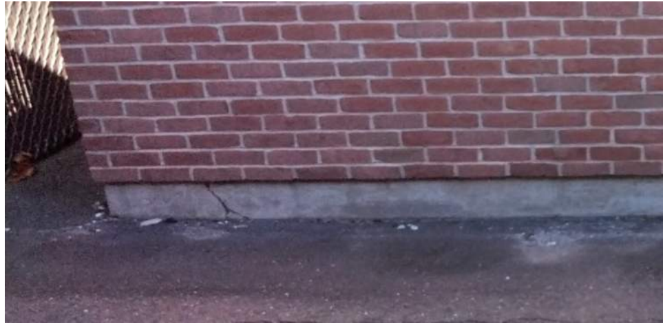
Cracked cast-in-place concrete foundation typical.
