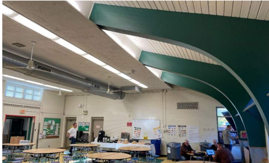
A view of the plank wood deck supported above laminated wood timbers at the east exterior wall of the cafeteria.
