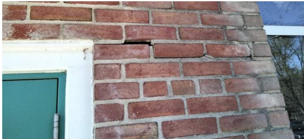
Cracked brick and failed mortar joints.
