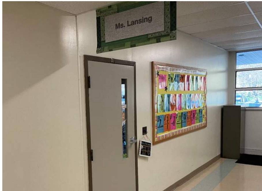
A typical suspended corridor ceiling demonstrating a slight deflection of the 2 feet by 4 feet ceiling panel.
