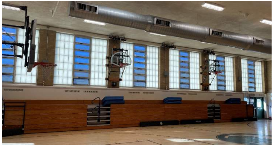
Existing retractable seating lacking provisions for accessible seating.
