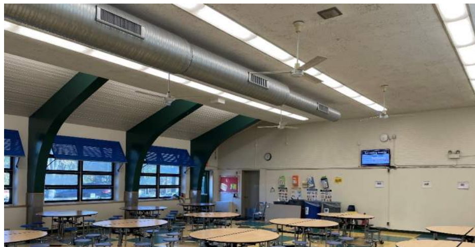
A view of the cafeteria with 12-inch square acoustic tiles in the foreground and exposed plank wood deck beyond.
