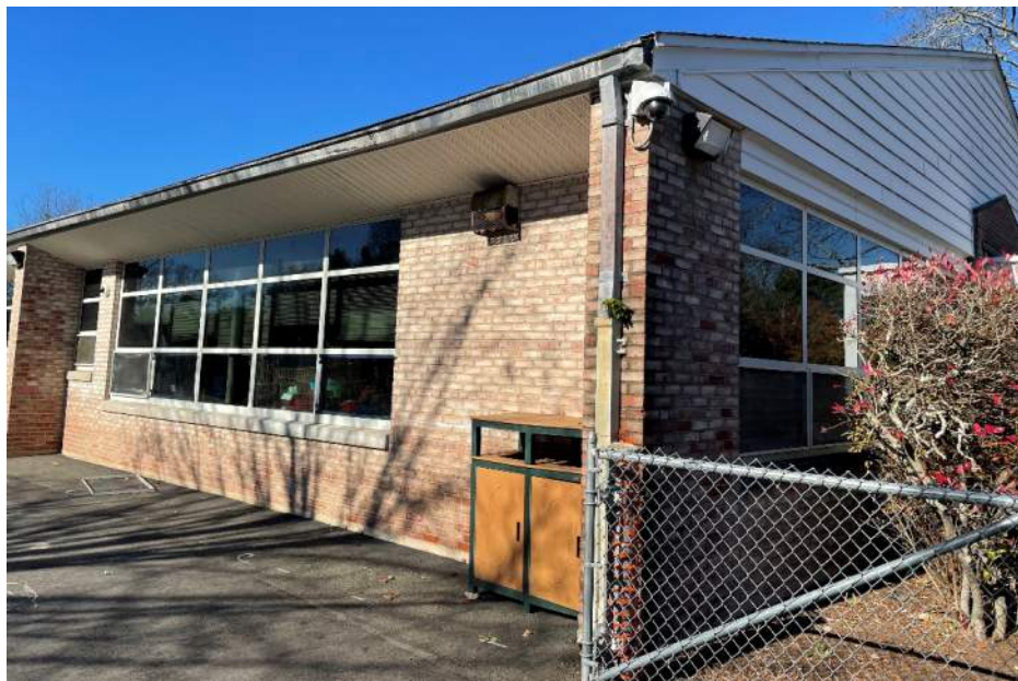
A gutter and leader connected to a below grade storm system.
