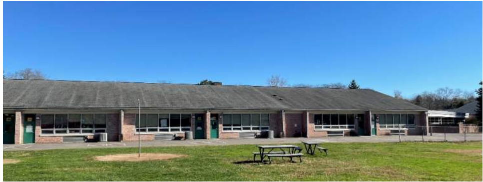
Staining of roof shingles and evidence of roof truss locations telegraphing through the roof finish.
