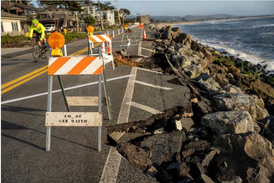
Storms in 2024 damaged Mirada Road in Miramar. County crews converted the street to one-way and added barriers. New funding would provide additional repairs to the road and riprap. Coastside News file photo
