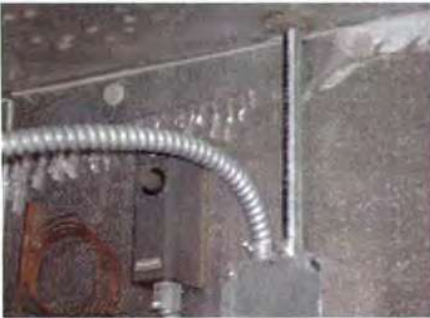
Operating Control Location
