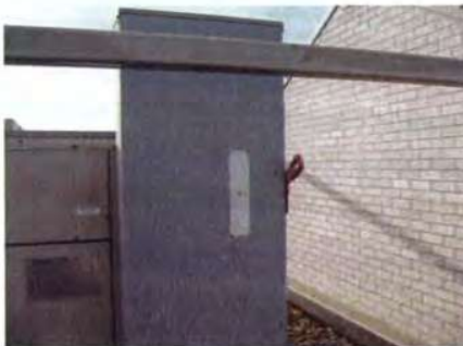
Isolating Device Location 1
