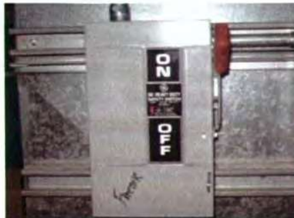
Isolating Device Location 1
