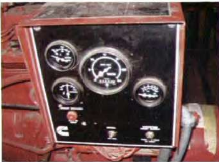
Operating Control Location
