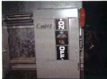
Isolating Device Location 1
