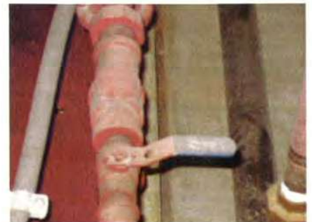
Isolating Device Location 2
