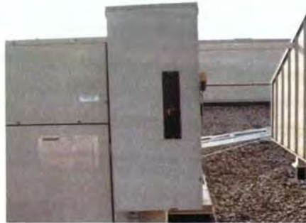
Isolating Device Location 1
