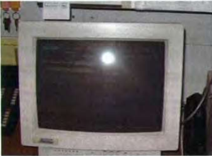
Operating Control Location
