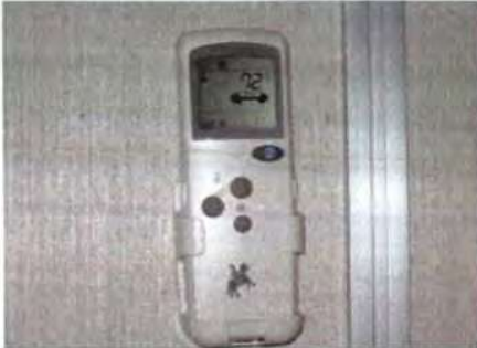
Operating Control Location
