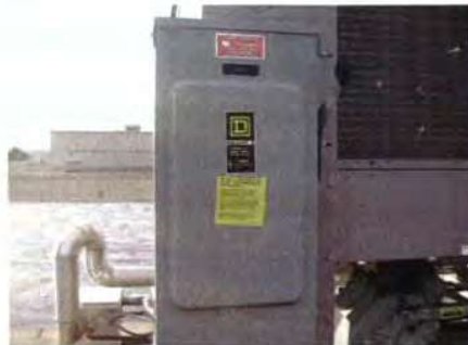
Isolating Device Location 1
