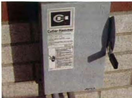
Isolating Device Location 1
