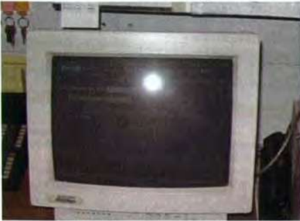
Operating Control Location
