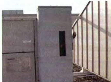
Isolating Device Location 1
