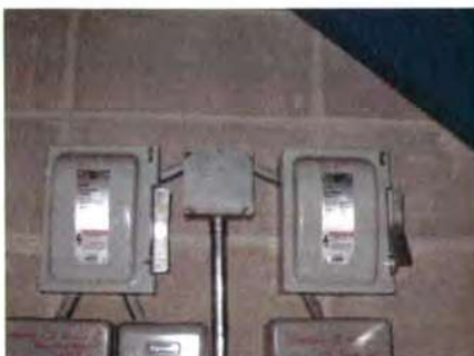
Isolating Device Location 1
