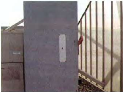
Isolating Device Location 1
