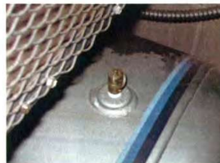
Isolating Device Location 2
