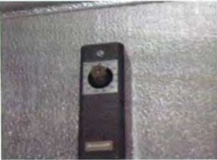
Operating Control Location
