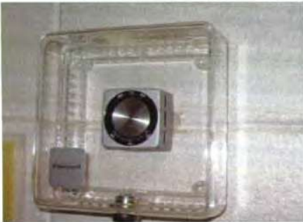
Operating Control Location
