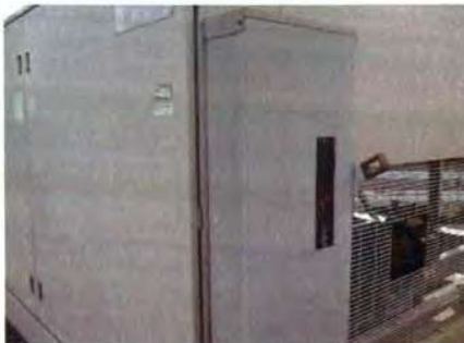
Isolating Device Location 1
