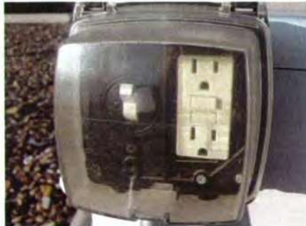
Isolating Device Location 1
