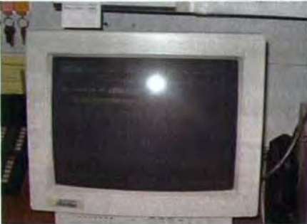
Operating Control Location
