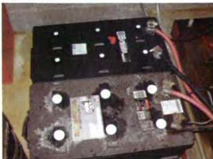
Isolating Device Location 1
