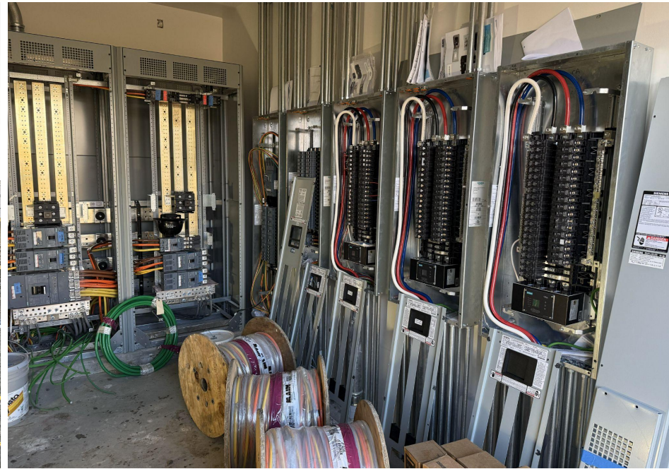
Bldg B Electrical Room
