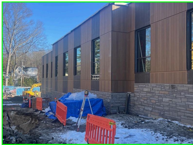
Photo 2: Installation of taping and prime painting of 2nd floor classrooms has begun
