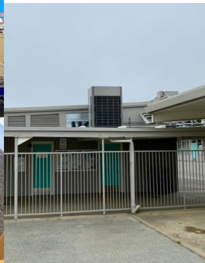
Roof mounted electric heat pump at Sunshine Gardens.
