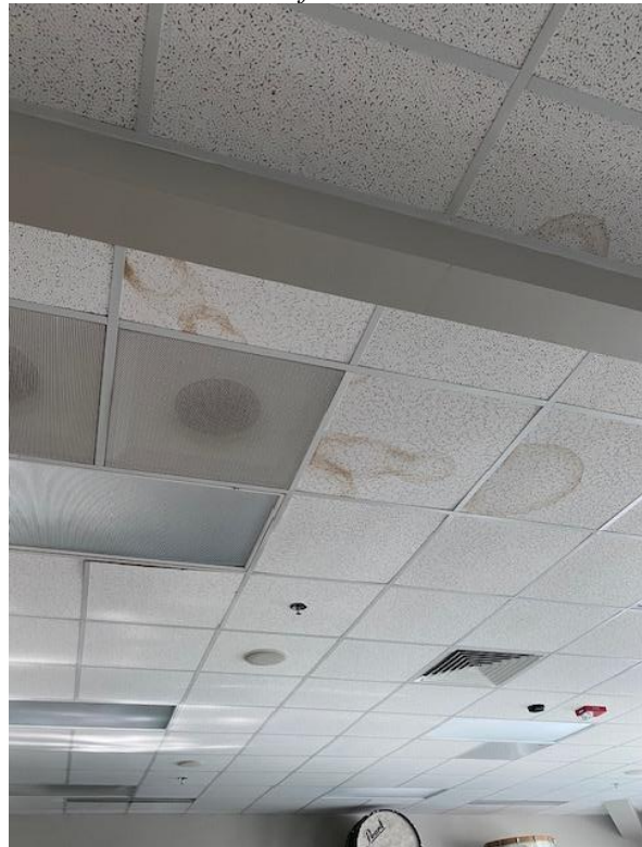
Classroom A106 – stained ceiling tiles
