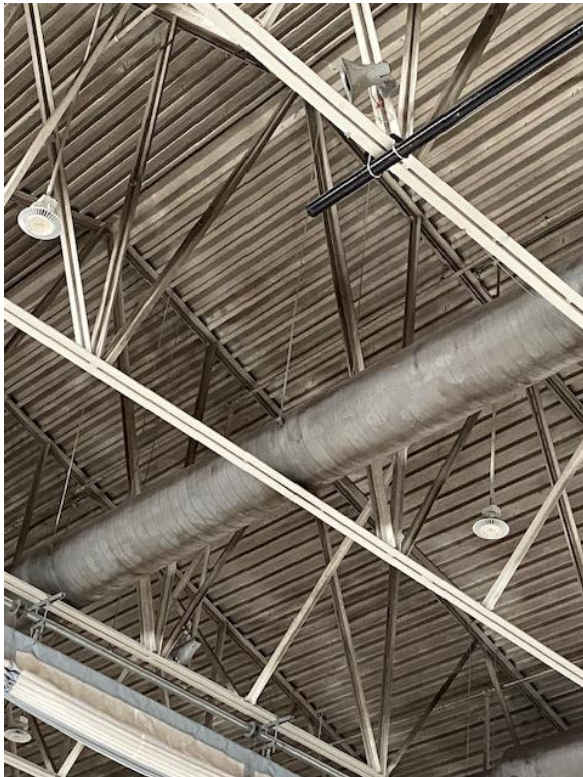
Gym – dark particulate on ceiling/roof structures
