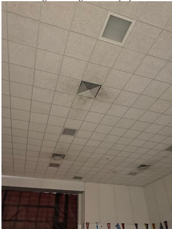
Gym – particulate on ceiling tile around supply diffusers
