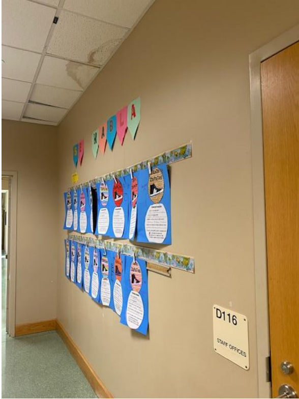
Staining on ceiling in Hallway by D116
