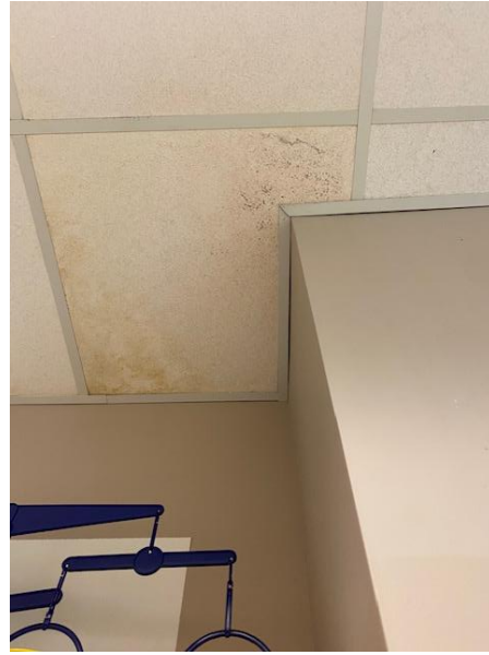
CR C316 Stained ceiling tile
