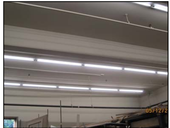
500 wing white fire piping at ceilings
