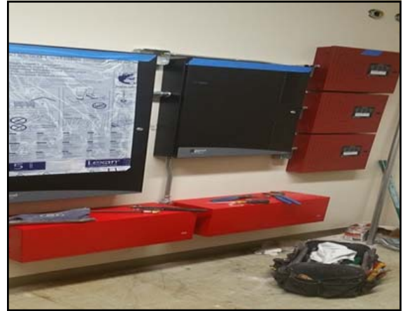
New main fire panels in admin area
