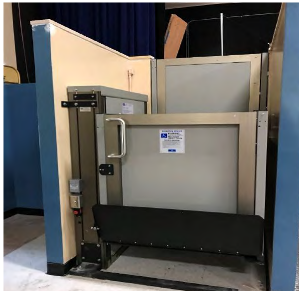
Fairmont ES - wheelchair lift to stage
