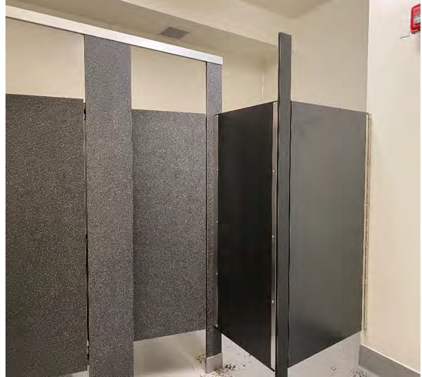
Student Restroom ADA Partition
