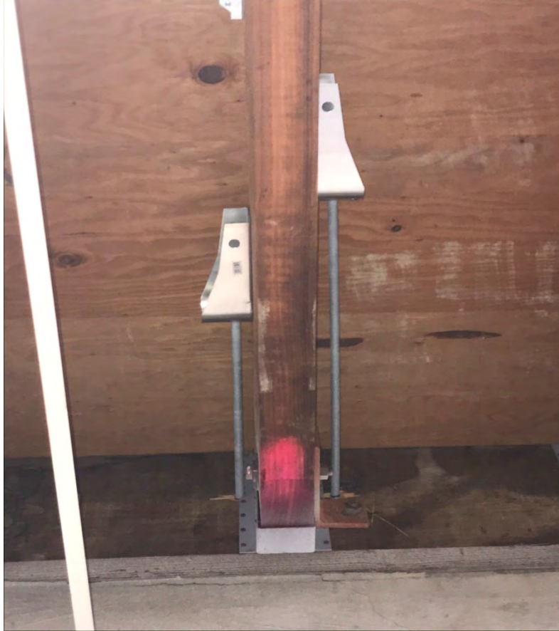
Seismic Braces, Science Bldg.
