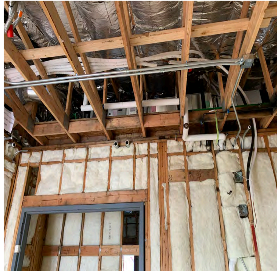
Kinder Room 111 HVAC Rough-In Above Ceiling
