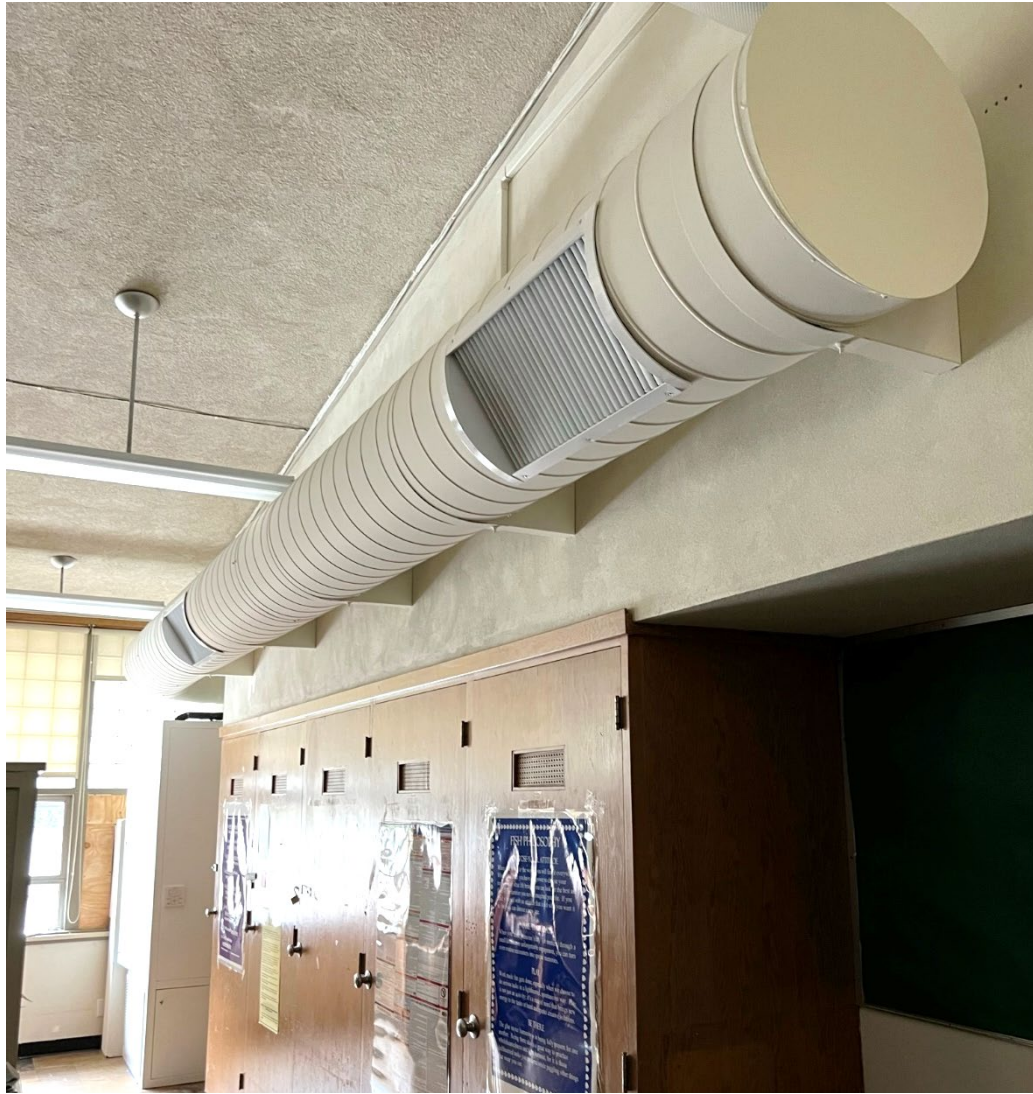
New Duct Work
