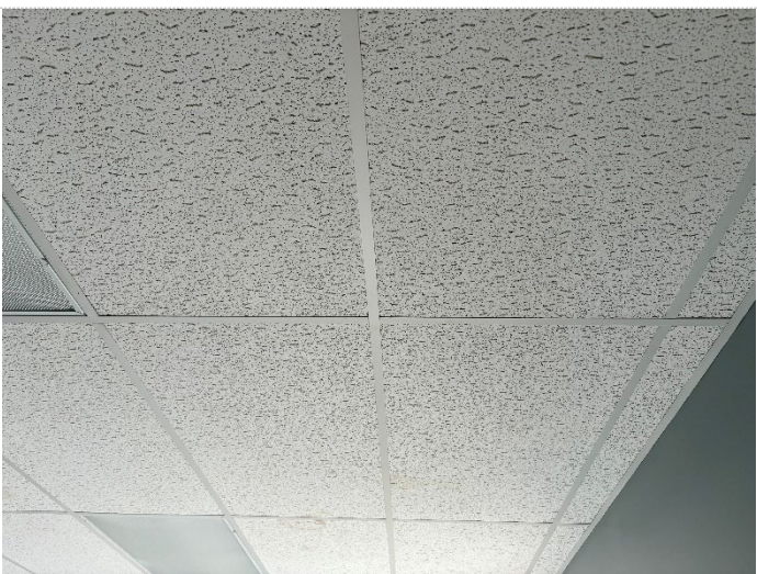
2x4 FCP – Pinhole Fissure
