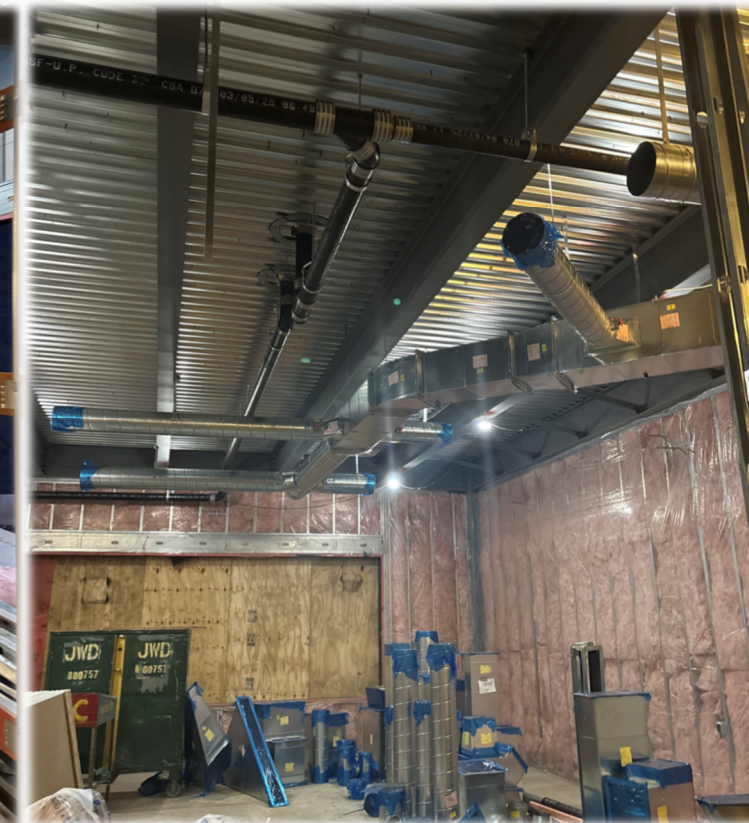
Windermere UPK Ductwork
