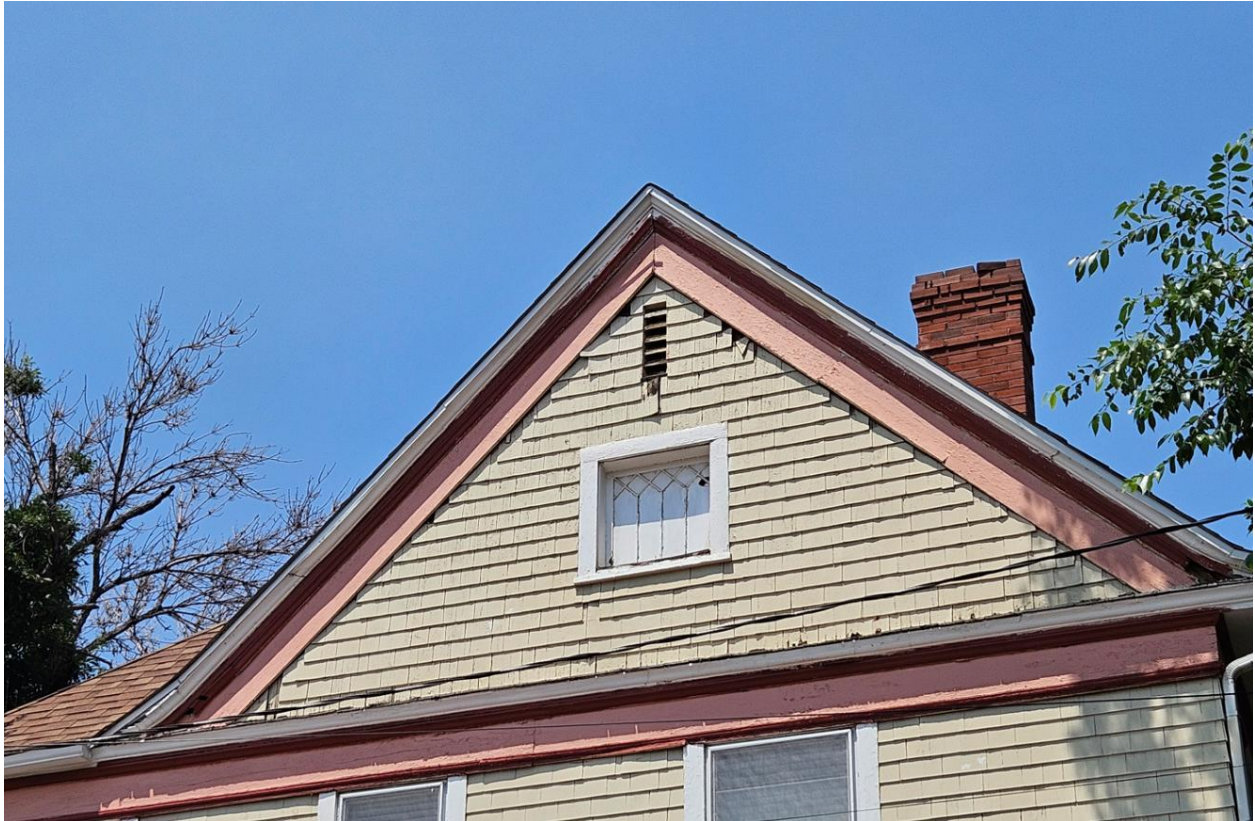
South Façade chimney and siding/trim condition detail
