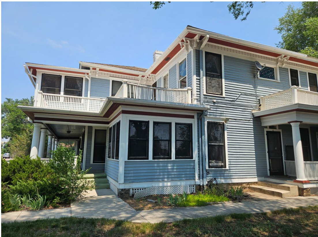
Partial South Façade showing cornice bracket detail and deteriorating railings
