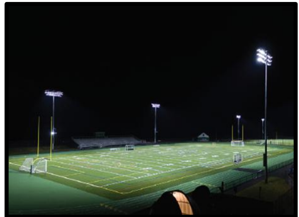
LED Field Lighting
