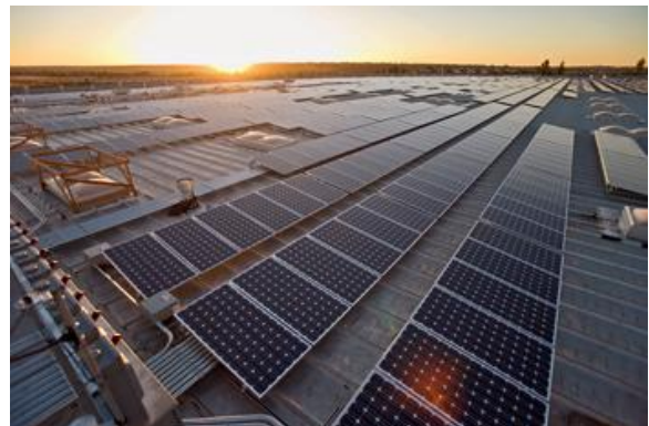
Photovoltaic (PV) solar array
