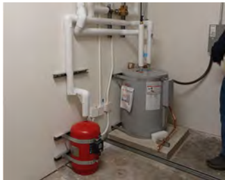
New Hot Water Heater
