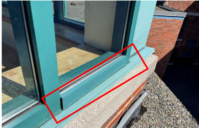
AE-30: Typical curtain wall snap cover that is not fully engaged to pressure plate at curtain wall located at East Elevation of West Wing
