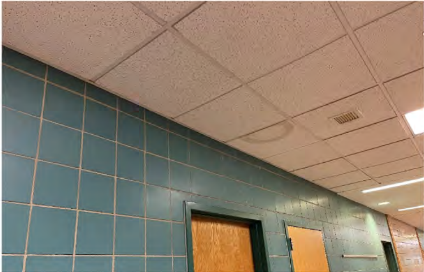
AE-56: Water damaged ceiling tile at leak location outside of Girl's Bathroom.
