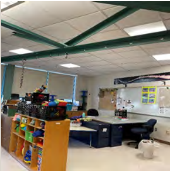
E-3: Classroom Lighting
