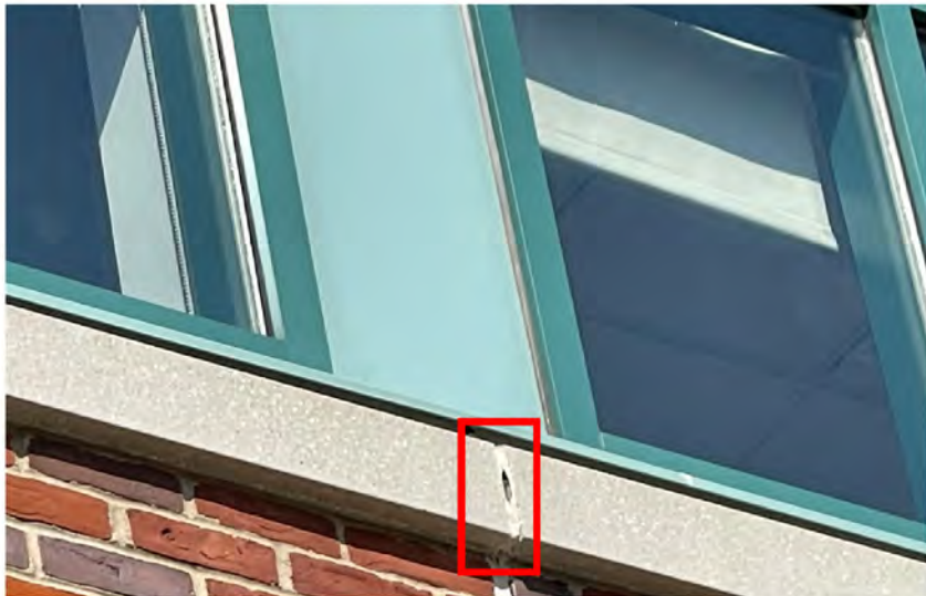
AE-15: Typical failed sealant at joint between precast sills
