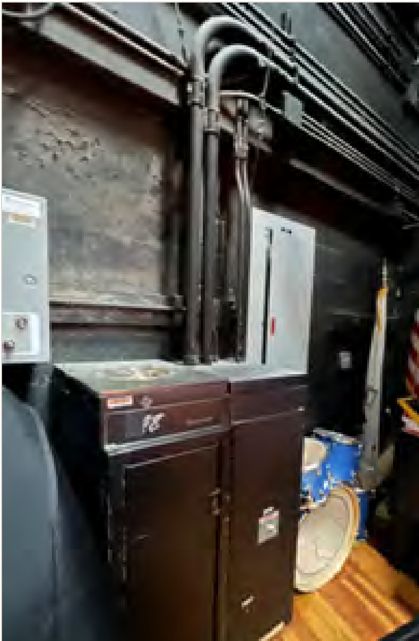
Existing Dimmer Rack
