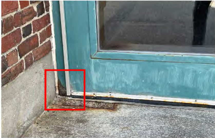
AE-37: Typical rusting at exterior base of metal framed door, typical in most locations.
