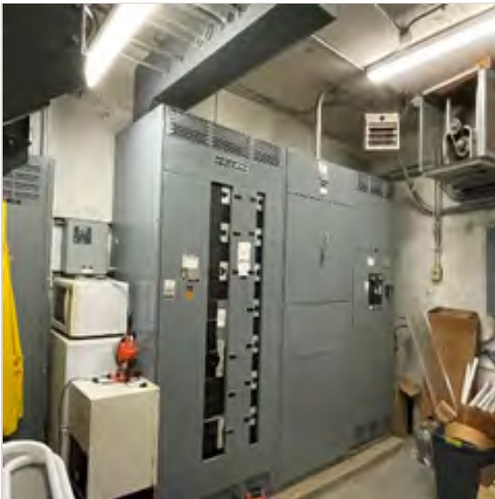
E-1: Main Electrical Service (Entrance)
