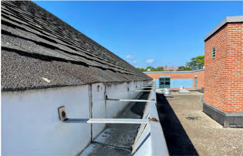
AE-54: Representative aluminum gutter along base of shingled roof.
