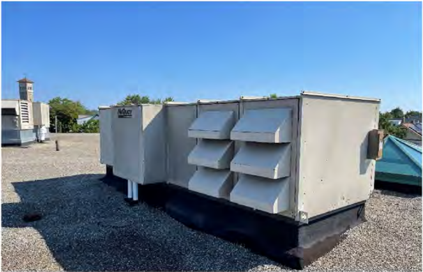
AE-50: Typical MEP unit on curb.
