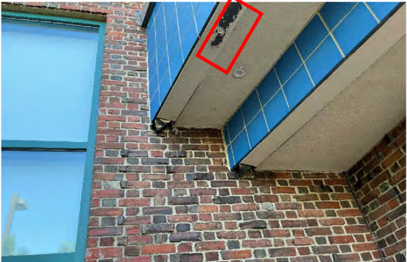
AE-20: Typical peeling paint at relieving angle
