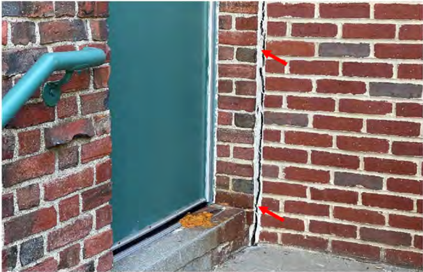
AE-22: Control joint at intersection of older building and addition, failed sealant at this joint.
