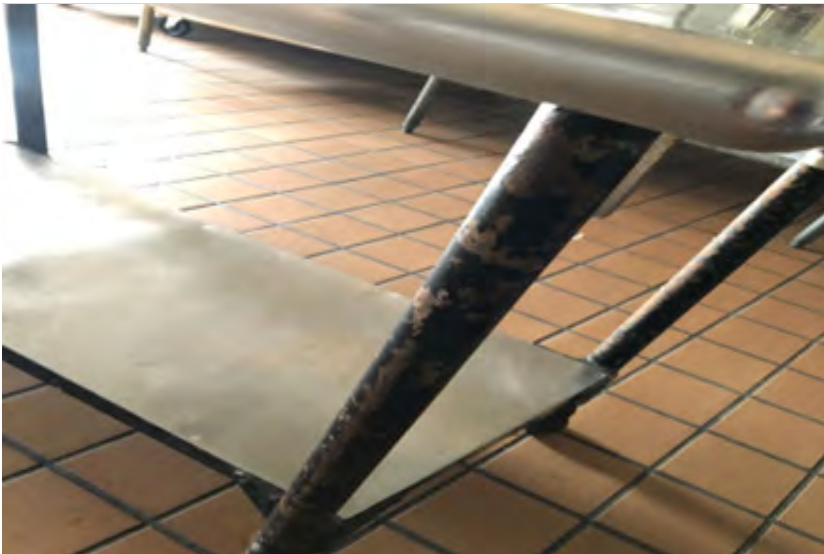
FS-1: Galvanized legs on work tables is a dated construction method. The galvanized steel chips and rusts and requires frequent painting to maintain. Stainless steel tables should be replaced with all stainless steel construction manufactured to meet NSF standards.
