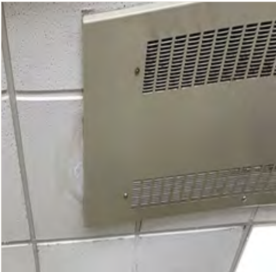
M-5: Water Damage by FCU
