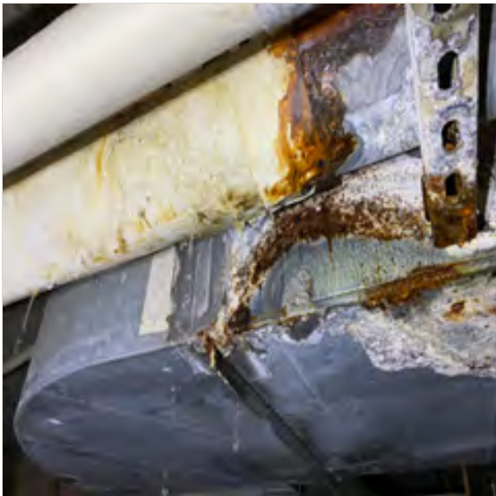
PL-1: Domestic Main Failure in Crawl Space
