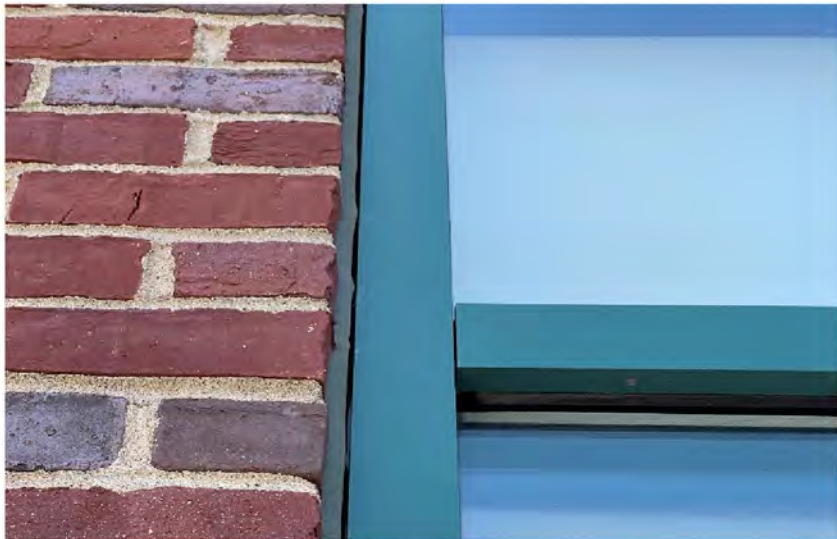
AE-39: Typical failed sealant at perimeter of fenestration
