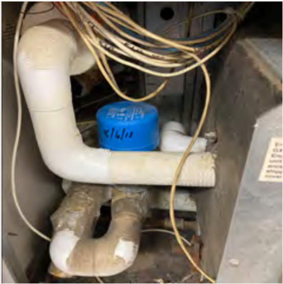
M-2: Unit Ventilator Interior Conditions
