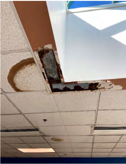
Photo ST-6: Water damage at cafeteria skylight
