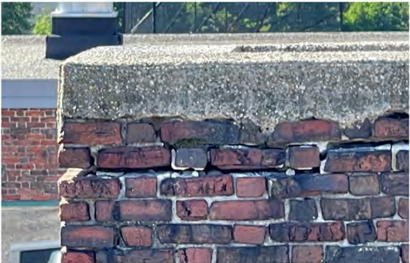
AE-12: Deteriorated mortar, displaced brick at chimney
