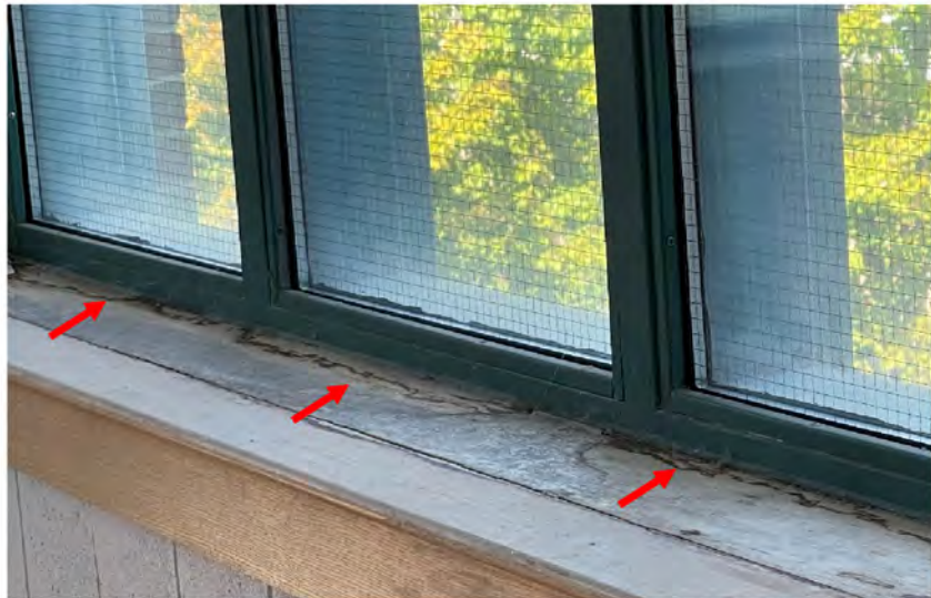
AE-36: Interior of Southwest stairwell where staining evident of water leakage was observed around hollow metal window assemblies.
