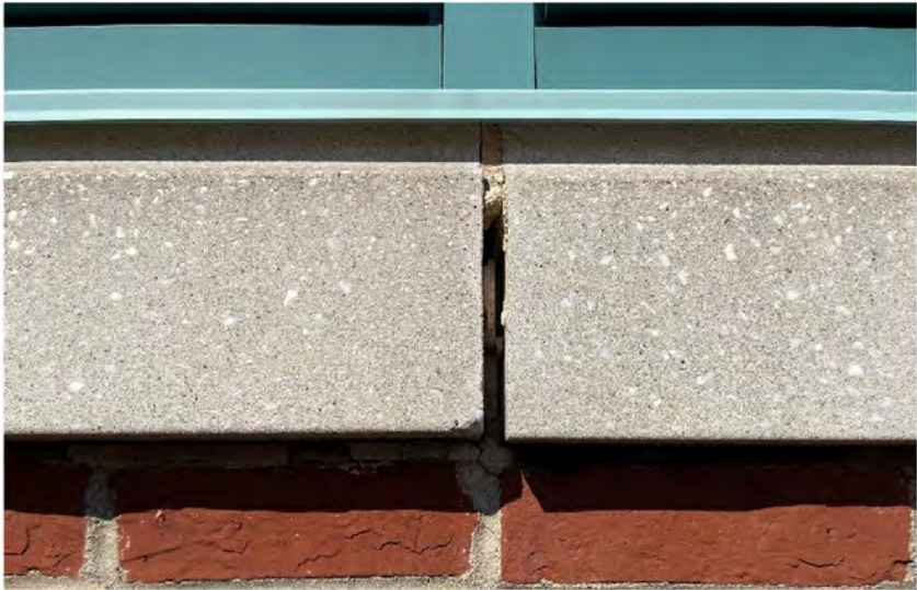
AE-14: Isolated cracked, spalled mortar between precast sills
