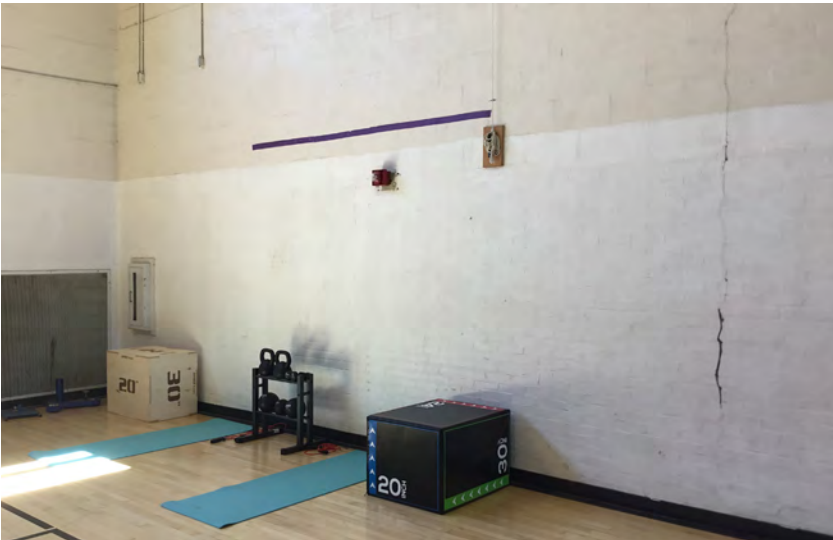
Crack in walls
