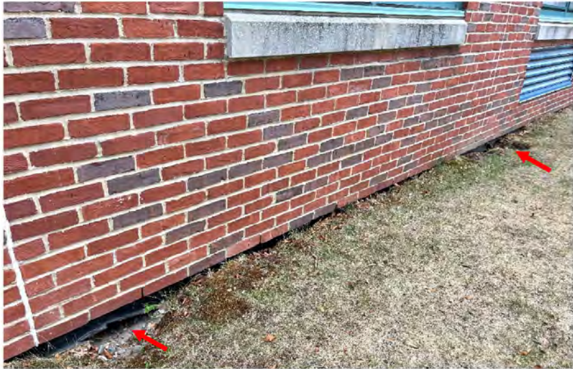
AE-21: Base of North Elevation where there is a cavity below the façade / building and rodents reportedly burrow and nest.
