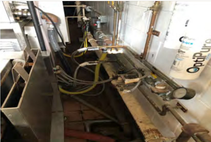
FS-4: Exposed utilities along the cook line building wall present cleanability issues and potential violations of the health code if not properly cleaned. Utilities should be provided within a furred-out wall in these circumstances for proper cleanability.
