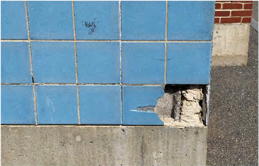
AE-18: Damaged glazed block at base of facade on Southeast corner
