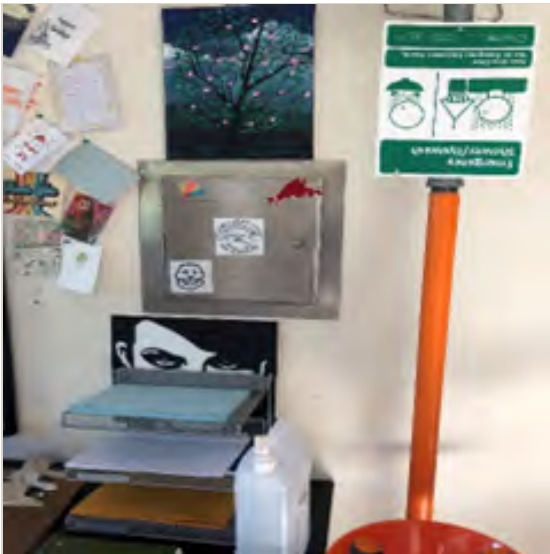
PL-4: Gas Valve Cabinet
