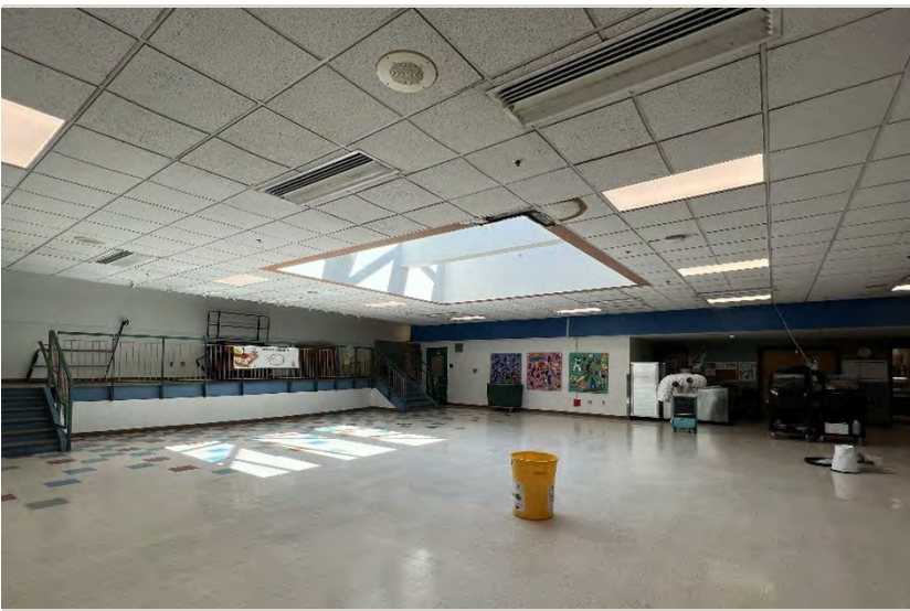
Cafeteria (leaks at skylight)
