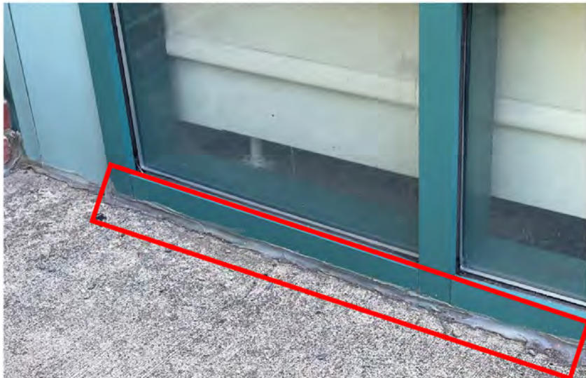
AE-31: Typical curtain wall where sealant has been applied over base of snap covers where drainage from curtain wall occurs
