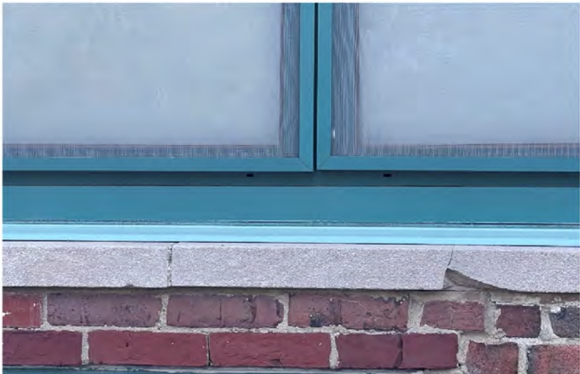
AE-16: Representative cracked and spalled limestone sill at older portion of building
