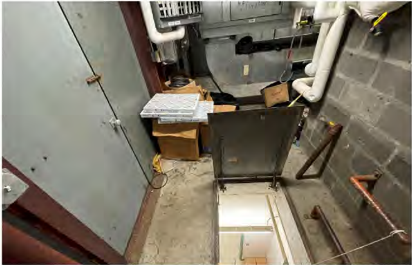
AE-41: Roof access within penthouse. Penthouse door is very close to hole in floor from access hatch. Very awkward and not safe.
