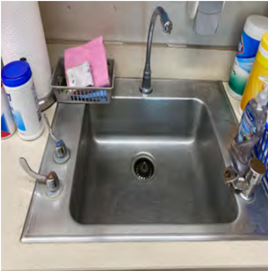
PL-3: Classroom sink
