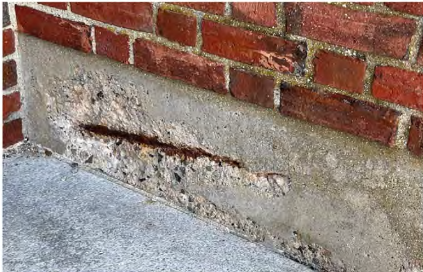
AE-23: Isolated exposed rebar at foundation of older portion of building near building entrance.
