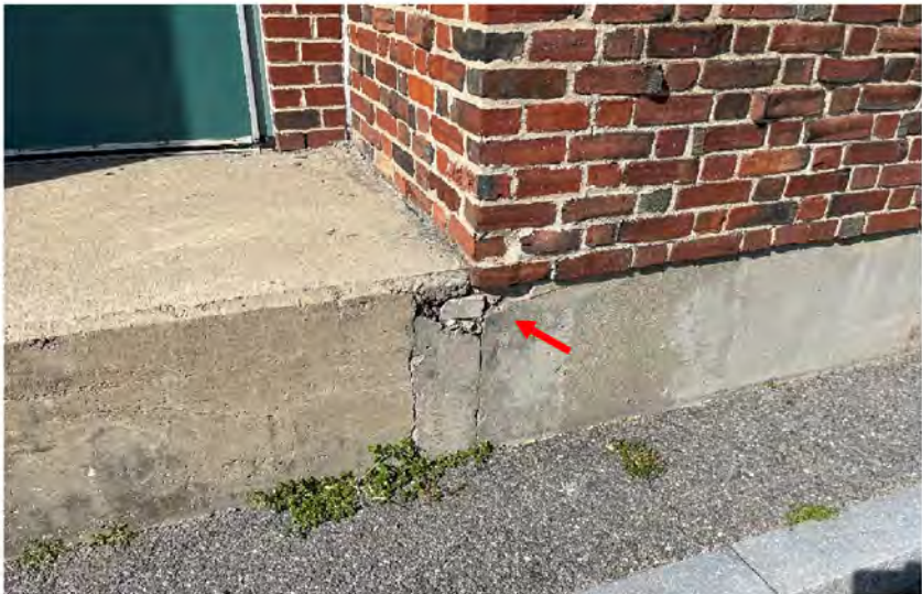
AE-24: Representative cracked and spalled concrete.
