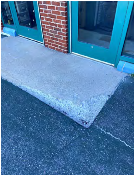
Photo ST-5: Deterioration of concrete approach slab
