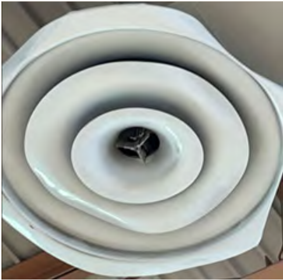
M-6: Gymnasium Diffuser Condition
