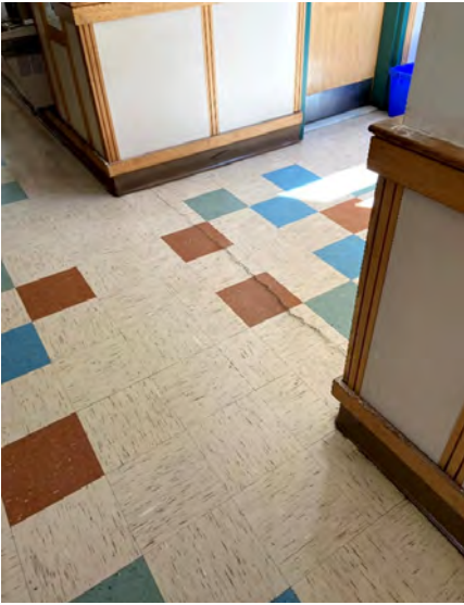
Photo ST-7: Crack at floor finish in 1995 addition corridor
