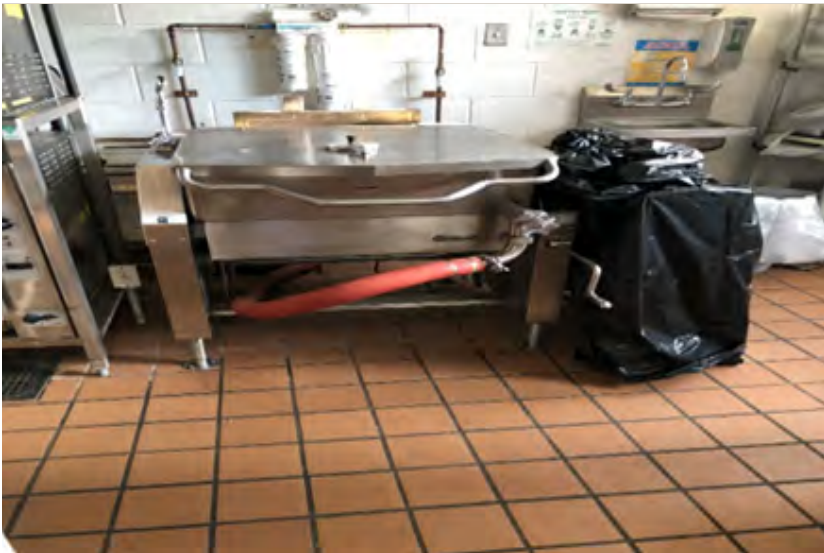
FS-3: Braising pans in efficient designs are provided with floor troughs with non-slip grating for proper cleaning and containment of the units' operation. The tangent draw-off valve is currently piped to a floor sink which presents several issues to the buildings plumbing system. The purpose of the tangent draw-off valve is to be able to prevent grease and other unwanted product from entering to entering the building drainage system.
