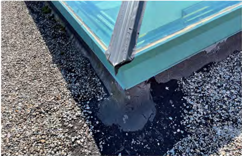
AE-49: Typical metal framed skylight with evidence of interior leakage. Note black tape applied over framing, sealants applied around glass.
