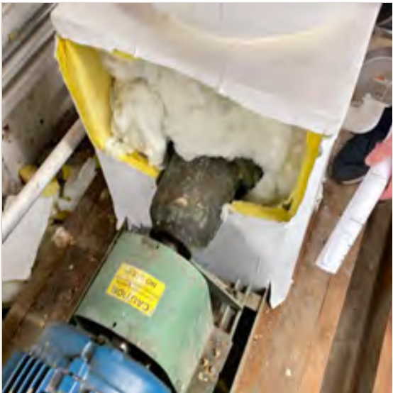
M-1: Exposed Pump Condition
