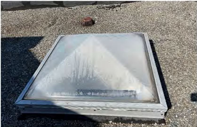
AE-48: Typical unit skylight where thermal seal has failed, allowing condensation between panes of skylight
