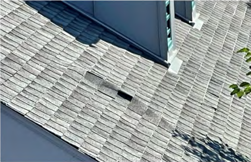
AE-53: Typical asphalt shingles buckling, noted in a few locations. Source of buckling is unknown.
