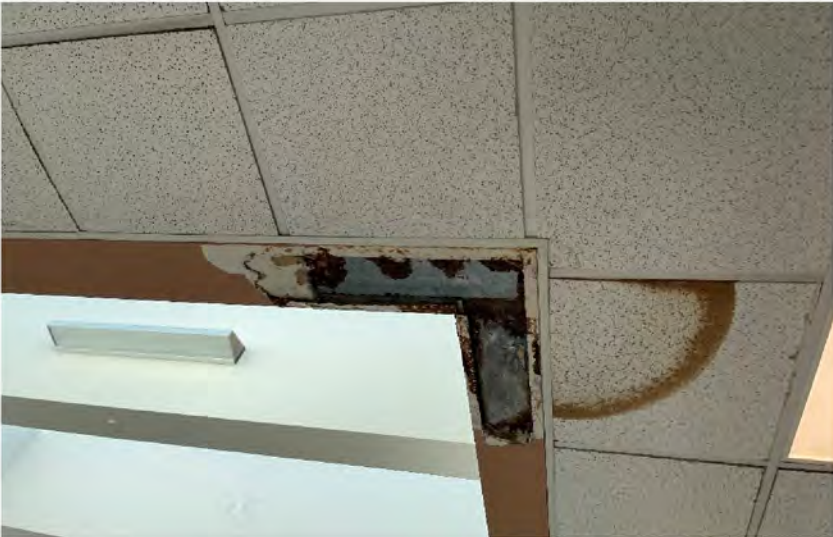
AE-55: Interior damage at leak below metal framed skylight in Cafeteria.
