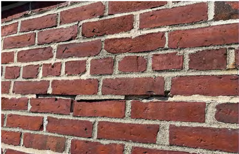
AE-11: Typical isolated deteriorated mortar at steel lintel
