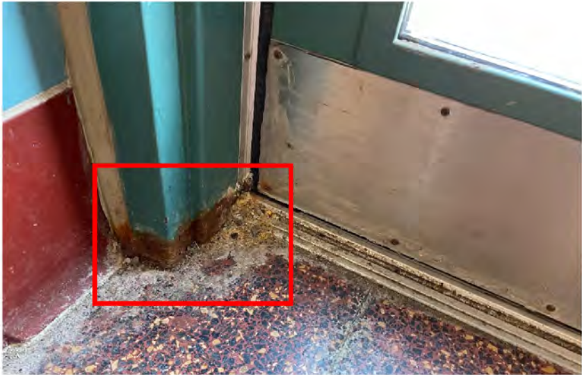
AE-38: Typical rusting at interior base of metal framed door, typical in most locations.
