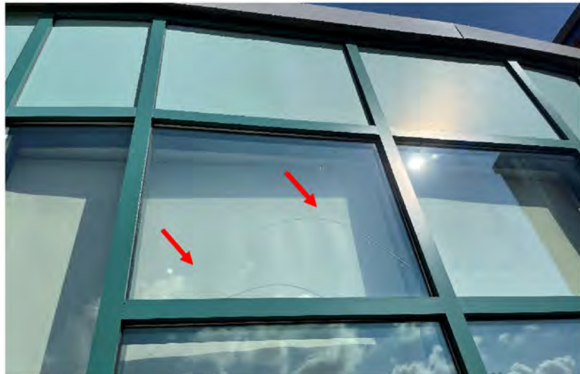
AE-32: Cracked glass within curtain wall on West Elevation at curved facade
