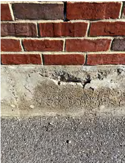
Photo ST-1: Concrete spalling at perimeter foundation wall
