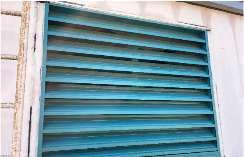
AE-28: Typical louver installed in mechanical penthouse, note multiple perimeter sealant colors around louver due to repairs made over time.
