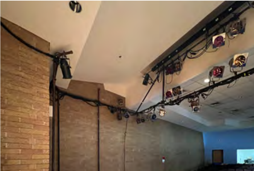
Additional Lighting Pipe at Front of House; Temporary Cable at Left
