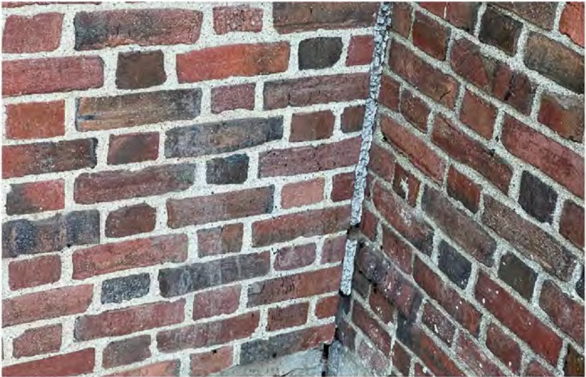
AE-10: Representative brick masonry at older portion of building. Note some failed control joint sealants.
