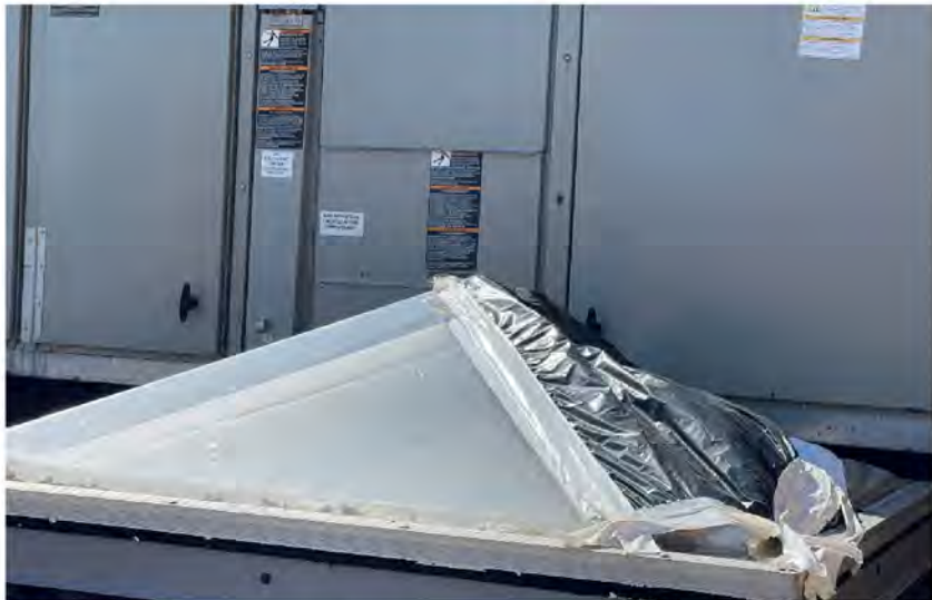
AE-47: Typical damaged unit skylight, covered with black plastic and duct tape
