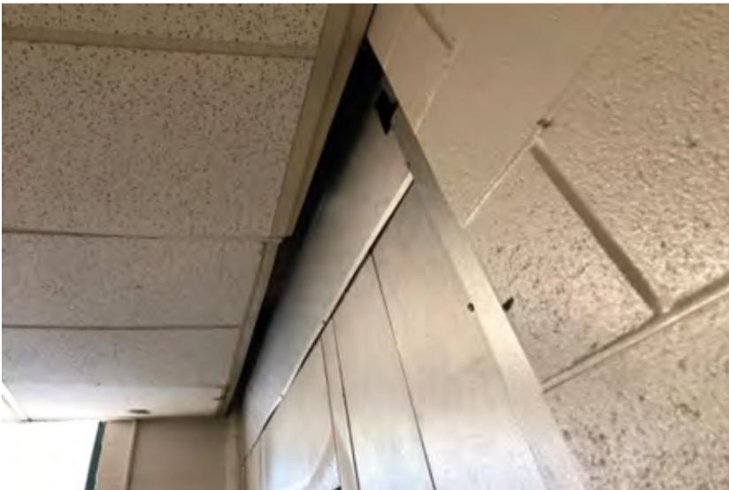
FS-2: Gaps in kitchens are not acceptable by health code. The ceiling track and/or the stainless closure should be provided to prevent large gaps within commercial kitchens per health code. Large gaps within kitchen spaces allow vermin and or insects entry points to food zones.
