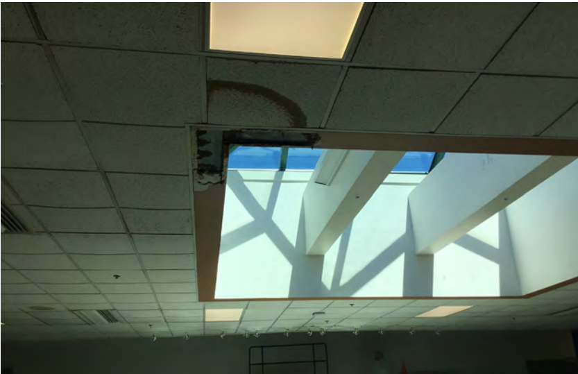
Water damage at skylight
