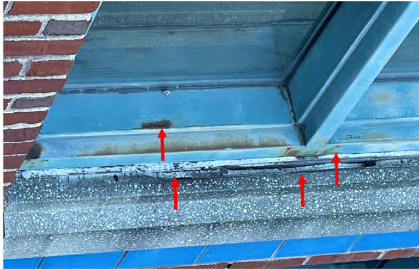
AE-34: Typical failed sealant joint between precast sill and hollow metal window assembly at Southwest Stairwell. Note rusting of metal frame.
