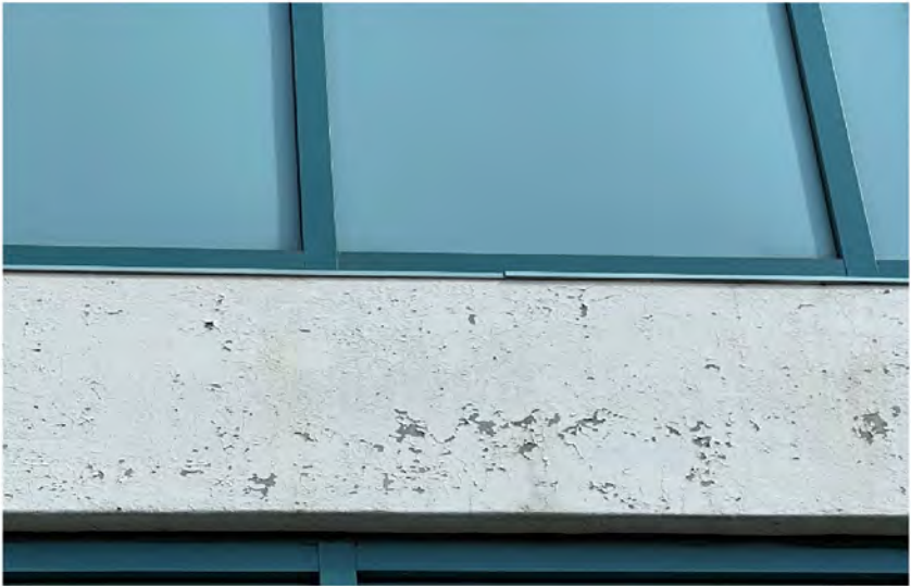
AE-26: Typical peeling paint at concrete facade
