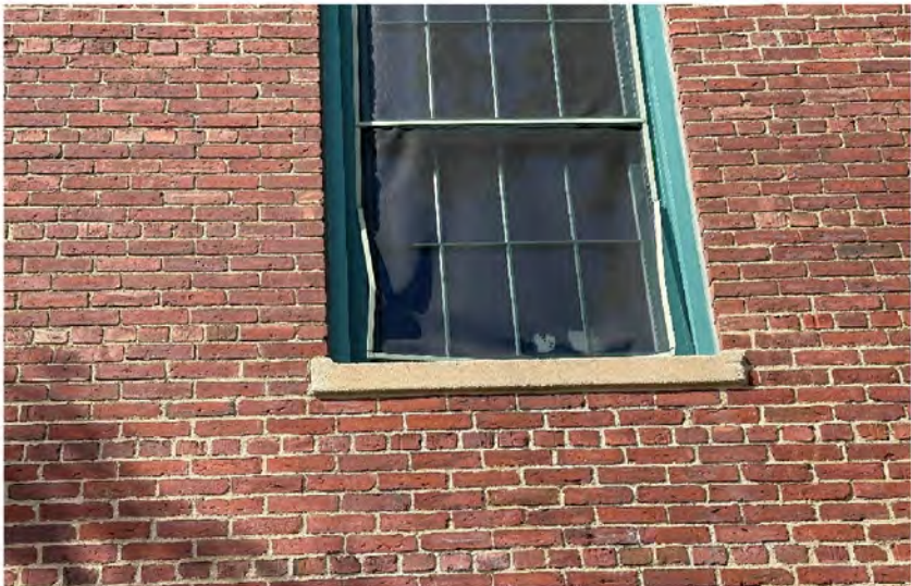
AE-40: Representative damaged insect screen
