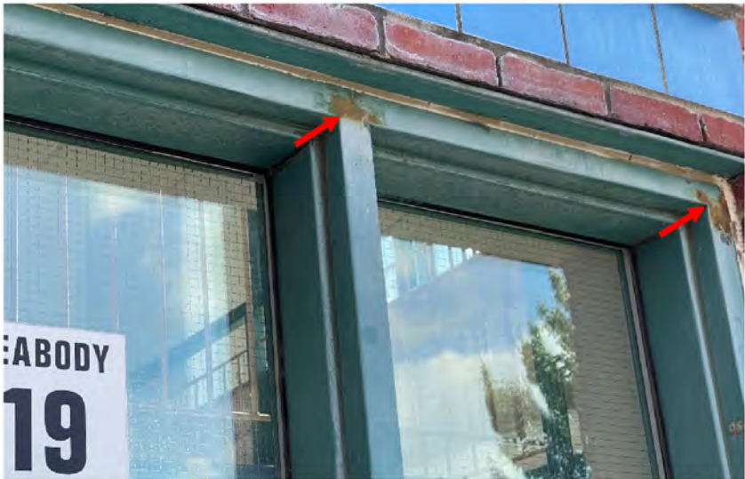
AE-35: Typical rusting of hollow metal window assemblies at Southwest Stairwell above Door 19.
