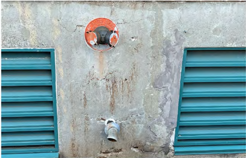
AE-25: Representative cracking and isolated spalling, exposed rebar at foundation wall of older portion of building, noted along East Elevation.
