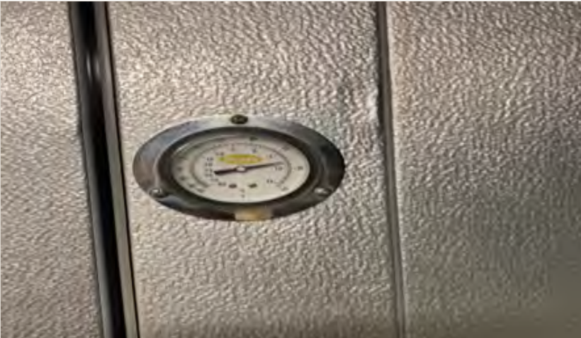
FS-2: The walk-in cooler shows clear signs of refrigeration issues as it’s currently holding at approximately 50°. This temperature is not within a safe range and the system requires service and repairs in the immediate future.
