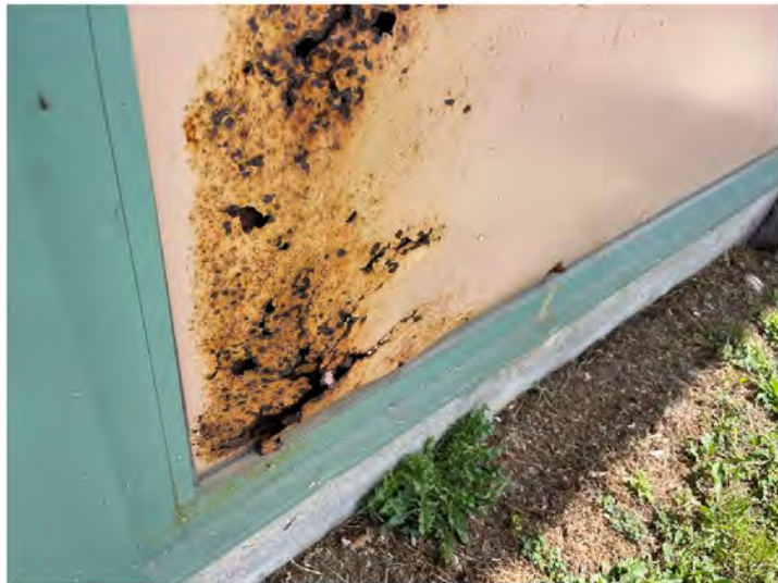
AE-31: Typical rusting of spandrel panel within storefront assembly
