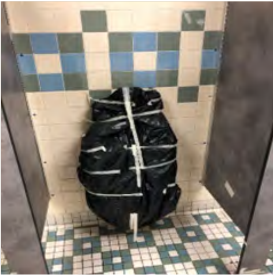
PL-4: Broken Urinal
