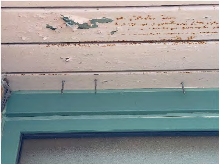
AE-53: Typical rusting and peeling paint at exposed underside of metal roof decking, typical in most locations. Not exposed fasteners from roof securement above.
