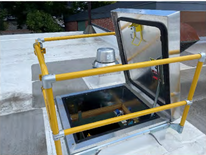
AE-68: Roof access hatch
