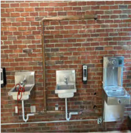
PL-2: Cafeteria Handwash Sinks Missing Hot Water
