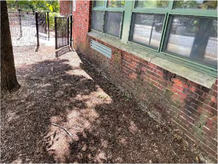
AE-17: Section of East Elevation at D Wing where roof drains to grade, splashing onto masonry façade. Some deteriorated mortar and vegetation growth on façade.
