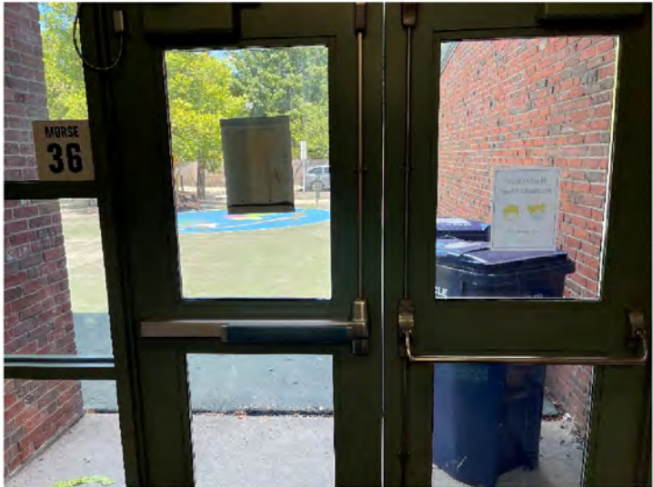
E-49: Interior of door 36 where no weatherstripping was observed at interior between door panels.
