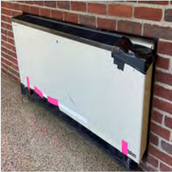
M-2: Cabinet Unit Heater Conditions
