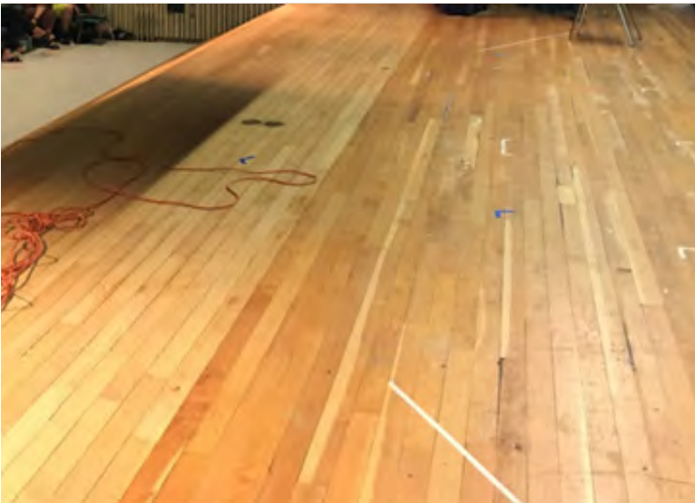
Stage Floor in Poor Condition
