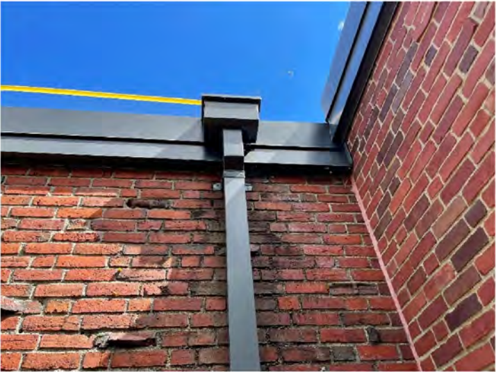
AE-19: Typical staining and isolated mortar deterioration around gutter at West Elevation near Cafeteria
