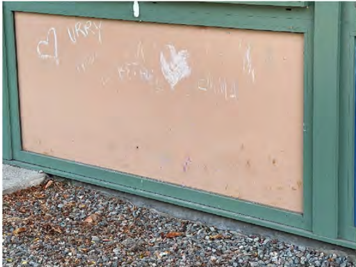
AE-33: Typical light surface rusting on typical spandrel panel within storefront assembly
