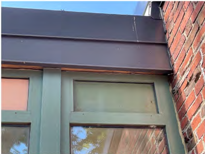
AE-36: Representative rusting of spandrel panel installed within storefront assembly
