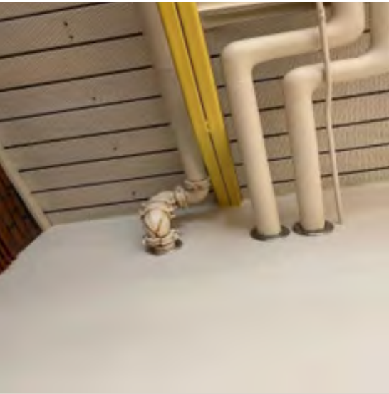
FP-2: Leaking Sprinkler Pipe
