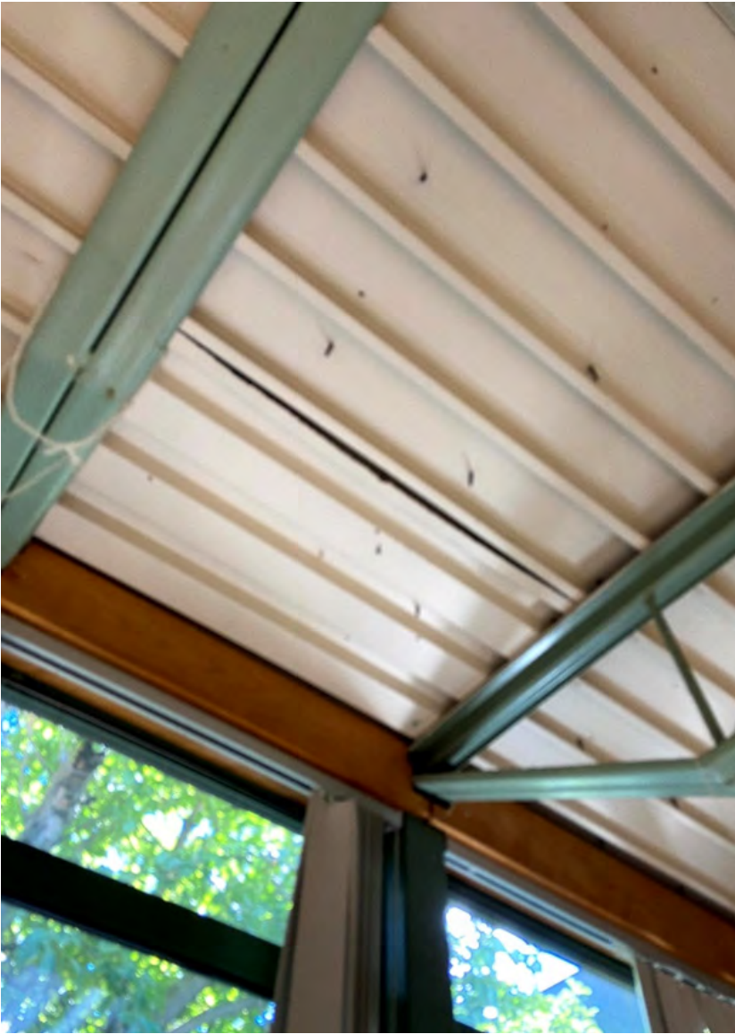
Photo ST-7: Steel roof deck separated side lap
