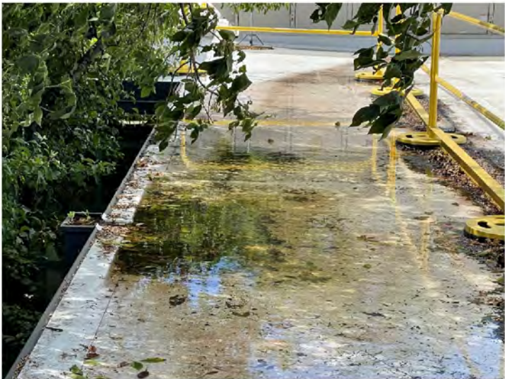
AE-63: Typical ponding of D Wing roof to North of Courtyard
