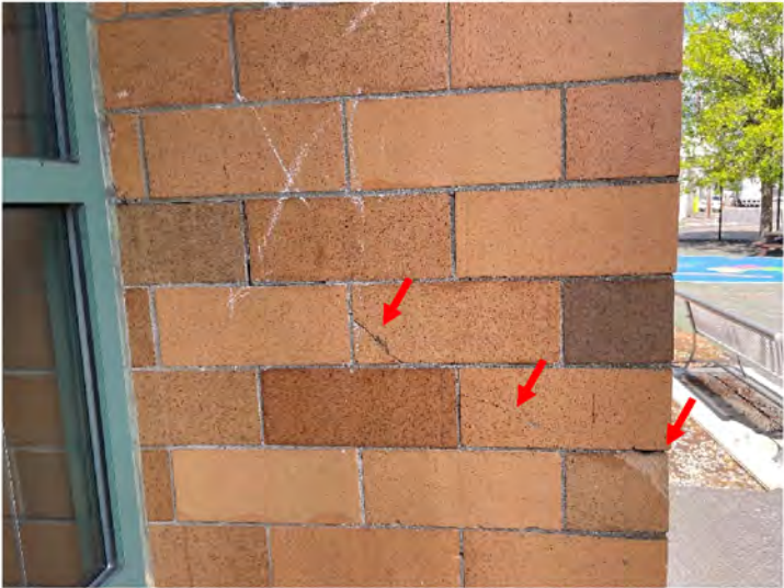
AE-15: Typical glazed brick accent wall. Typical cracking and some spalling observed.
