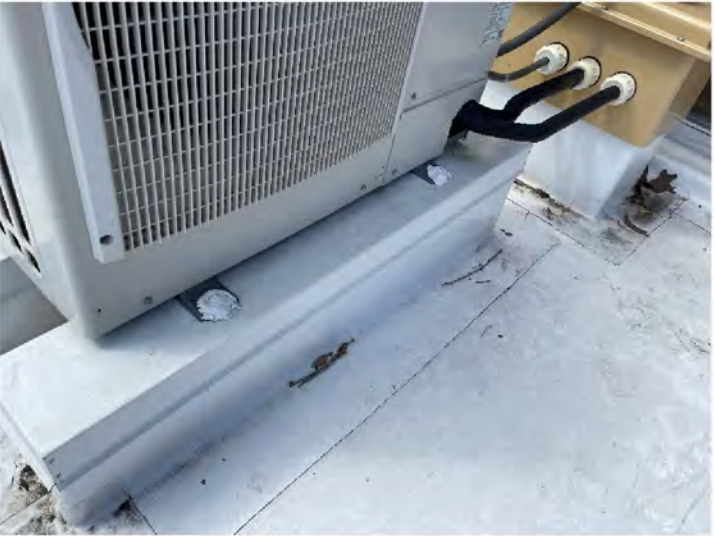
AE-60: Typical condenser unit on sleeper curb
