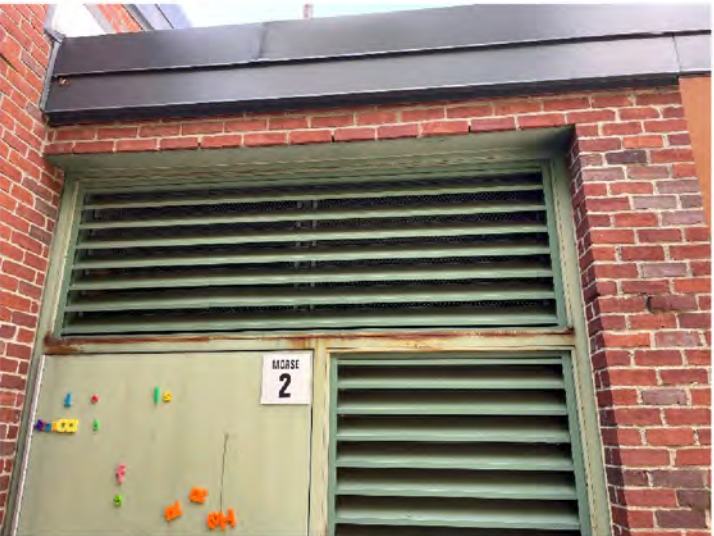
AE-44: Typical metal framed door assembly with louvers, note surface rusting in various areas
