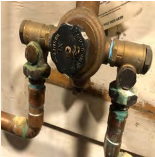
PL-1: Corroded Mixing Valve
