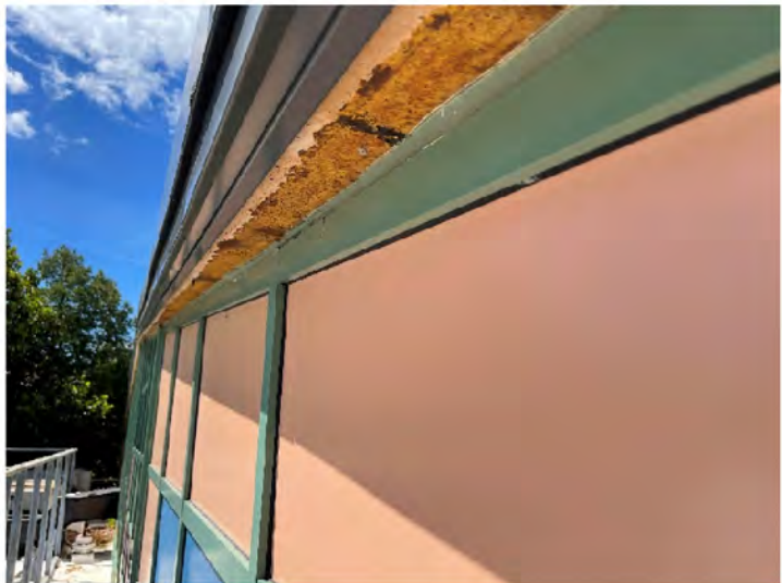
AE-51: Typical rusting of exposed underside of metal roof decking
