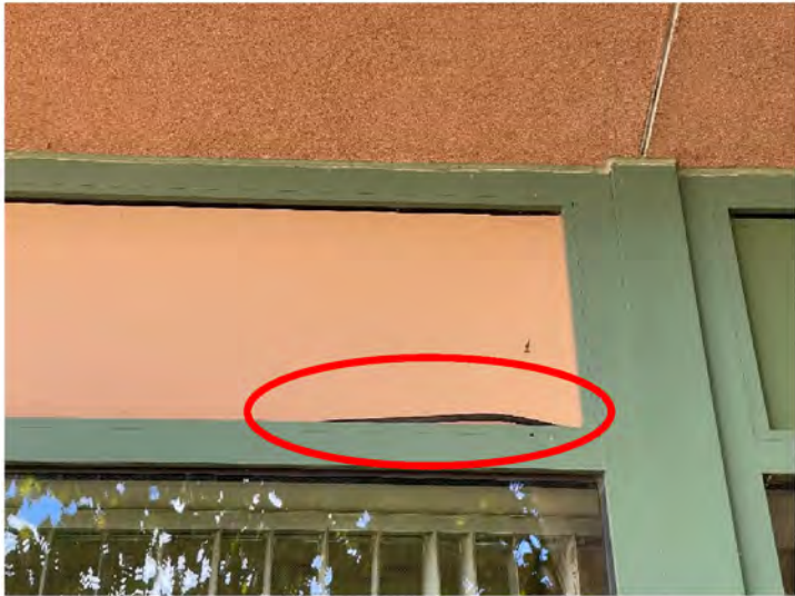
AE-34: Atypical glazing gasket at perimeter of spandrel panel that is not fully engaged to storefront assembly
