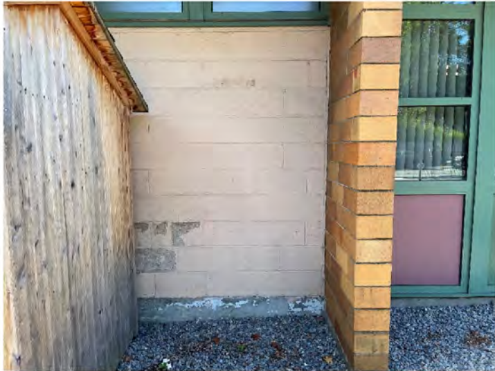
AE-16: Typical peeling paint at concrete block facade
