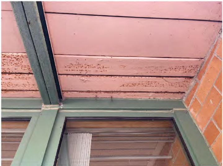
AE-52: Typical rusting and peeling paint at exposed underside of metal roof decking, typical in most locations.
