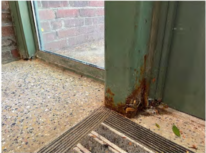
AE-46: Interior of typical exterior metal door frame with rusting at base of jamb framing.
