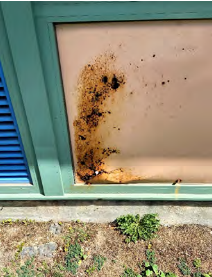
Photo ST-1: Rusting architectural panel at classroom wing
