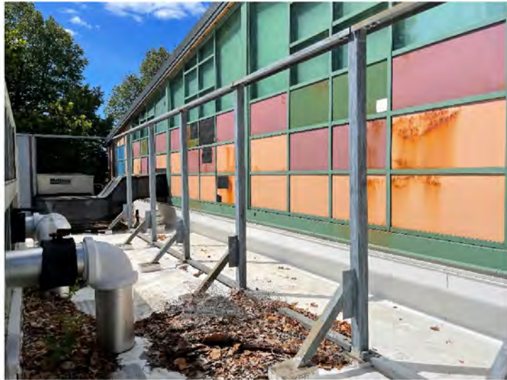
AE-29: Typical curtain wall with fixed lites and insulated metal spandrel panels. Note rusting / corrosion of spandrel panels in many locations.
