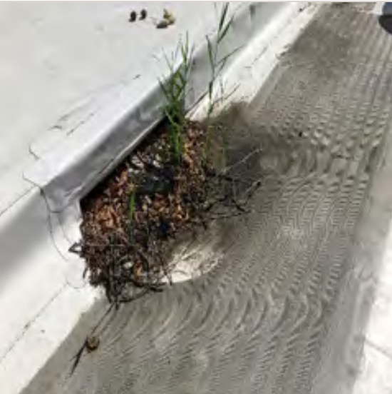
PL-6: Clogged Roof Drain
