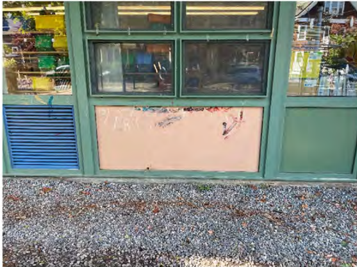
AE-30: Typical peeling paint on spandrel panel installed within storefront assembly
