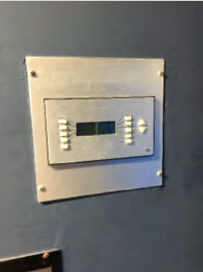
House Lighting Control Station
