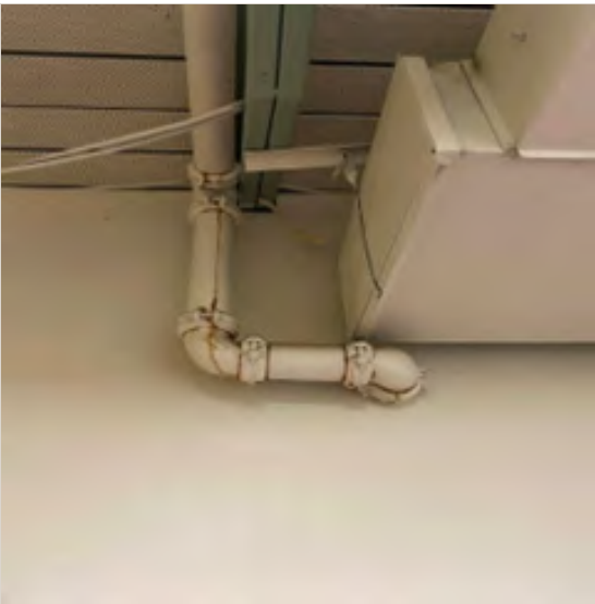
FP-1: Leaking Sprinkler Pipe
