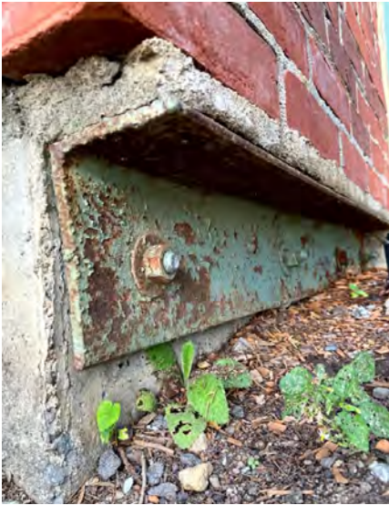
Photo ST-4: Rusting steel angle at base of masonry wall
