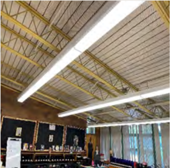
E-3: Classroom Lighting
