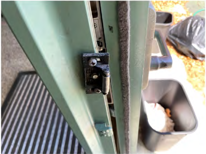
AE-50: Typical door hardware lacking full securement, is loose.
