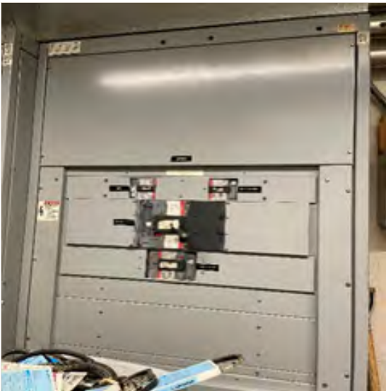
E-1: Main Electrical Service (Entrance)
