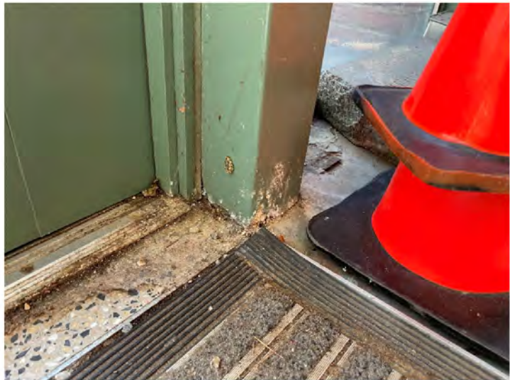
AE-47: Early signs of corrosion on interior at base of exterior door.
