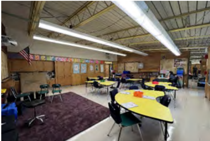
Typical Classroom – E Wing (note open VCT joints)
