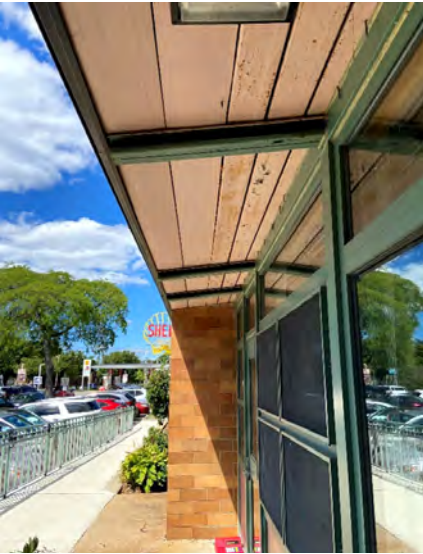
Photo ST-2: Rusting underside of steel roof deck at classroom roof overhang
