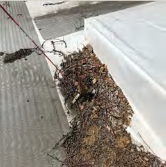
PL-7: Obstructed Roof Drain
