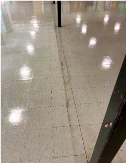
Photo ST-6: Crack in floor finish at cafeteria
