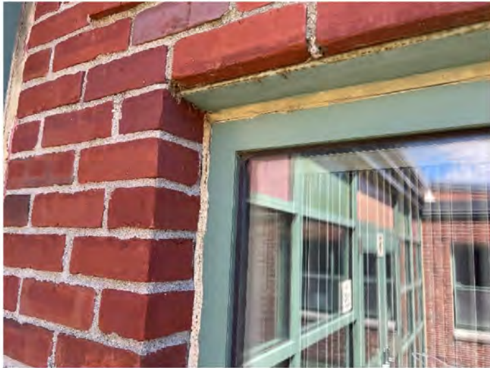
AE-25: Representative rusting of lintel at head of window opening, typical perimeter sealant reaching end of expected service life
