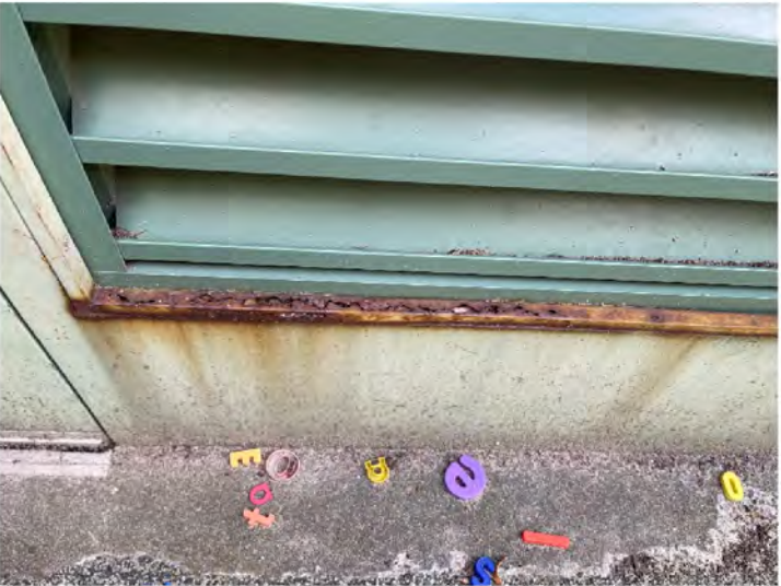
AE-42: Rusting of hollow metal frame below louver infill
