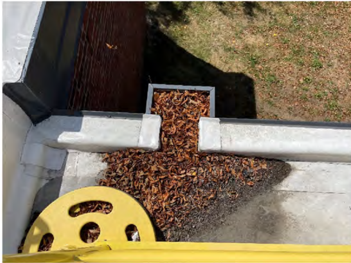
AE-65: Typical downspout clogged with leaves at West Elevation
