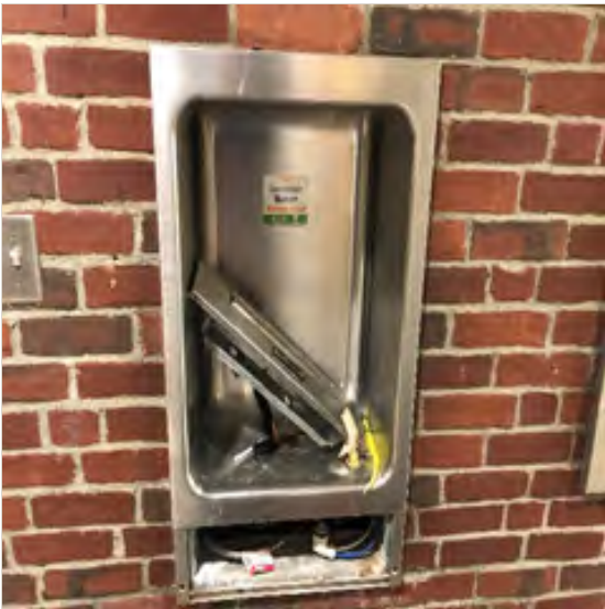
PL-3: Broken Drinking Fountain
