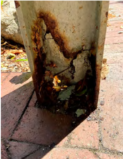
Photo ST-3: Deterioration at base of canopy column
