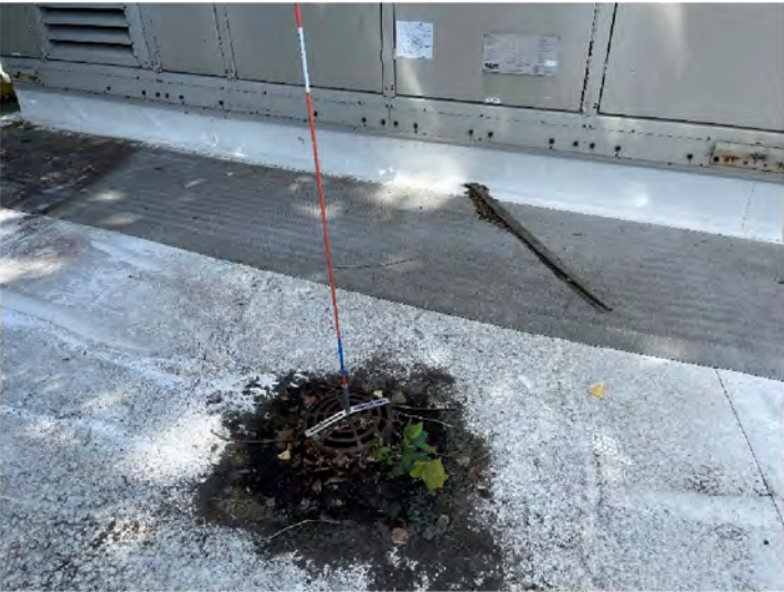
AE-66: Typical internal roof drain with leaves and sediment build up
