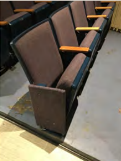
Damaged Auditorium Seat
