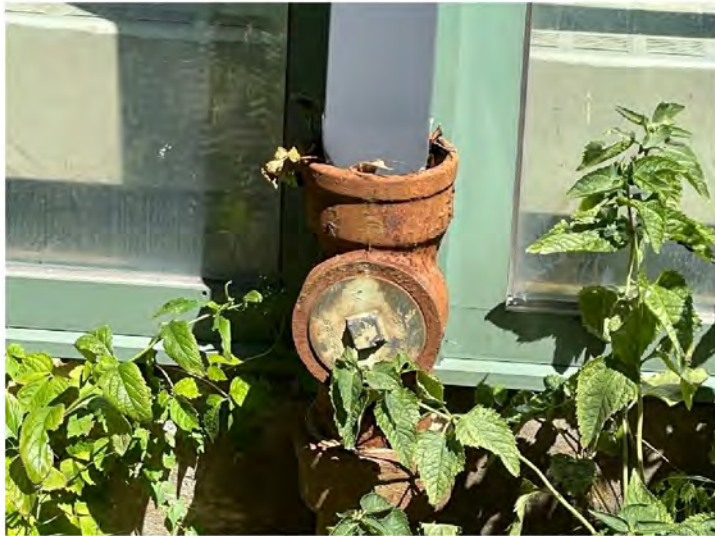
AE-62: Base of downspout in Courtyard appears clogged with leaves
