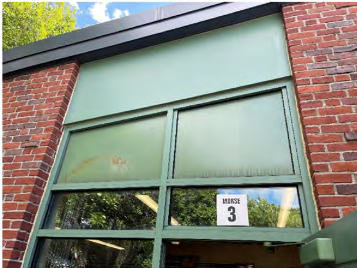
AE-35: Typical storefront assembly with metal panel above, rusting of insulated metal spandrel panel within storefront
