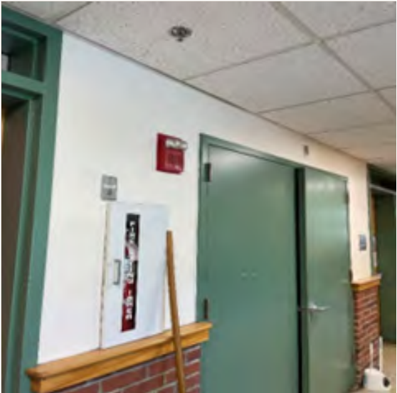
E-5: Existing Fire Alarm Device
