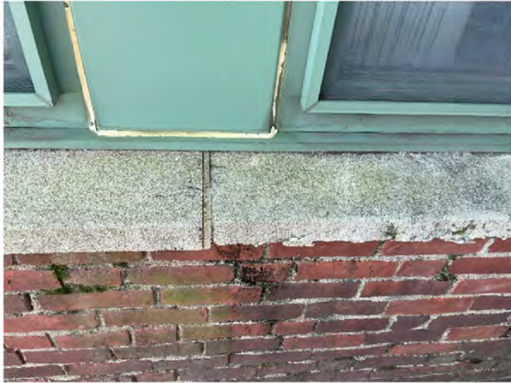
AE-14: Atypical precast concrete window sill and brick masonry with evidence of excess moisture due to moss growth.
