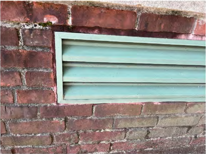
AE-41: Typical louver within masonry façade, perimeter sealant nearing end of expected service life
