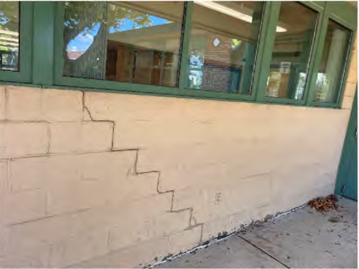
AE-20: Step cracking of concrete block at East entrance to B Wing
