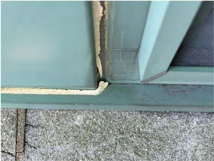
AE-37: Typical failed perimeter sealant at storefront assembly
