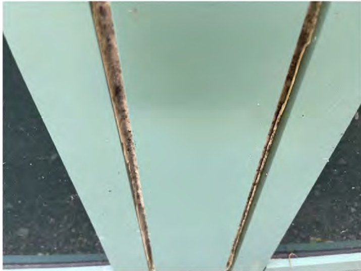
AE-38: Representative failed sealant between storefront assemblies
