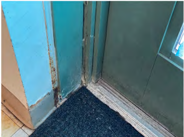
AE-48: Typical surface rusting on interior at base of typical exterior door.
