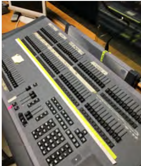
Theatrical Lighting Control Console
