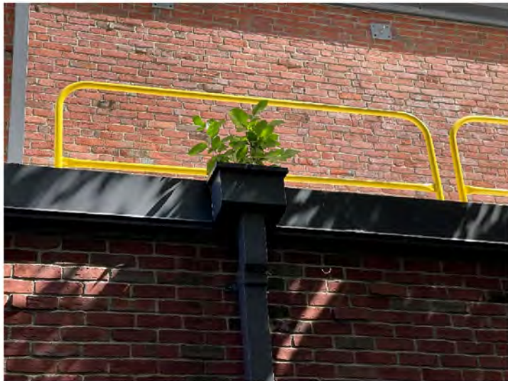
AE-64: Typical downspout at West Elevation with vegetation growth due to leaves filling top of downspout
