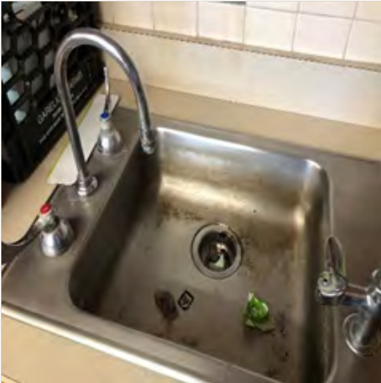
PL-5: Corroded Classroom Sink
