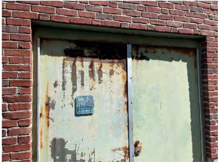
AE-45: Representative exterior metal door with significant rusting
