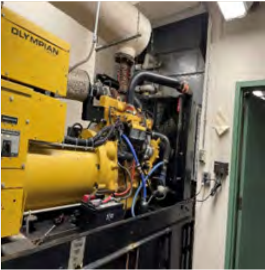
E-2: Diesel Generator
