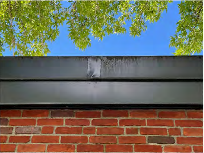
AE-18: Roof edge at D Wing where roof drains over roof edge, onto façade below.
