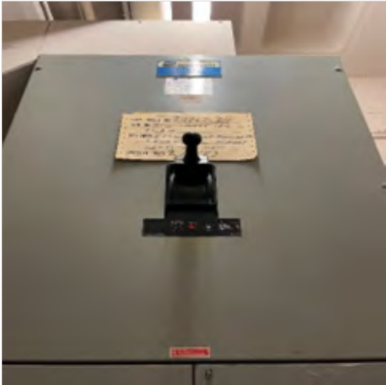
E-1: Main Electrical Service (Entrance)
