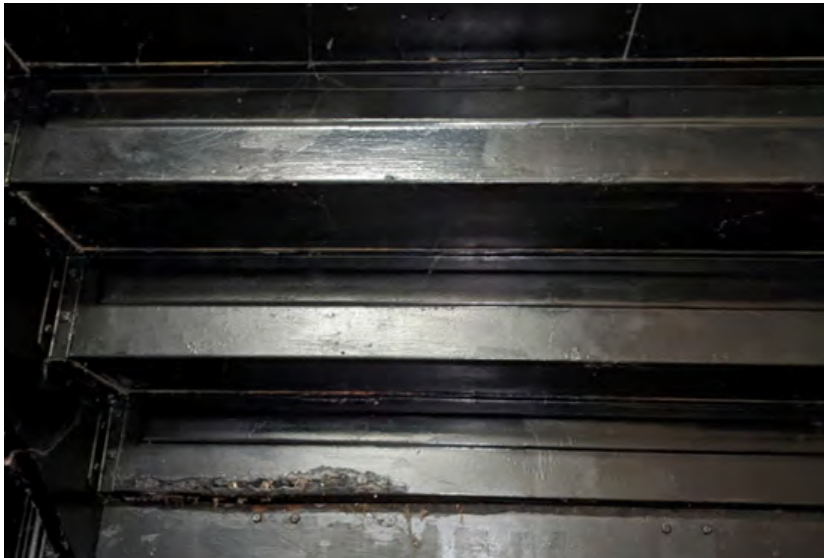
Photo ST-5: Corrosion of Stair Tread/Riser
