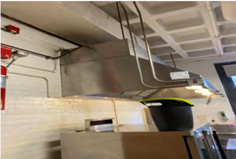
FS-2: The exhaust hood in this kitchen is extremely old and not properly closed off to the ceiling above. The angled surfaces are an area that collect dirt, debris and dust and cannot be properly cleaned. Modern code requires vertical closure panels from the top of the hood to the finished ceiling.
