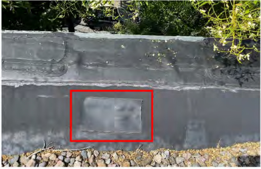
AE-29: Typical patch in EPDM roofing lacking termination lap sealant at perimeter
