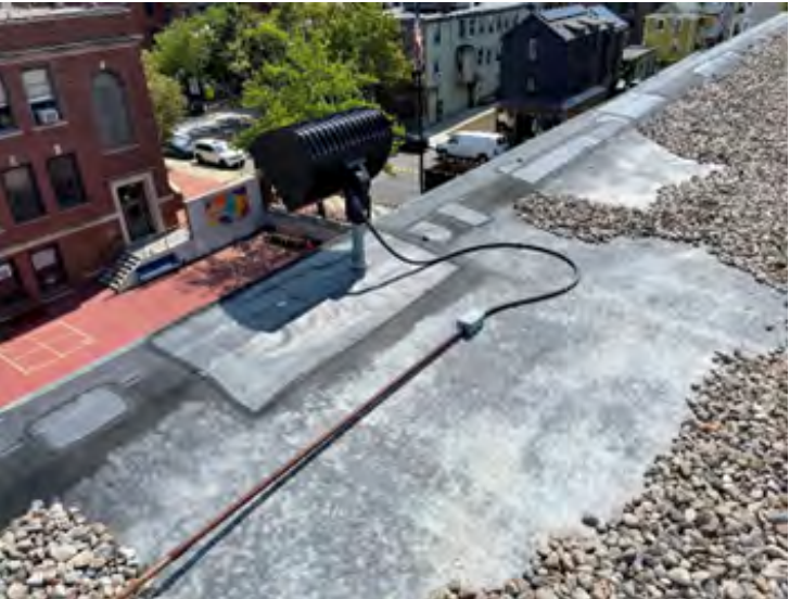
AE-D: Representative roof edge condition at EPDM roof. Note multiple patches due to damage over time.
