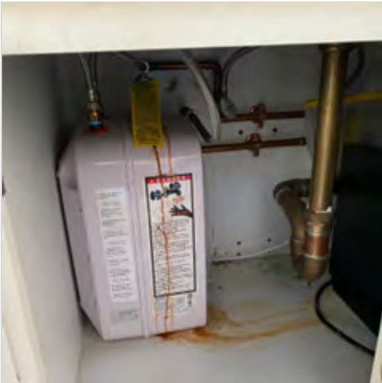
PL-2: Corrosion on Point of use Water Heater
