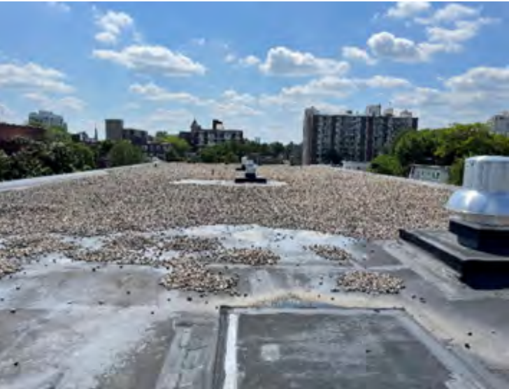
AE-C: Representative view of roof. Note ballast is not evenly distributed, leaving areas of exposed / unsecured EPDM.
