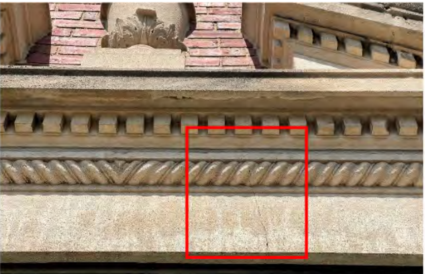
AE-16: Representative cracked limestone at building entrance
