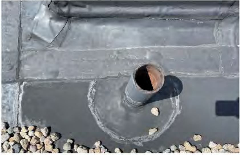
AE-31: Typical vent pipe penetration through roof, failing lap sealant at perimeter of flashing boot
