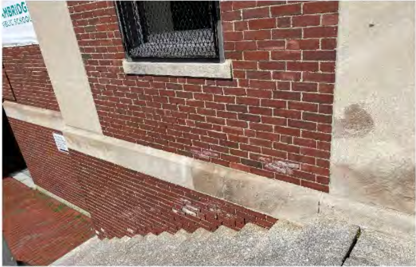
AE-9: Representative precast concrete coping cap at West Wing. Note failed sealants between caps.
