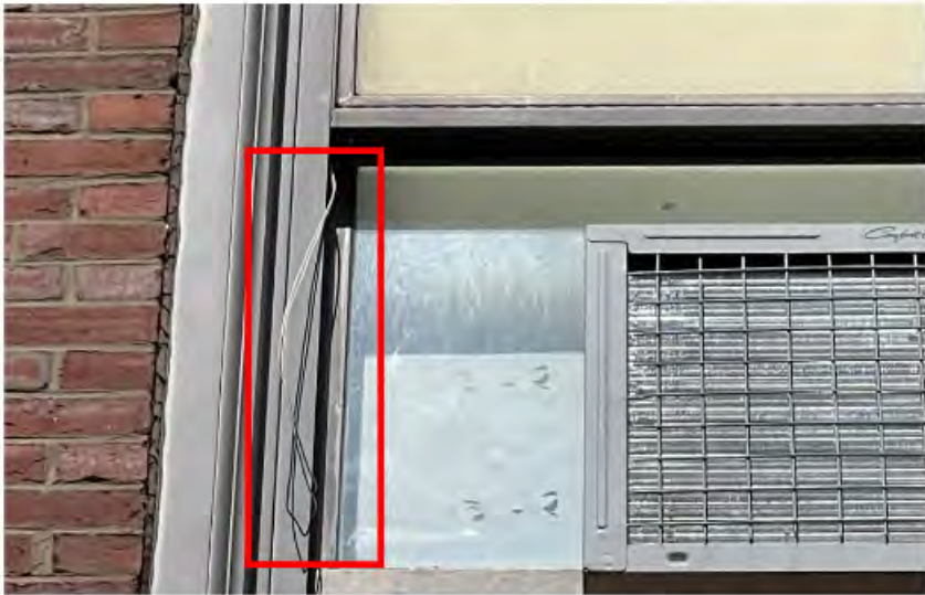
AE-24: Representative aluminum window where sash cord is not fully engaged within window frame, is exposed on exterior
