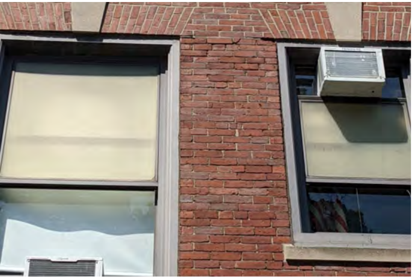
Photo ST-4: Brick Joints in Need of Repointing
