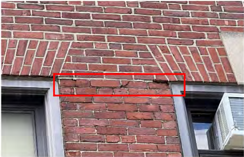
AE-11: Representative rust jacking of steel lintels, resulting in cracked brick and mortar
