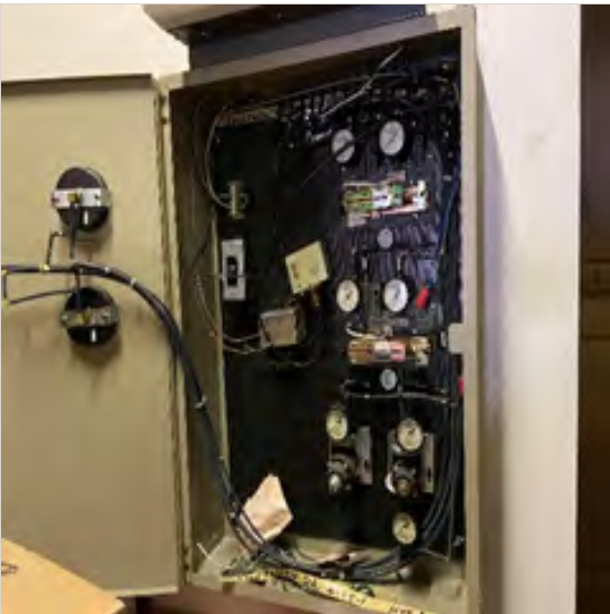
M-6: Original Pneumatic Control Panel
