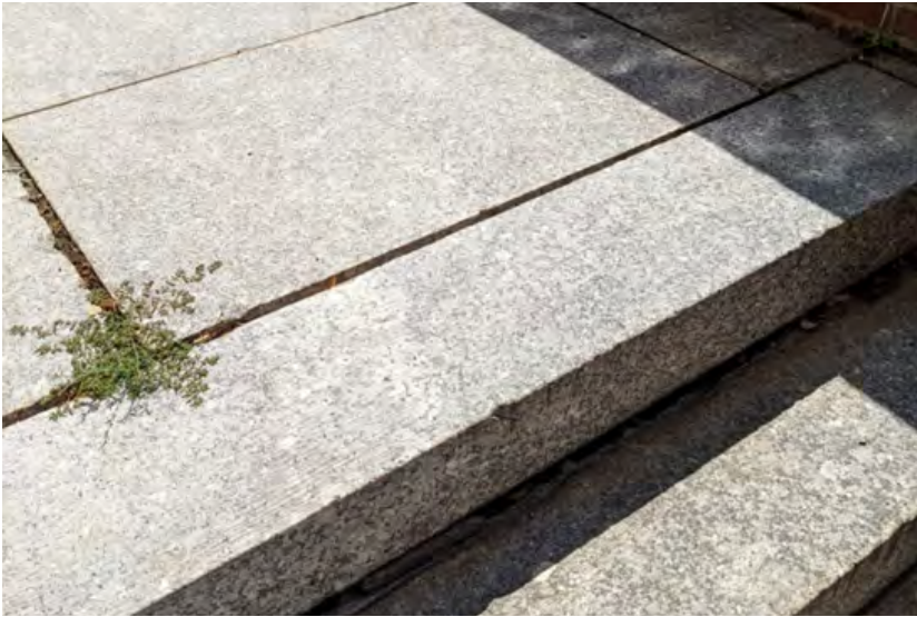
Photo ST-2: Open Joints in Granite
