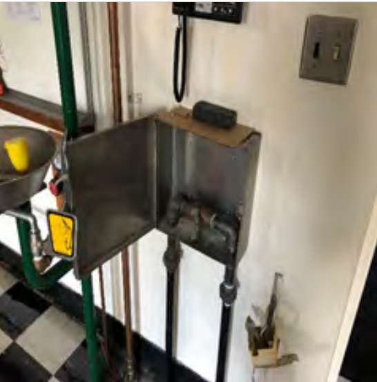
PL-9: Existing Gas Valve Cabinet
