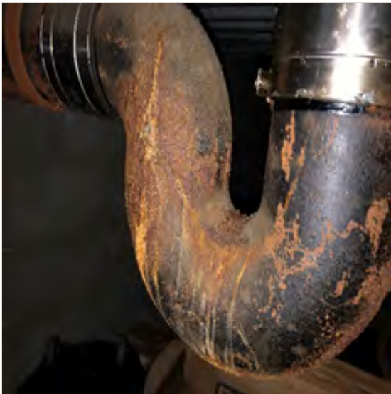
PL-6: Cracked P-Trap
