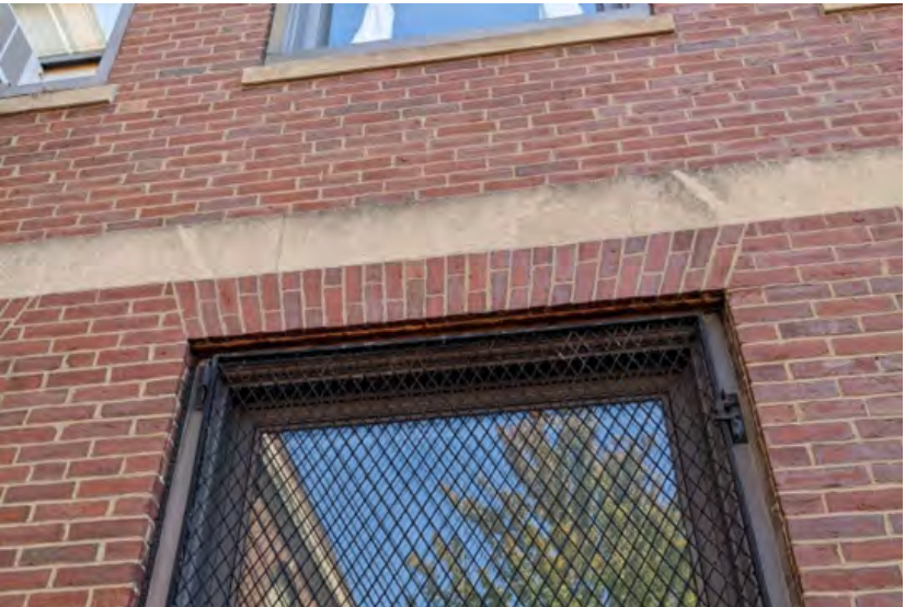
Photo ST-3: Sagging Lintel (Rust-Jacking)
