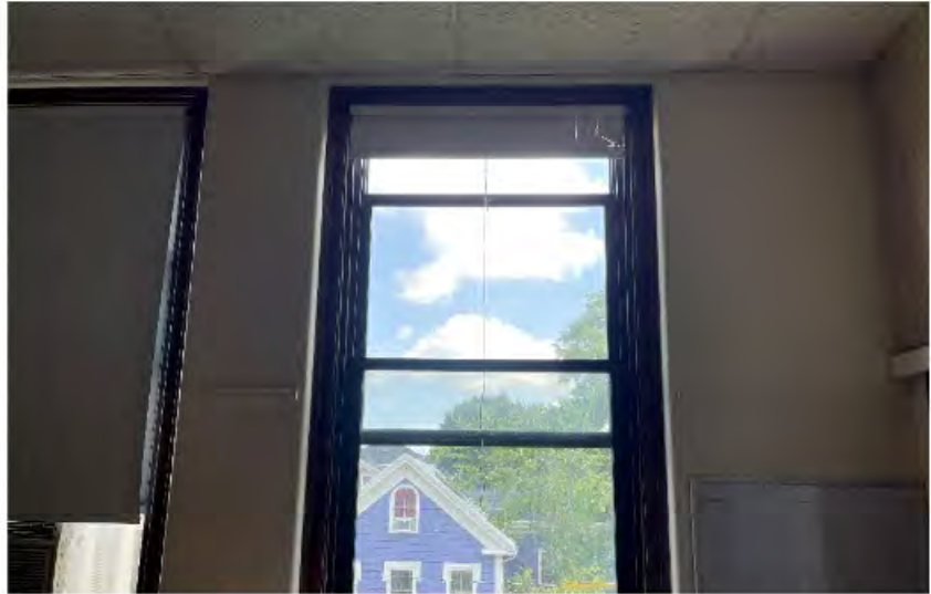
AE-36: Interior of representative window where upper sash is difficult to remain closed
