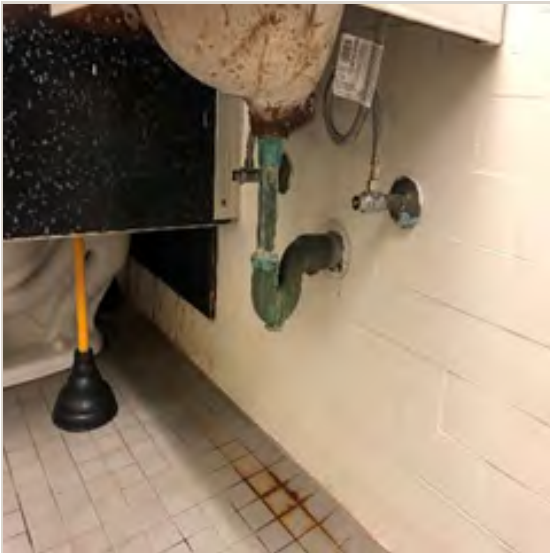
PL-4: Corroded Lavatory
