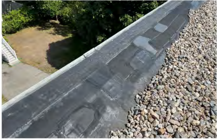
AE-28: Typical patches in EPDM along perimeter of roof
