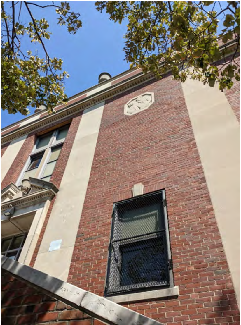
Photo ST-8: Bowing/Bulging Exterior Facade
