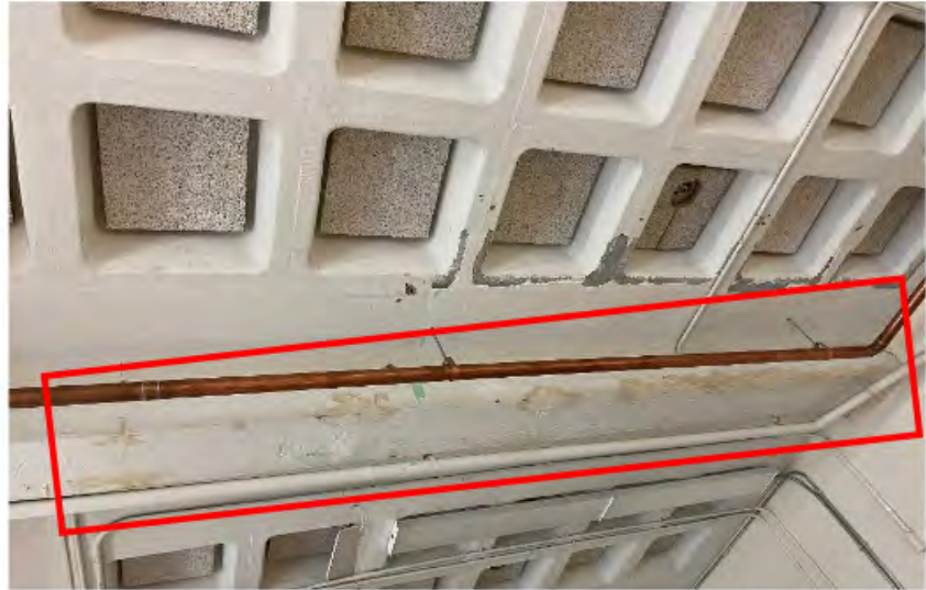
AE-35: Interior leak within Room 7, located below Room 109 above
