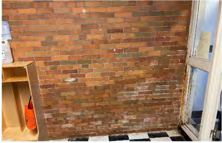
AE-26: Efflorescence on brick and rusting of door frame on interior of building at lower level below Main entrance at East Wing
