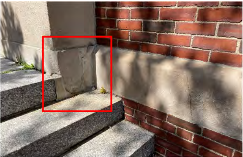
AE-15: Representative spalled limestone near building entrance, cracked limestone band
