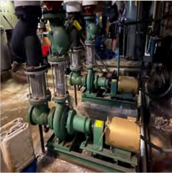
M-2: Hot Water Pumps
