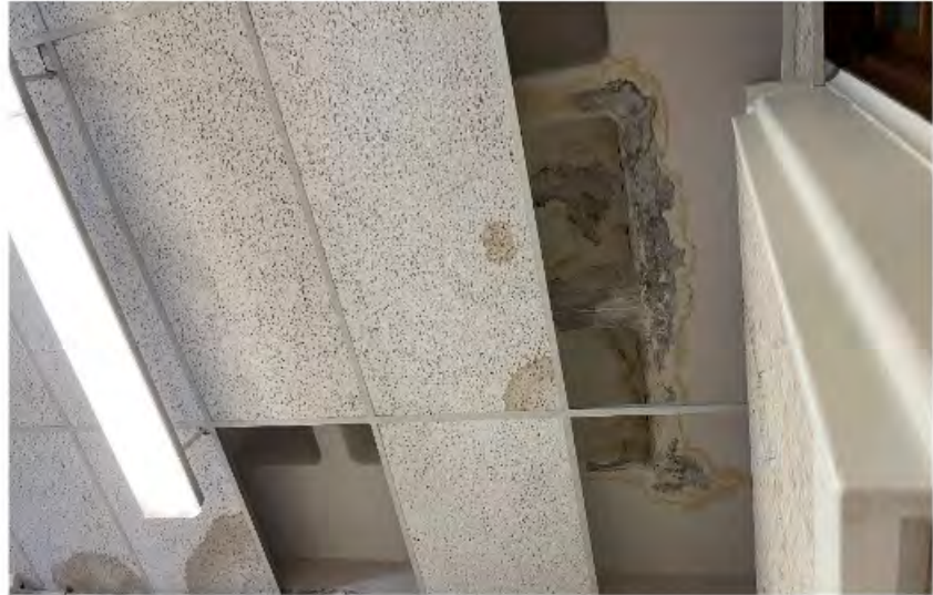
AE-33: Interior leak within Room 109 and adjacent hallway. Leak is within interior of building, not near roof edge
