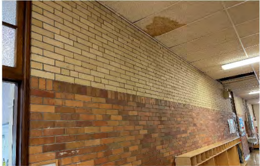
AE-34: Interior leak within hallway adjacent to Room 109. Leak is within interior of building, not near roof edge
