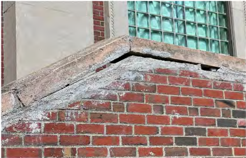
AE-19: Typical spalled and displaced cast stone cap at building entrance
