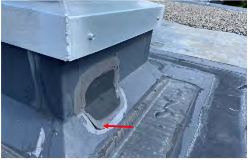
AE-32: Typical EPDM patch applied to MEP curb that is lacking adhesion, lap sealant has failed
