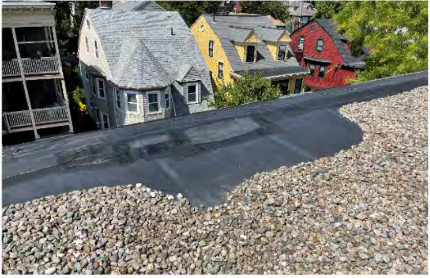
AE-30: Typical patches in EPDM at perimeter of roof. Note, EPDM is loose laid on this roof, is tented along perimeter in most conditions.
