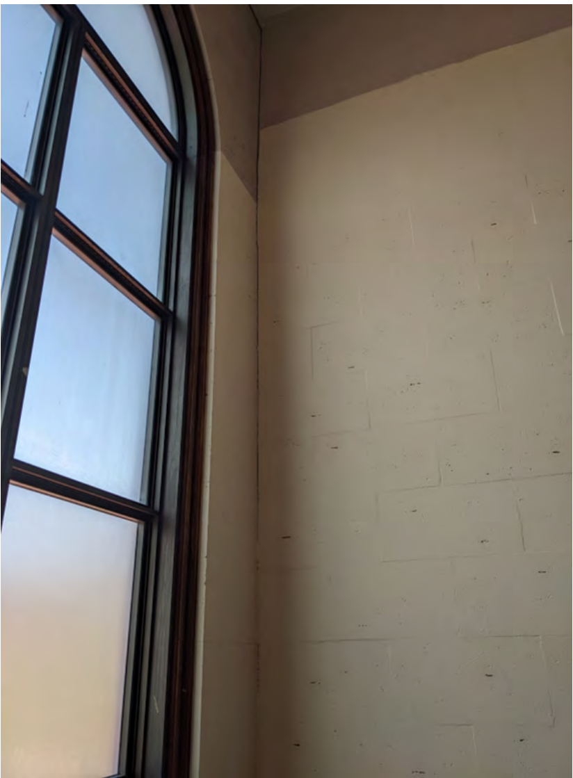
Photo ST-7: Gap Between Perpendicular Walls
