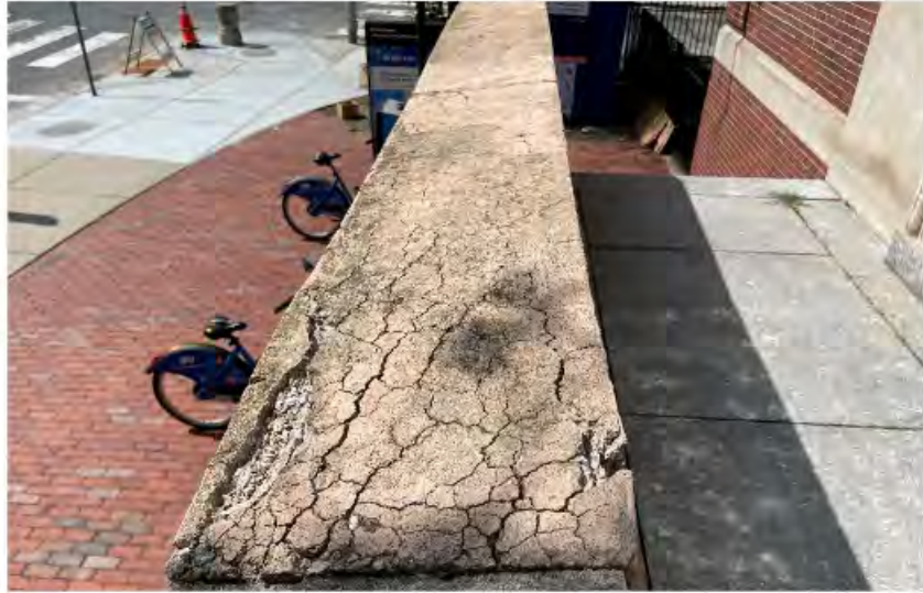
AE-18: Typical spalled cast stone cap at exterior stair to building entrance
