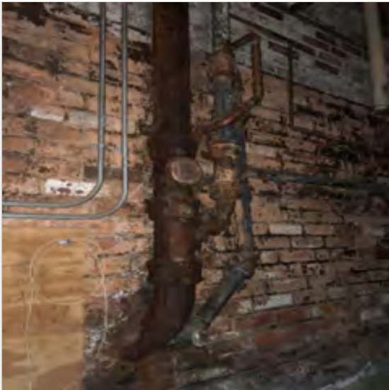
PL-7: Heavily Corroded Cast Iron Pipe
