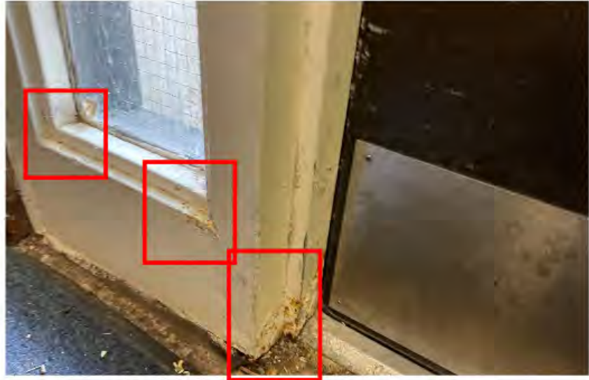
AE-25: Interior of typical exterior door: Note rusting of door frame
