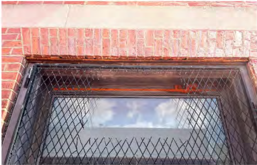
AE-23: Window at lower level where perimeter of upper sash is filled with spray foam insulation
