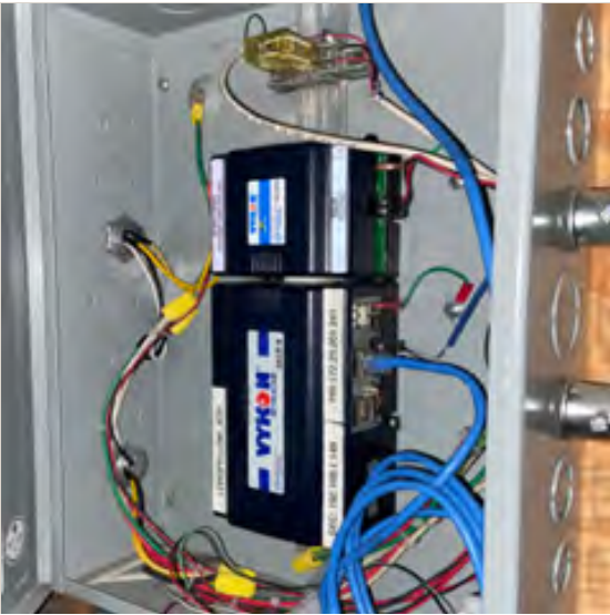
M-7: Upgraded Network Controller
