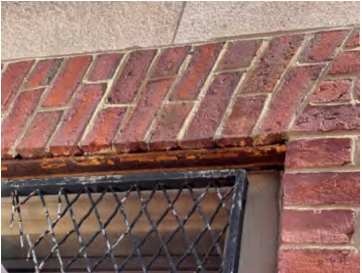
AE-B: Representative rusting steel lintel at window head
