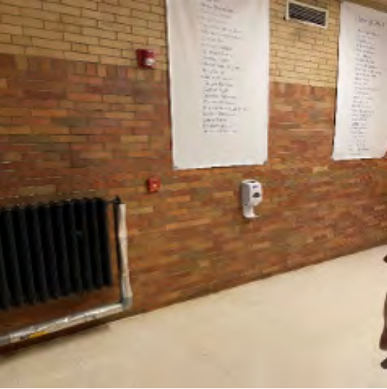
E-5: Existing Fire Alarm Device
