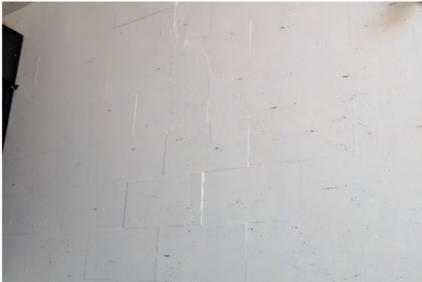
Photo ST-6: Cracking and Displacement of Masonry Units - Stair No. 1
