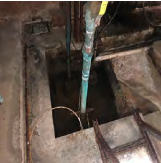
PL-8: Heavily Corroded Sump Pump Discharge Piping
