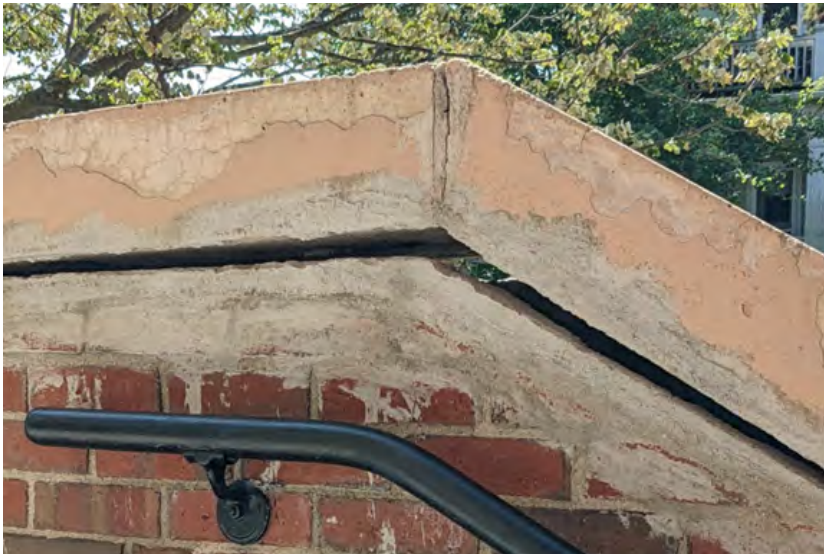
Photo ST-1: Loose Wall Cap at Site Stair
