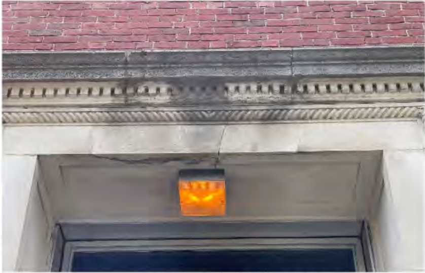
AE-17: Representative cracked limestone at building entrance
