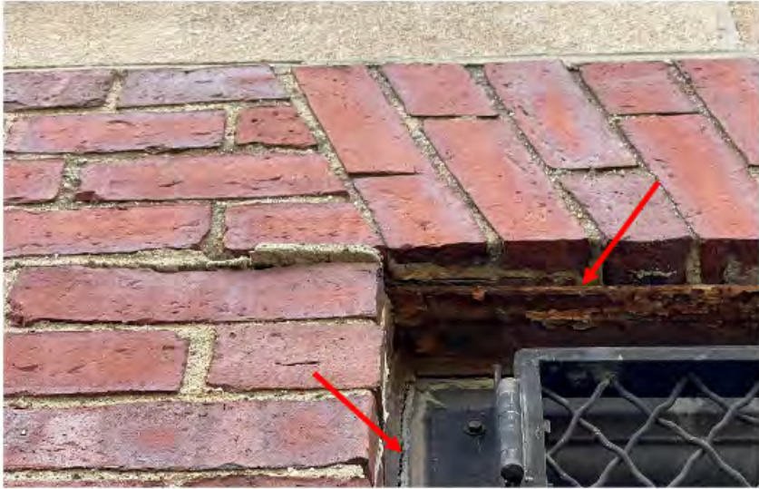
AE-22: Representative aluminum window: Typical rusted lintel with peeling paint, typical failed window perimeter sealant
