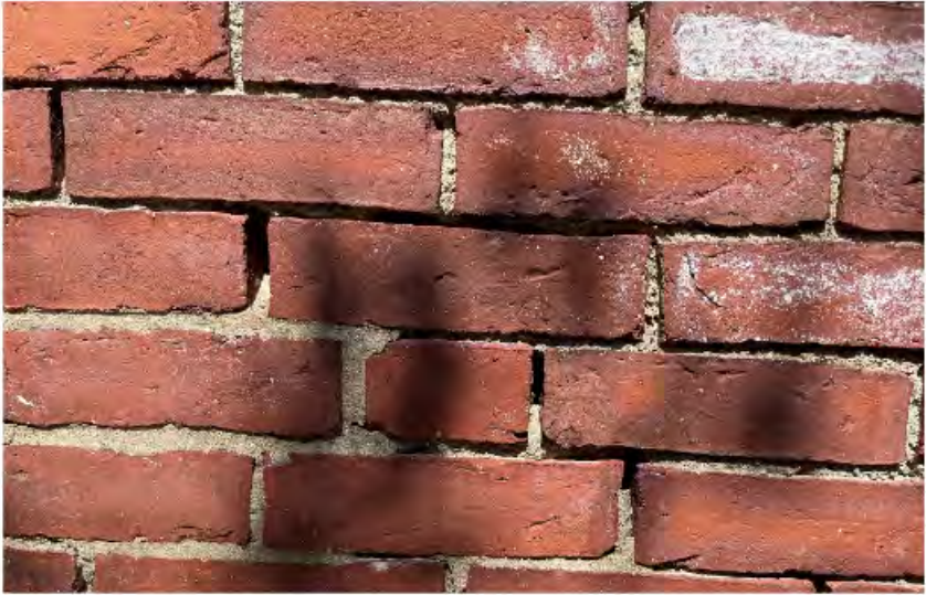
AE-10: Representative brick masonry with deteriorated mortar, typical near stairs at building entrances
