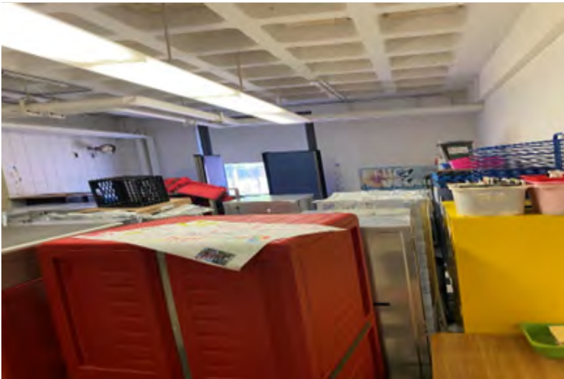
FS-1: There is no finished ceiling in this space which is required by health code in commercial kitchens. Due to the lack of a finished dropped ceiling, all utilities and mechanical equipment is exposed and this prevents proper cleanability of the kitchen space.
