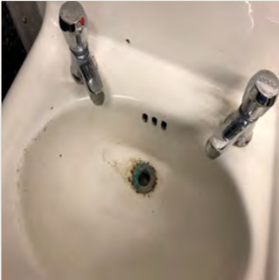
PL-3: Outdated Lavatory
