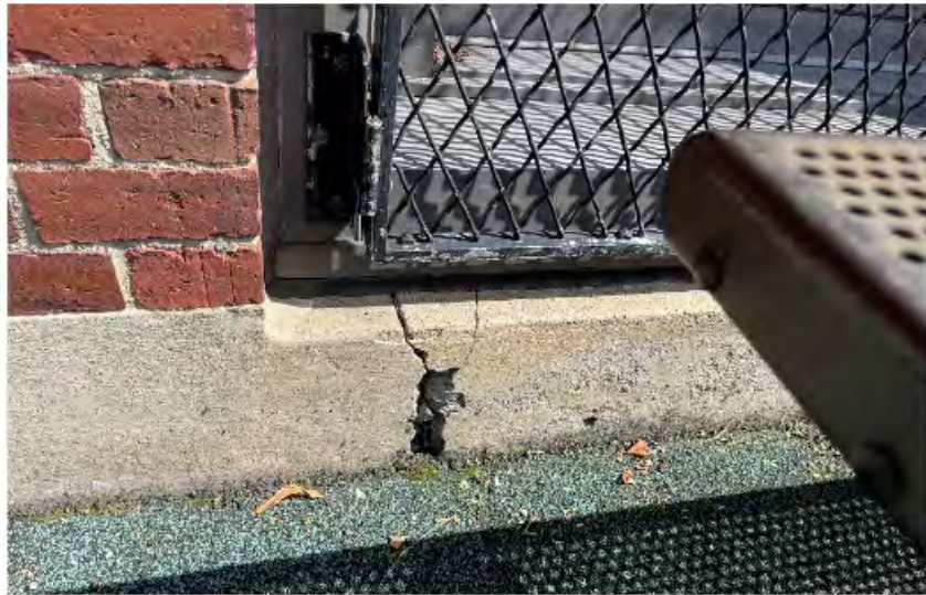
AE-20: Typical cracked and spalled foundation wall
