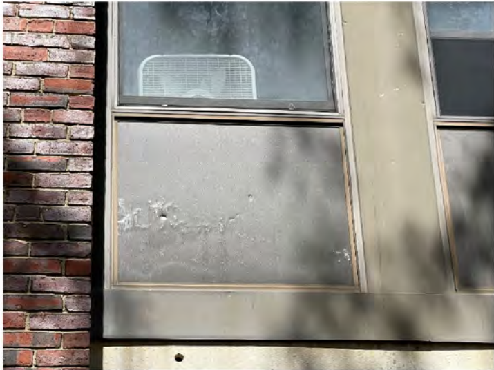
AE-26: Typical metal spandrel panel below typical aluminum window assembly. Not corrosion of panel, typical in many locations.
