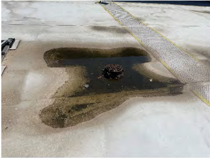
AE-52: Typical standing water and sediment build up at drain sump
