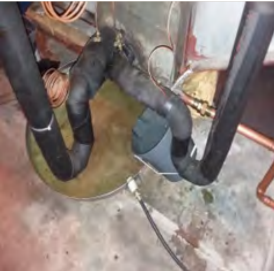
M-4: Existing Air Handling Unit With Condensate Pan Leakage
