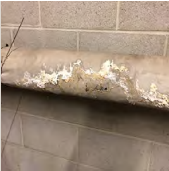
PL-4: Insulation with Mold
