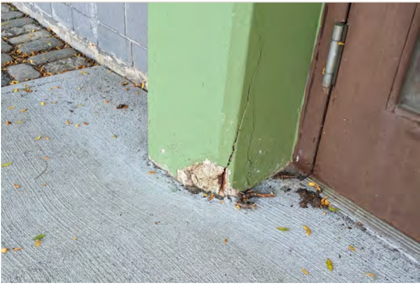
Photo ST-3: Cracked Concrete Encasement
