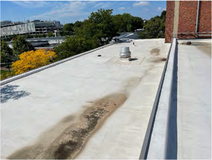
AE-51: Typical standing water and gathered sediment at low roof
