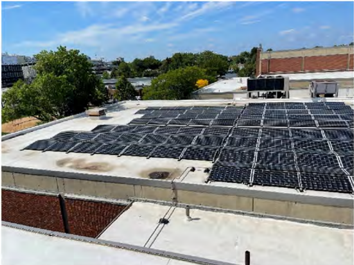
AE-45: Partial view of typical roof area, covered with PV panels
