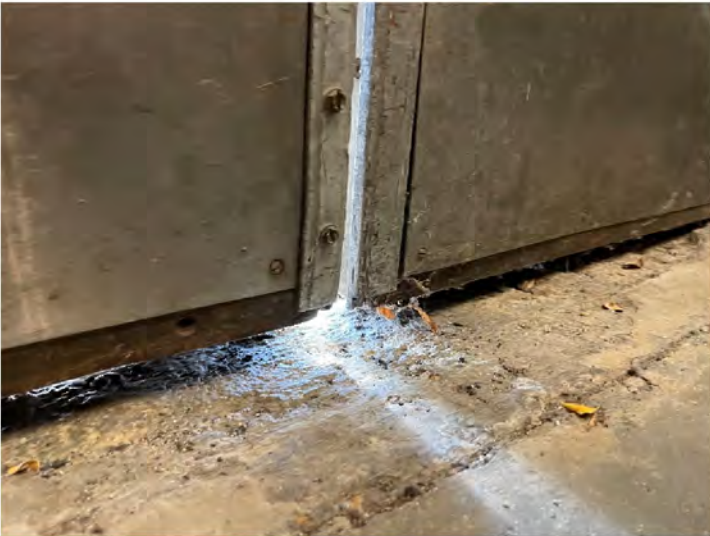
AE-41: Interior condition at base of door where daylight is visible due to failed weatherstripping
