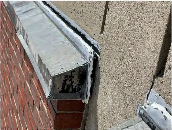
AE-16: Representative metal flashing along top of brick masonry façade. Note flashing is no longer engaged to concrete facade, sealants have failed.
