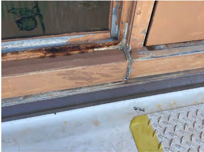
AE-28: Exterior of typical steel framed window assembly located above roof. Note rusting of window frame and various layers of failed sealant.
