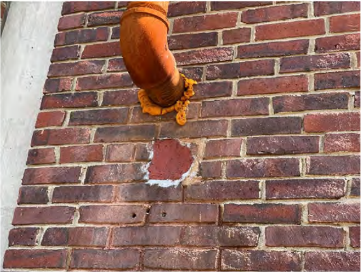
AE-17: Typical façade penetrations filled with spray foam insulation.
