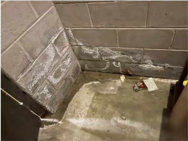
AE-63: Interior of hallway adjacent to Auditorium where ponded water and efflorescence are present due to active water leakage.
