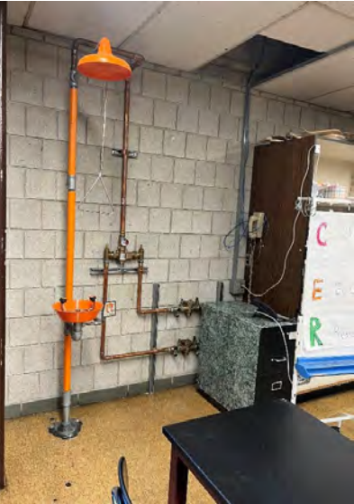
Exposed Piping in Science
