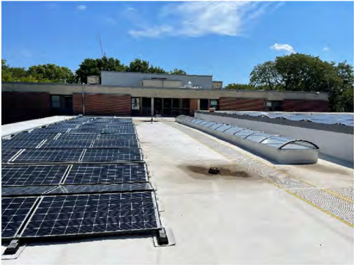
AE-47: Representative PV panels and skylight over main lobby
