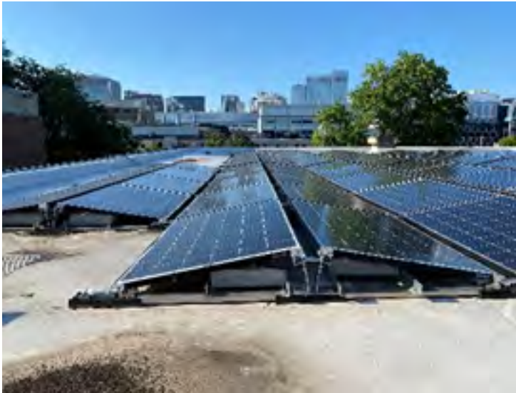
E-5: Solar panels – roof
