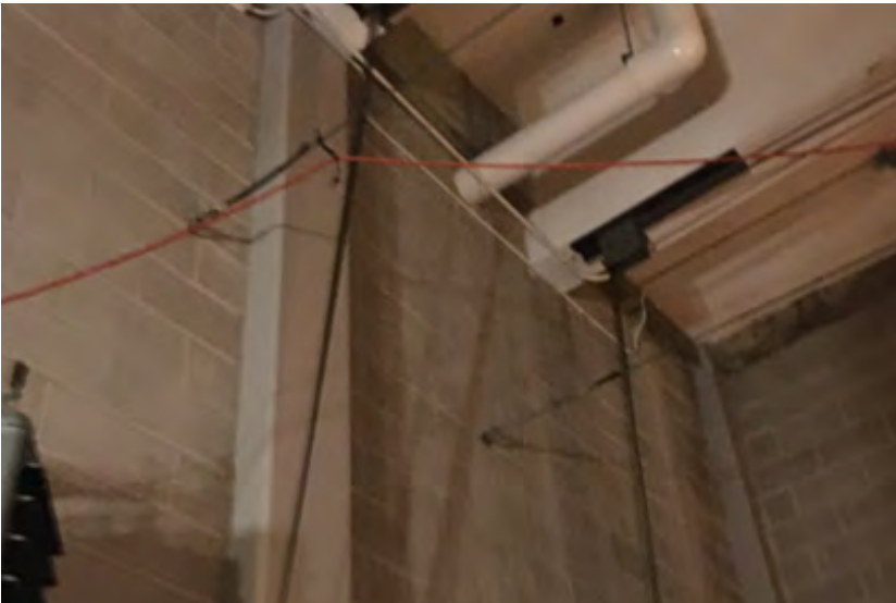
Temporary Cable Suspended Backstage
