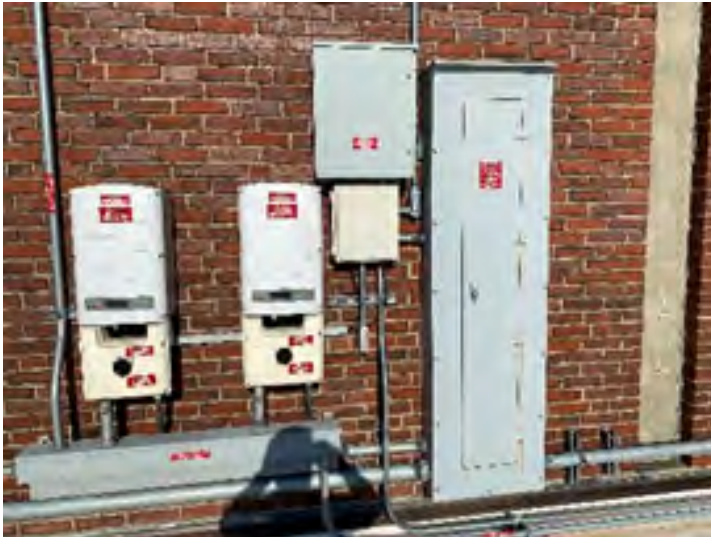
E-6: PV equipment – Subpanel, Inverters, Disconnects
