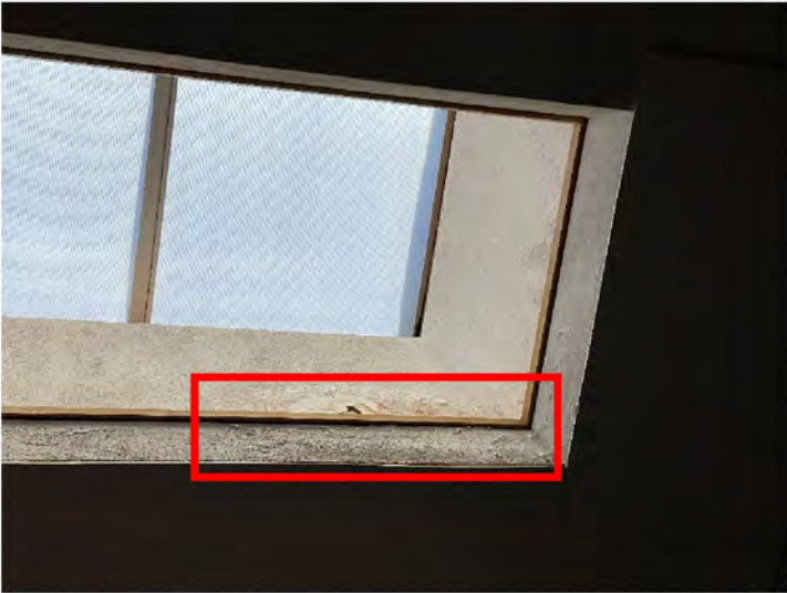
AE-64: Interior of skylight at main lobby where there is ceiling damage from water leakage
