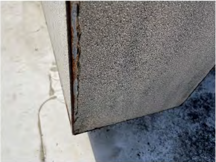
AE-22: Typical surface rusting and some cracking of cementitious cladding at roof monitors.
