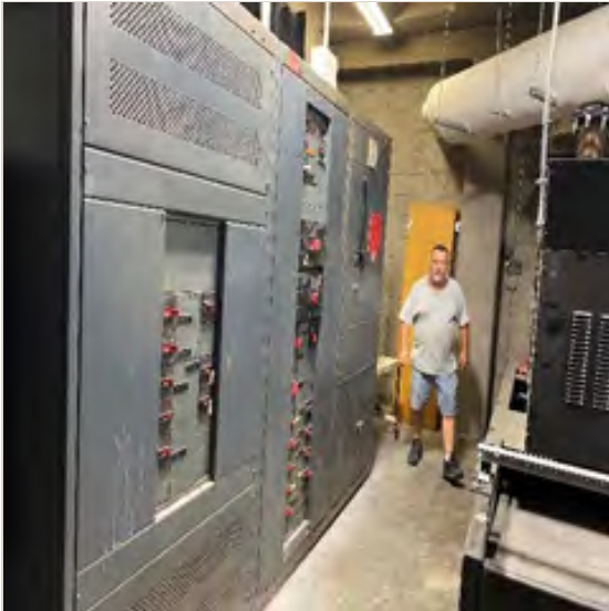
E-1: Main Electrical Service (Entrance)
