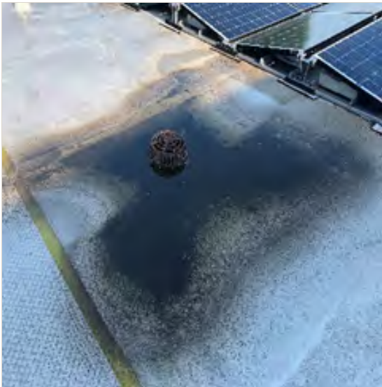
PL-9: Ponding at Roof Drain.
