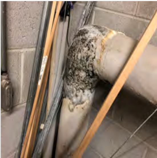
PL-3: Insulation with Mold
