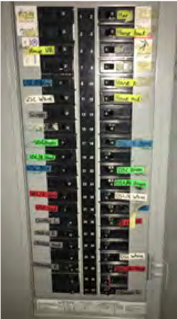
Local Panelboard Used to Control Stage Lighting
