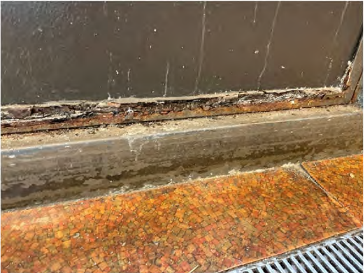
AE-32: Interior of typical steel window frame where rusting is occurring
