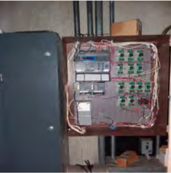
M-6: JCI Air Handling Unit DDC Control Panel
