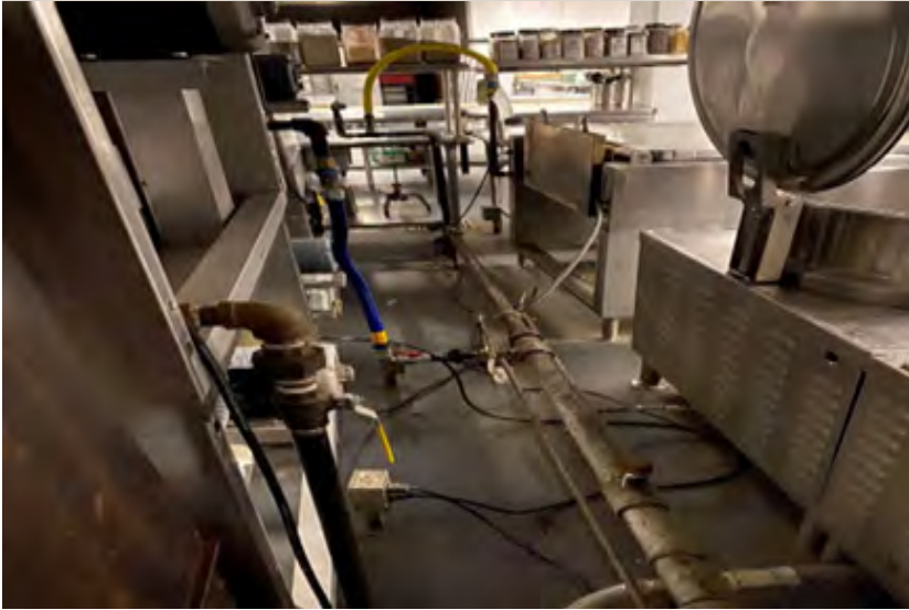
FS-1: Exposed utilities in the cooking area present cleanability issues. Utilities should be enclosed and provided with a smooth washable surface.
