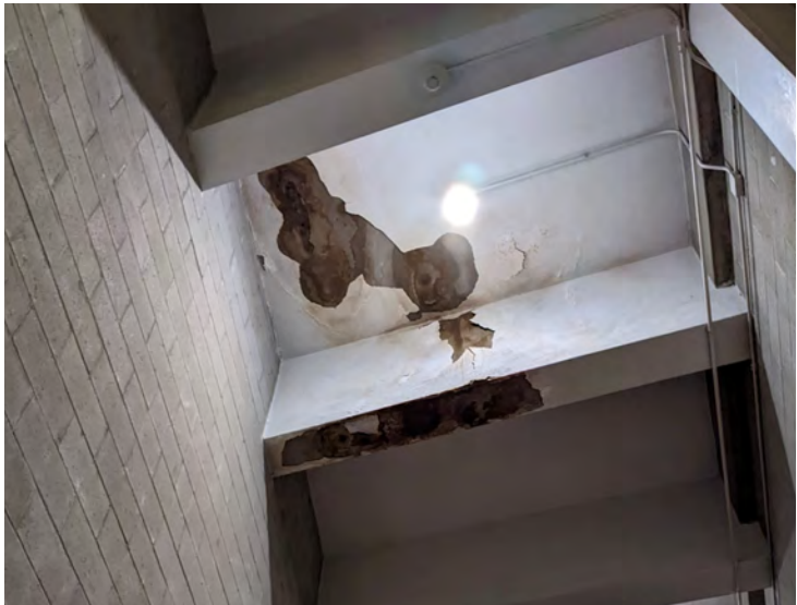
Photo ST-2: Water-Stained Finishes above Stage
