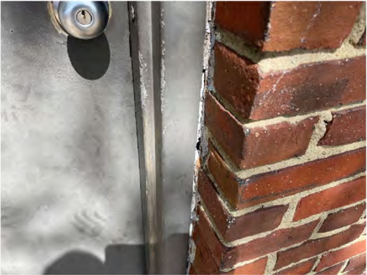
AE-40: Typical failed perimeter sealant at typical exterior door
