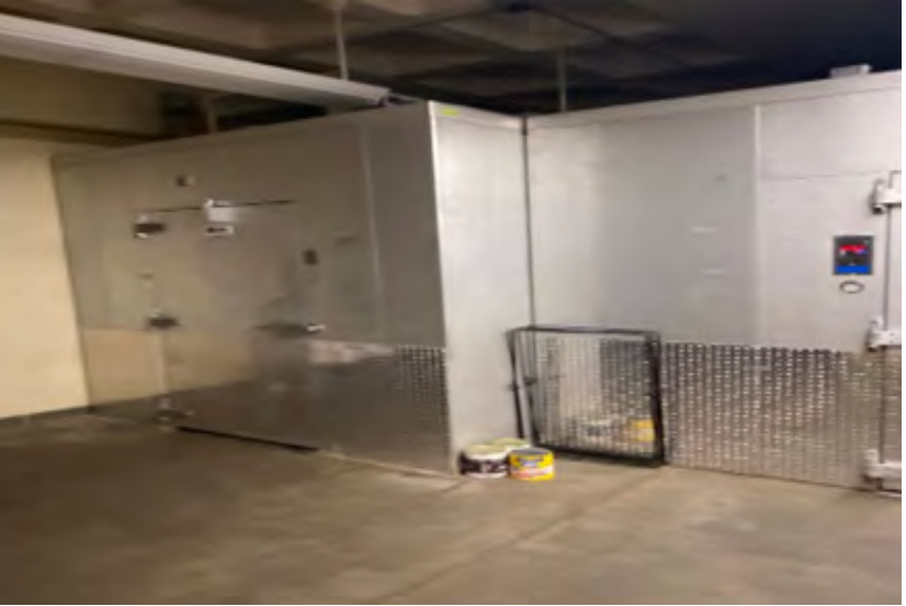
FS-3: Walk-in coolers are required to have vertical closure panels from the top of the box to the finished ceiling. This prevents dirt, dust and debris build up and is required by code. The floor at the exterior of the box is required to be coved in order to properly mop and clean the space. Neither of these requirements are met and require updates.
