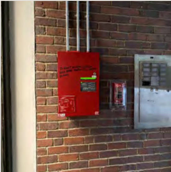
E-5: Existing Fire Alarm Control Panel
