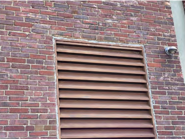
AE-36: Representative mechanical louver on exterior of building, note failed perimeter sealant
