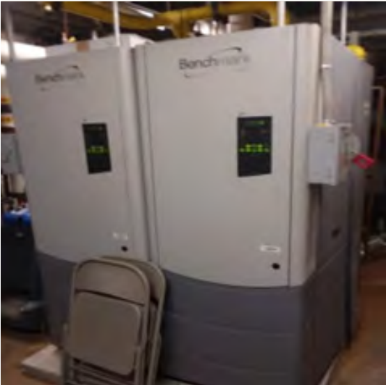
M-1: (2) of (4) existing Benchmark Aerco boilers
