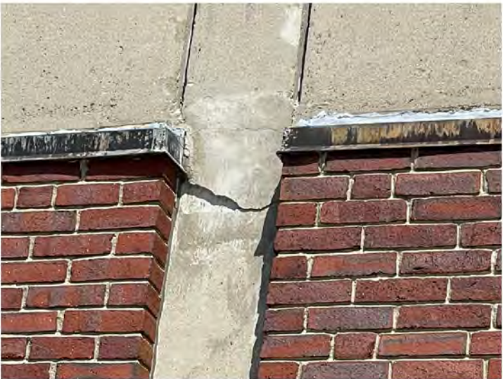
AE-14: Typical previous concrete repair at exposed cast in place concrete that has cracked and spalled.
