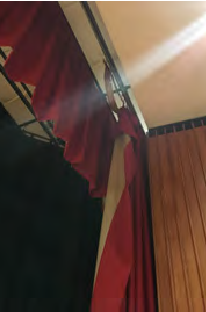
Damaged Stage Drapery
