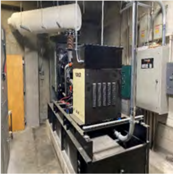
E-2 Generator – Good Condition
