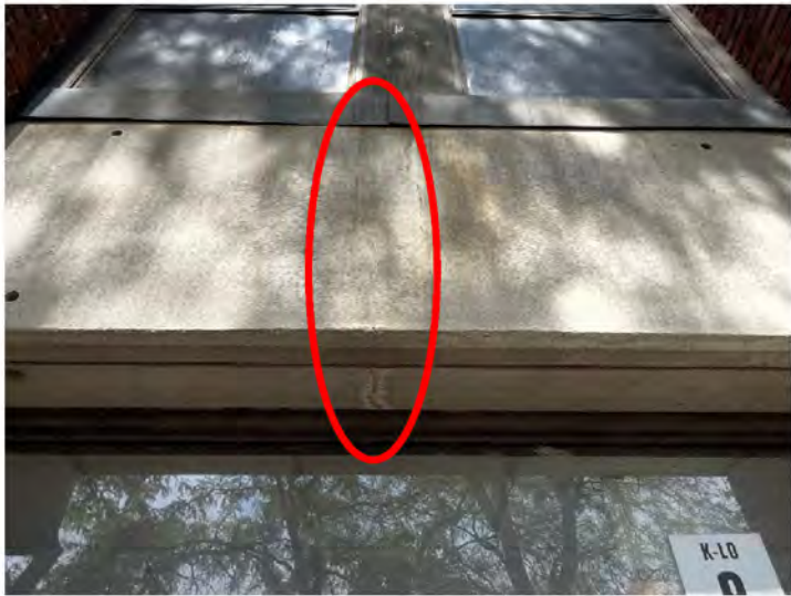
AE-12: Representative vertical cracking at exposed concrete between floors. Condition observed in many locations throughout building.
