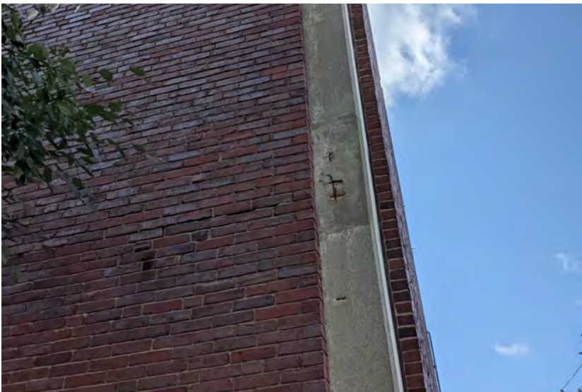
Photo ST-4: Exposed Reinforcing Steel
