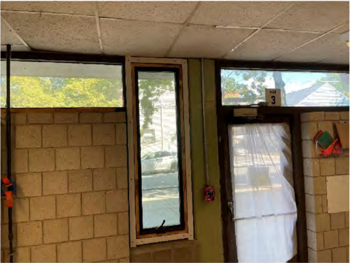
AE-35: Interior of typical newer operable casement window installed as part of COVID-19 pandemic.
