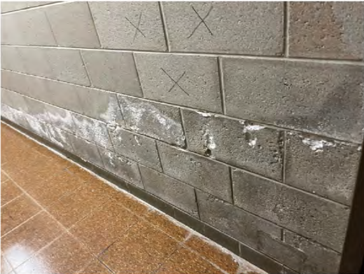
AE-62: Interior of hallway adjacent to Auditorium where efflorescence is present due to active water leakage.
