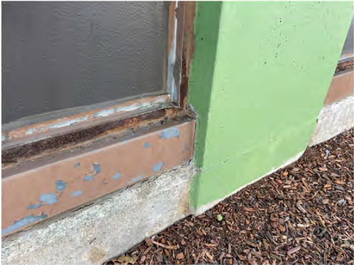
AE-31: Exterior of typical steel framed window with glass lites and metal spandrel panels. Note rusting of framing throughout.
