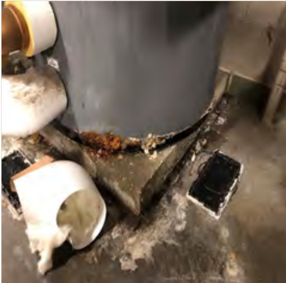
PL-1: Failed Hot Water Tank
