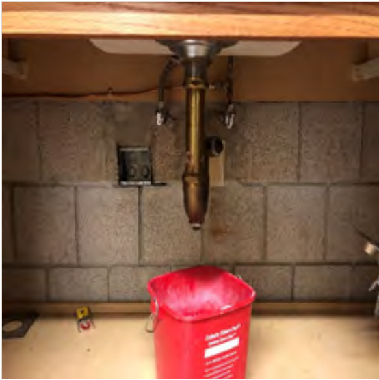
PL-6: Failed P-Trap at Teachers Room Sink
