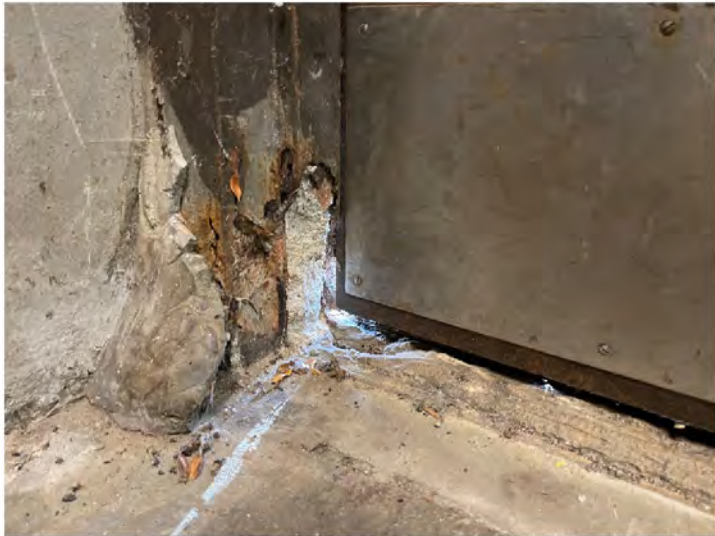
AE-42: Interior at base of typical metal door frame. Note rusting of frame has created a gap at base of door.
