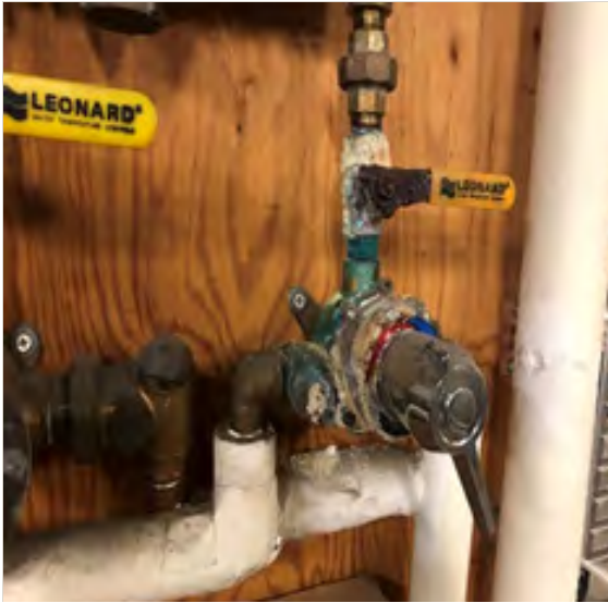
PL-2: Corroded Mixing Valve
