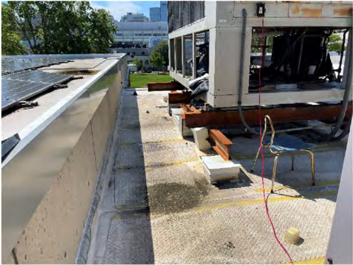
AE-55: Representative MEP unit on dunnage
