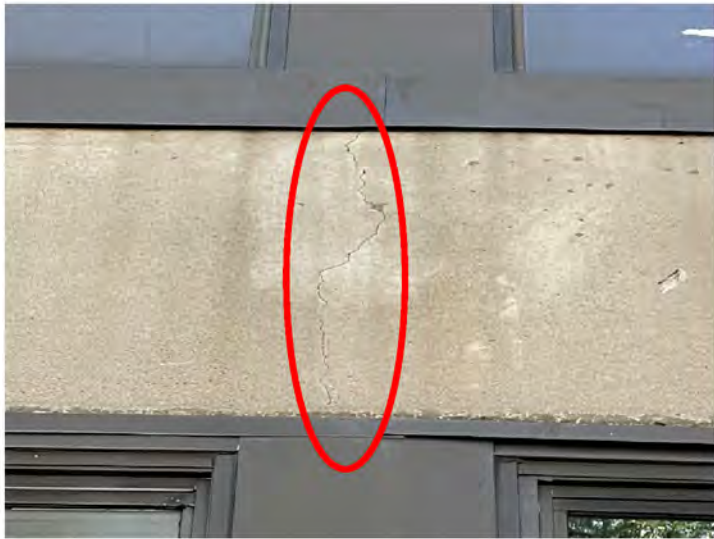
AE-11: Representative vertical cracking at exposed concrete between floors. Condition observed in many locations throughout building.
