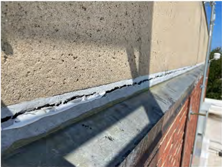
AE-15: Typical failed sealant along top of metal flashing located on top of brick masonry façade.
