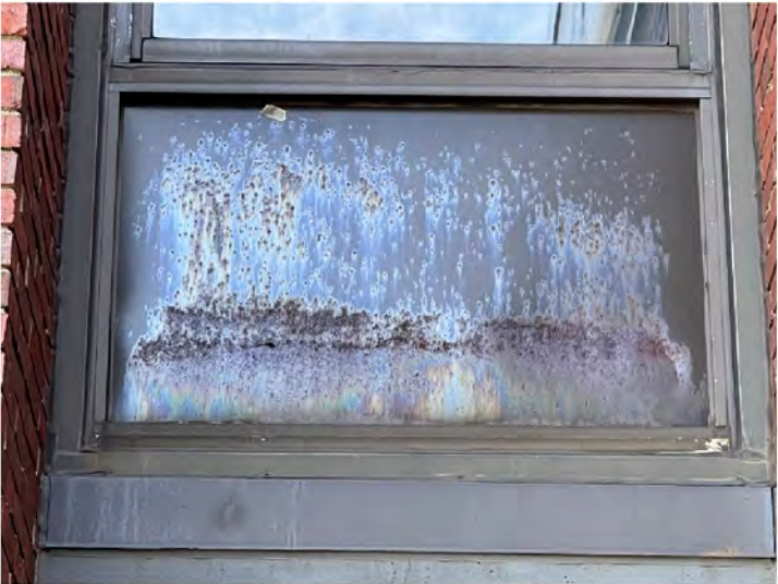
AE-25: Typical metal spandrel panel below typical aluminum window assembly. Not corrosion of panel, typical in many locations.
