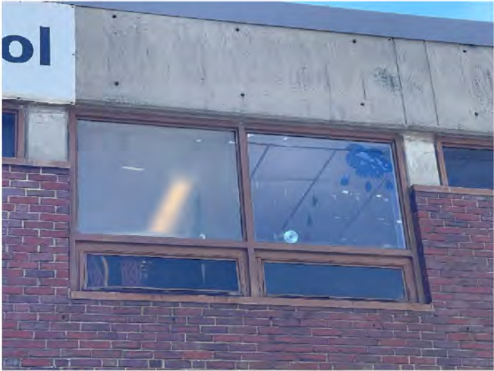
AE-23: Representative steel framed windows with fixed and operable vents, rusting observed on frame.
