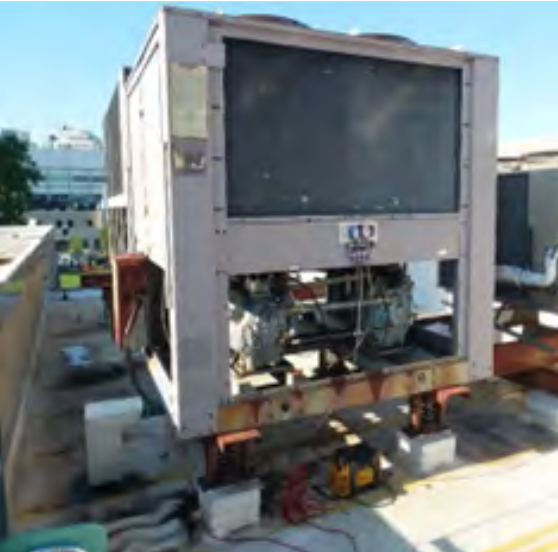
M-3: 2005 Existing Condensing Unit Under Repair
