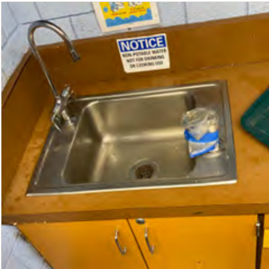
PL-5: Typical Classroom Sink Condition
