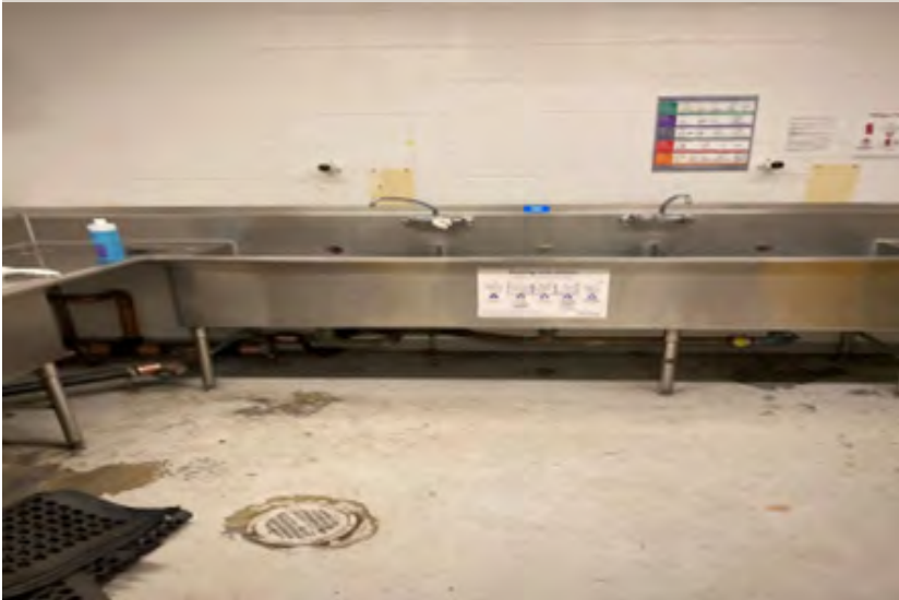
FS-2: Sealed concrete flooring is in poor condition. The seal on the floor is worn and damaged in many locations. The prevent the kitchen floor from being properly cleaned and sanitized.
