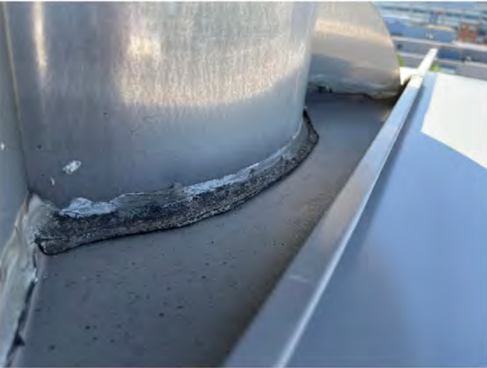
AE-60: Failing sealant at flue penetration in chimney cap
