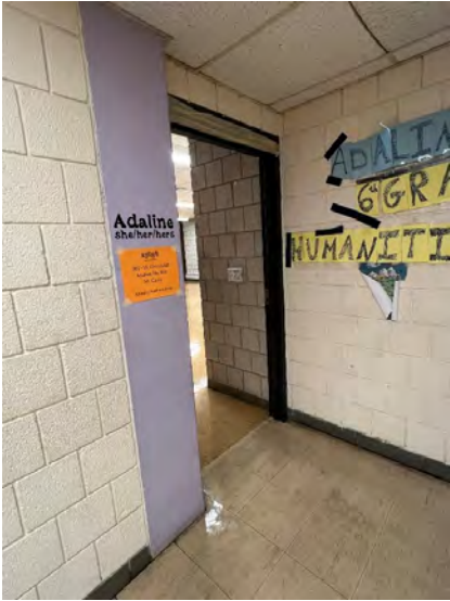
Third Floor- Worn out Flooring
