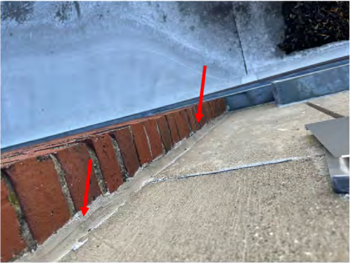
AE-19: Typical sealant at intersection of concrete and brick façade elements, nearing the end of its expected service life.
