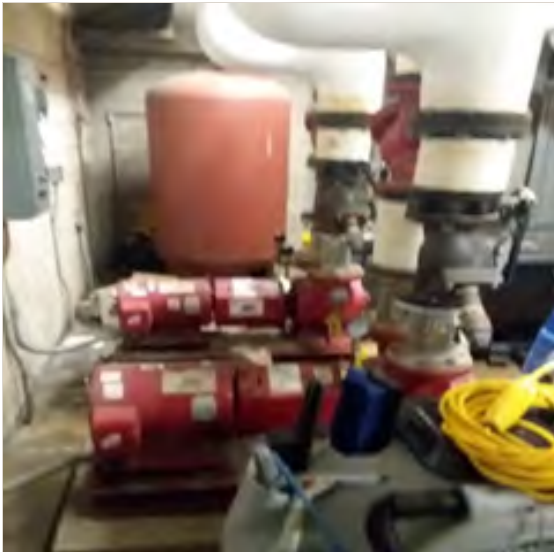
M-2: Existing hot water pumps
