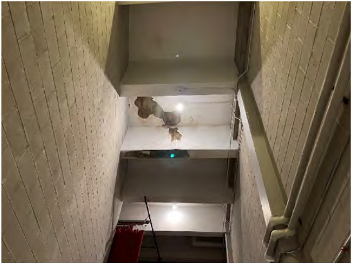
AE-61: View of ceiling above active leakage location at hallway adjacent to Auditorium.
