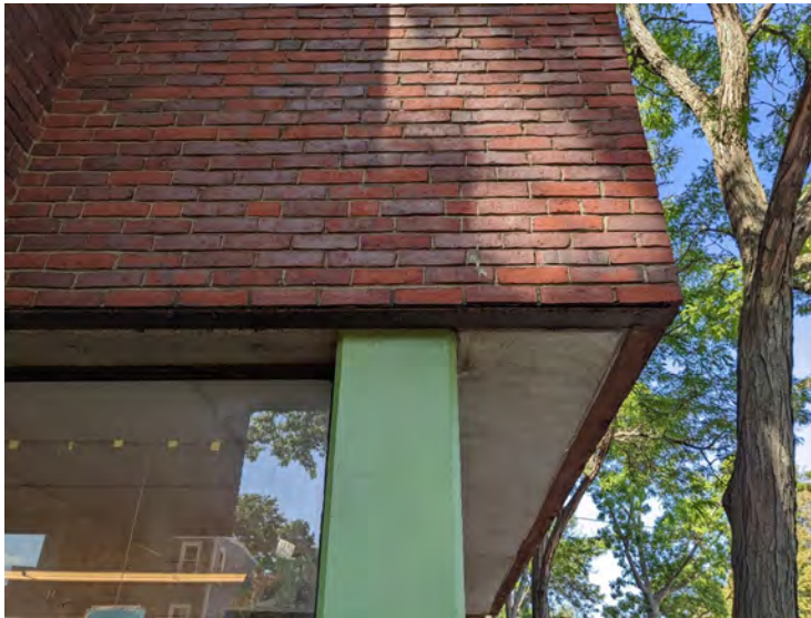
Photo ST-1: Brick Joints and Rusted Lintels
