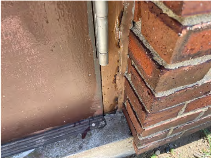
AE-39: Typical failed perimeter sealant at typical exterior door
