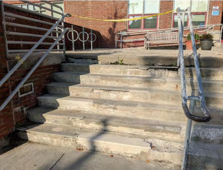
Photo ST-1: Spalling Concrete at Site Stair
