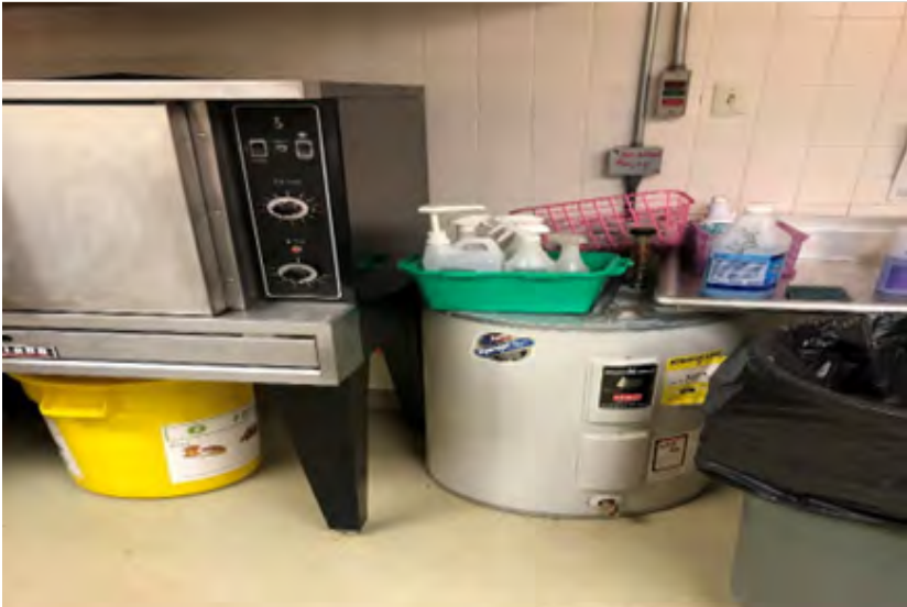
FS-4: There is a water heater located within the kitchen in between cooking and pot washing equipment. Normally this type of equipment is located remotely in a mechanical closet. With the location this equipment is in, it’s difficult to clean, and ends up being used to store items that do not belong. This location presents issues with cleanability of the kitchen and damage to the water heater itself. This equipment should be relocated out of the kitchen space.
