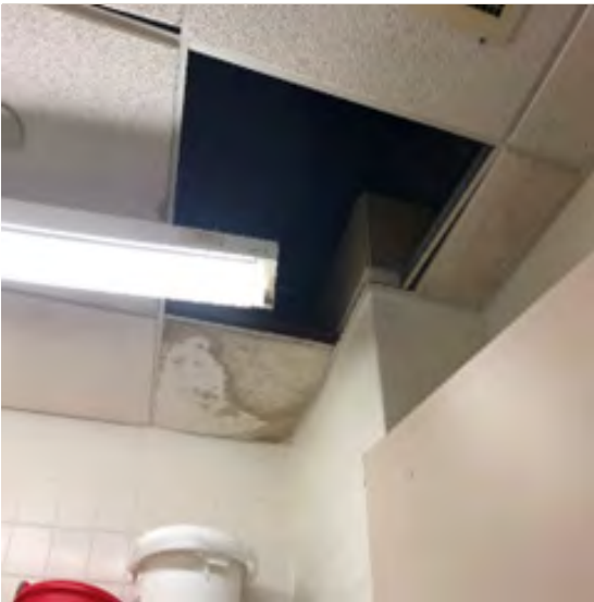
FP-1: Ceiling Tile shall be replaced
