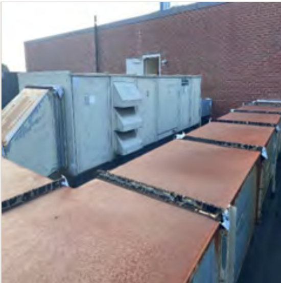
M-5: Rooftop Air Handling Unit and Ductwork
