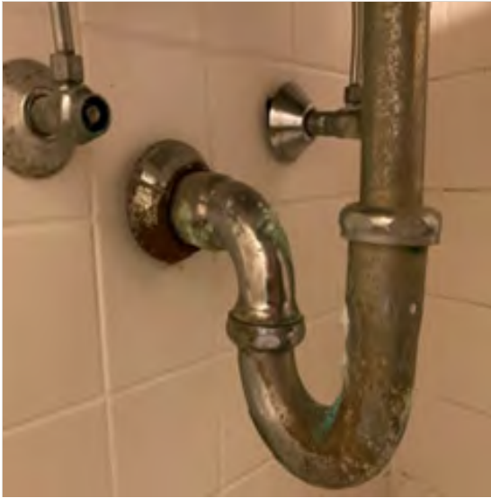
PL-3: Corroded Lavatory Piping
