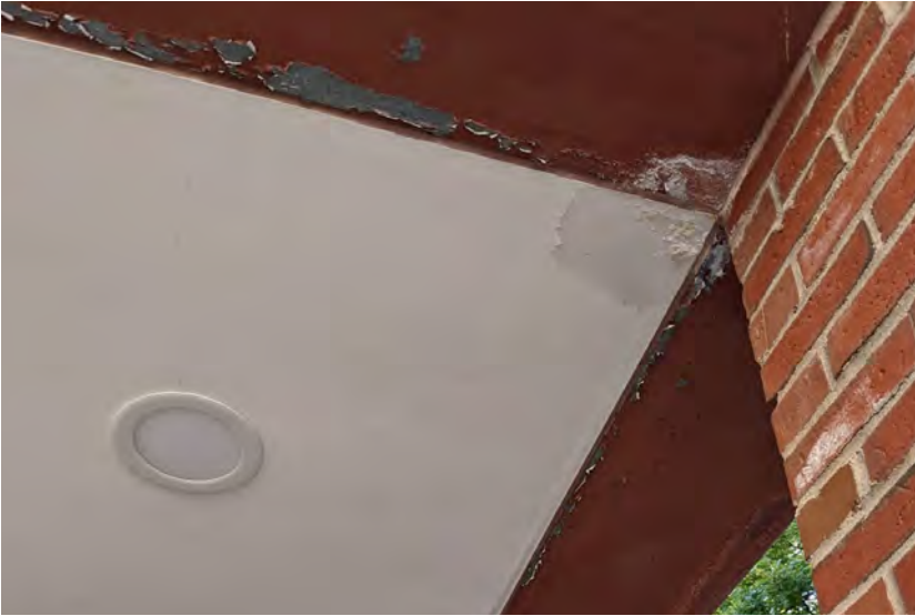
Photo ST-8: Peeling Paint at Exterior Soffit
