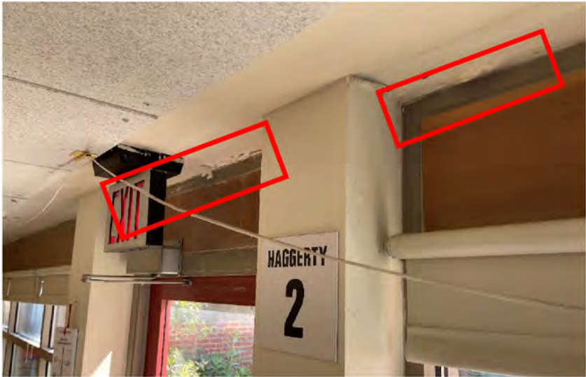
AE-14: Interior of typical classroom at West Wing, East classrooms below Main Entry: Water leakage, drywall damage and peeling paint at interior side of relieving angles and adjacent drywall, storefront spandrel panels.
