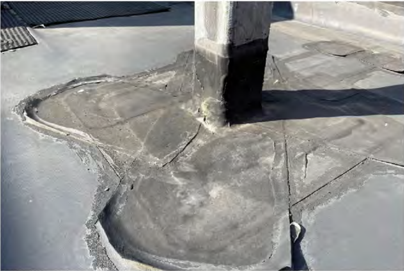
AE-41: Typical EPDM patch with failed lap sealants that has become unadhered
