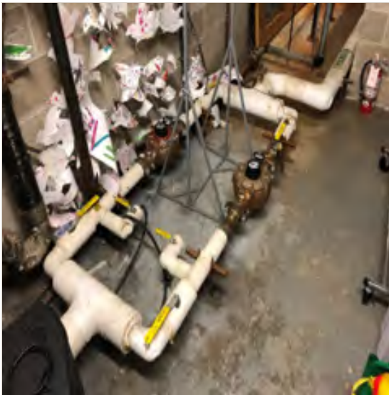
PL-1: Water Service Entrance
