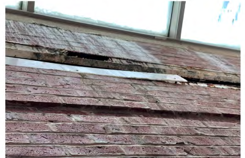
AE-32: Interior of Corridor below Sloped glazing at transition between Main Building and West Wing: Typical area of active water leakage, note staining and efflorescence on brick masonry.
