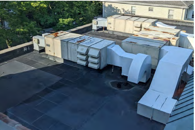
Photo ST-4: Ponding Water
