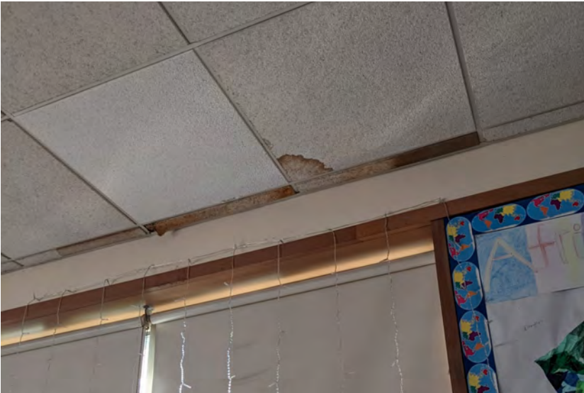
Photo ST-6: Water-Stained Ceiling Tiles
