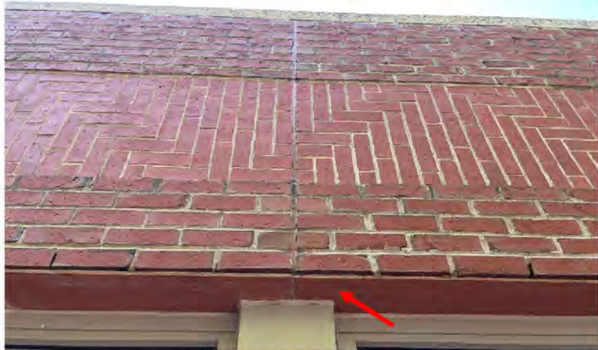
AE-12: Representative brick masonry façade along West Wing: Less efflorescence observed in this area. Note relieving angle is continuous from exterior to interior at head of all storefront
