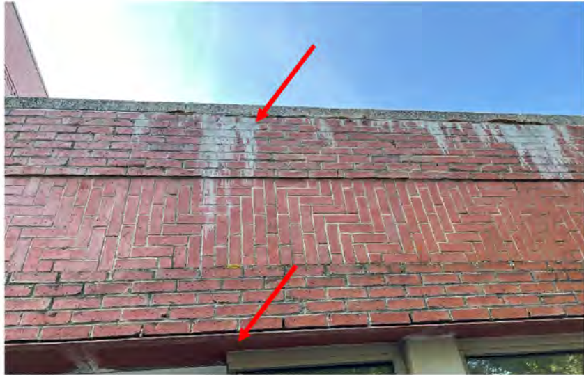
AE-10: West Wing: Conditions typical throughout West Wing and East classrooms below Main Entry. Typical efflorescence on masonry due to excess moisture, note relieving angle is exposed at head of storefront, continues from exterior to interior
