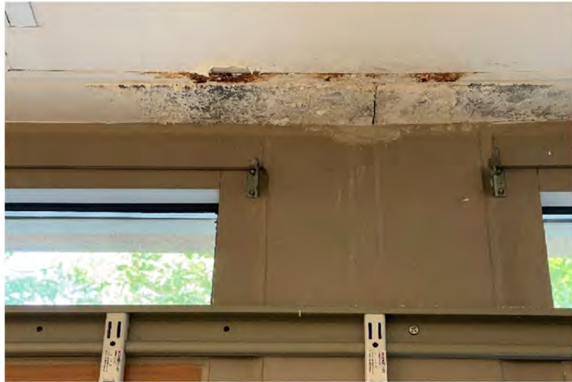
AE-13: Interior of typical classroom at West Wing, East classrooms below Main Entry: Similar conditions observed in all of these classrooms. Water leakage, rusting and peeling paint at interior side of relieving angles.
