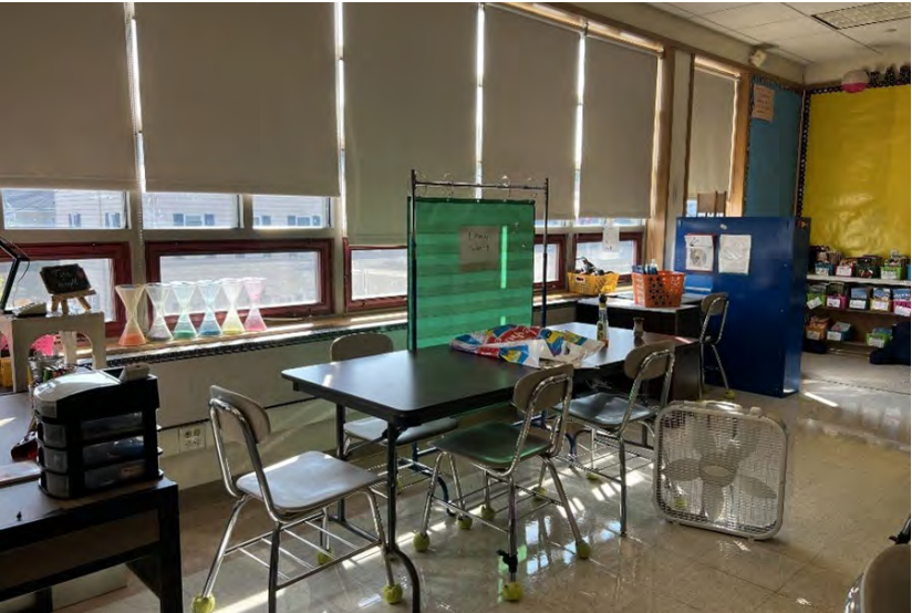
Third Floor Classroom (mold possible)
