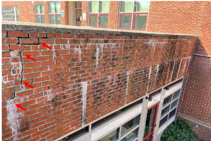
AE-11: Representative East Classrooms below Main Entry: Conditions typical throughout West Wing and East classrooms: Efflorescence, cracked and displaced brick
