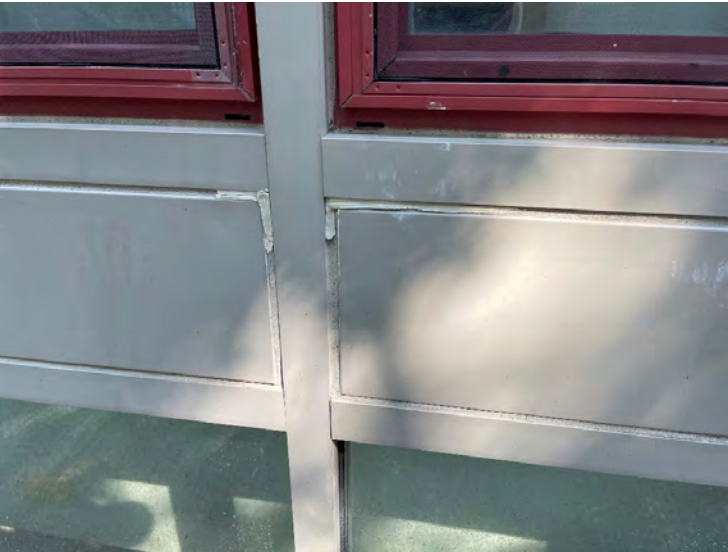
AE-C: Typical storefront spandrel panels with added sealants
