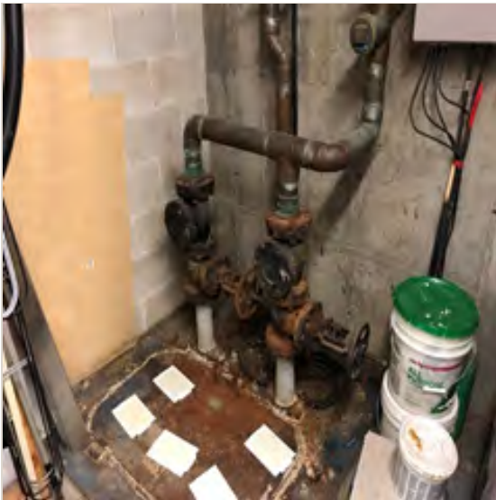
PL-5: Existing Sewage Ejector
