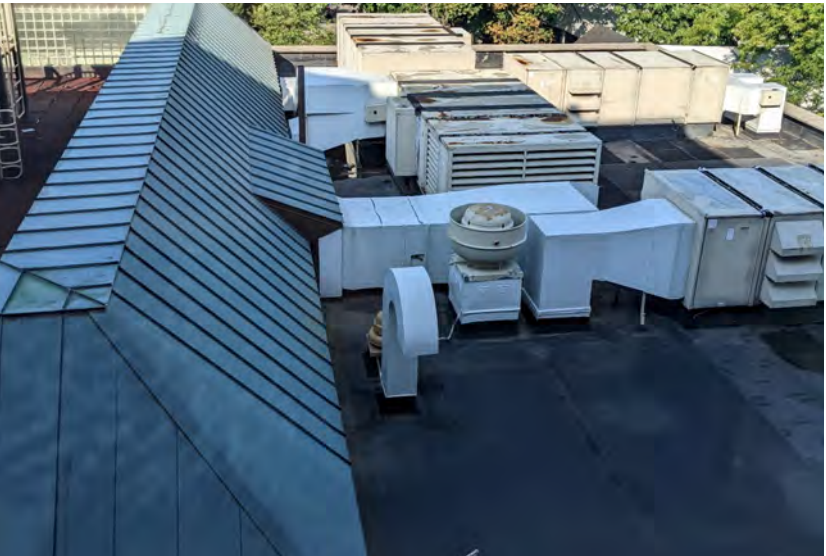
Photo ST-5: Ponding Water
