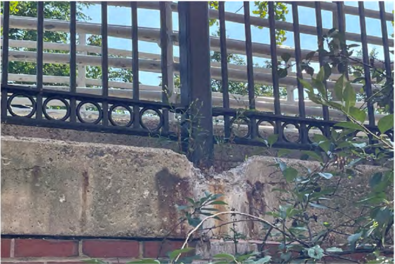
AE-46: Typical spalling concrete at retaining wall around East side of building
