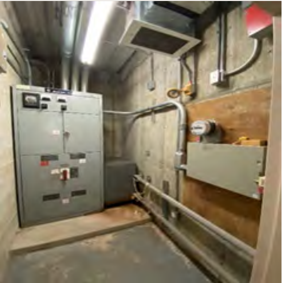
E-1: Main Electrical Service (Entrance)
