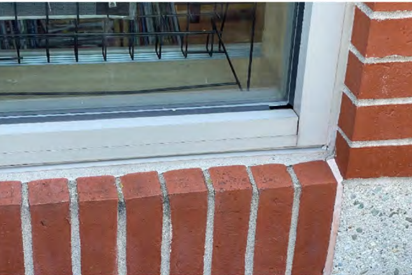
AE-15: Representative brick masonry façade at perimeter of window: Note perimeter sealants and masonry control joint sealants are reaching the end of their service lives.
