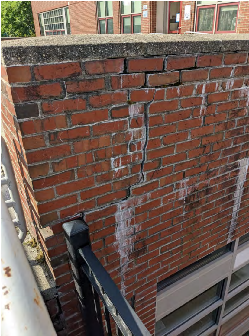
Photo ST-3: Cracked Masonry at Site Wall
