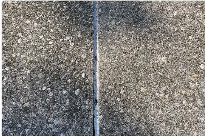
AE-9: Representative precast concrete coping cap at West Wing. Note failed sealants between caps.
