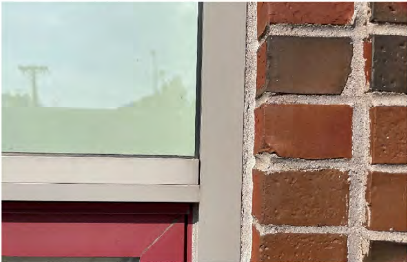
AE-16: Representative brick masonry façade at perimeter of window: Note perimeter sealants and masonry control joint sealants are reaching the end of their service lives.
