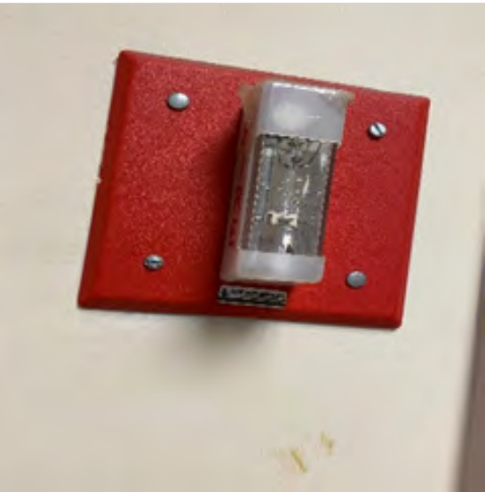
E-7: Existing Fire Alarm Device (1993)
