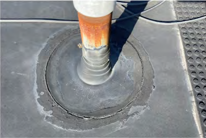
AE-43: Typical prefabricated EPDM flashing boot with failed lap sealant at perimeter. Note perimeter of boot is starting to become unadhered.
