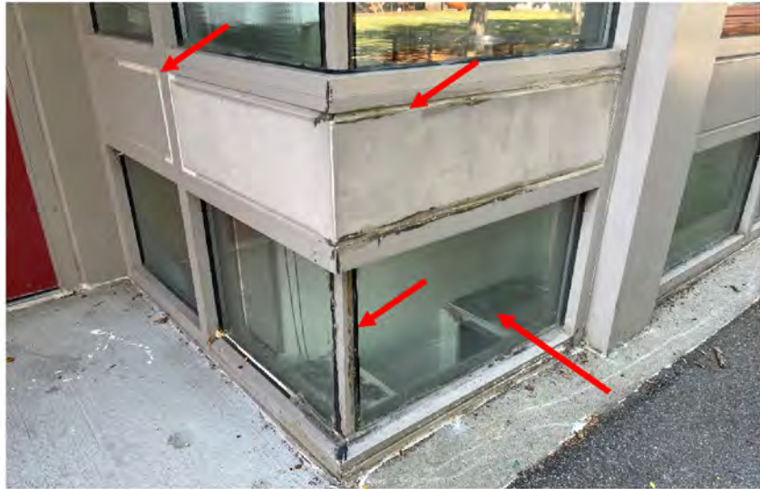
AE-26: West Wing and East classrooms below Main Entrance: Typical storefront near classroom entry door. Note added sealants at glass and spandrel panels, missing drywall due to leakage in Cafeteria below.
