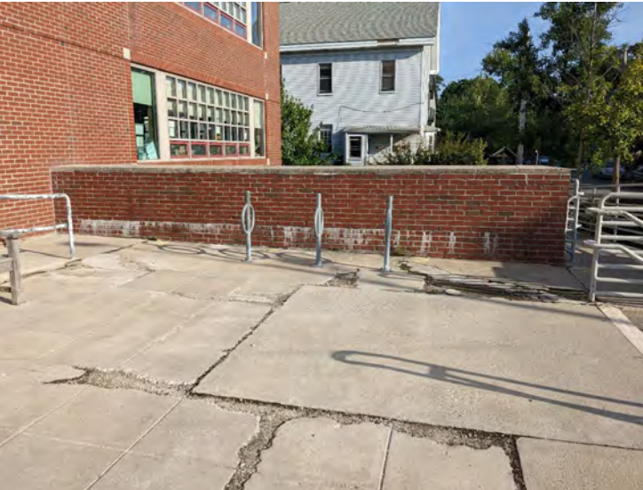
Photo ST-2: Deteriorating Site Paving
