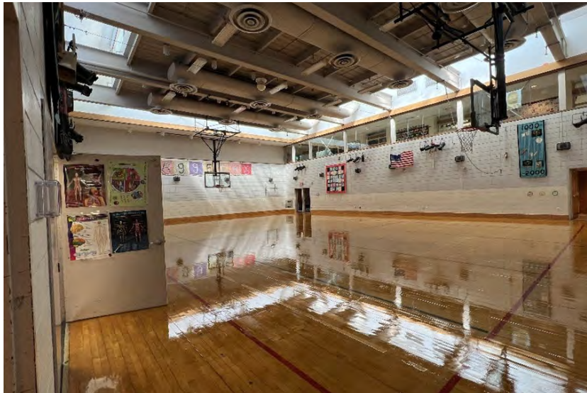
Gym (Wood floor gaps)
