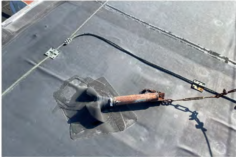
AE-44: Damaged guyline anchor post at flue: Note failed EPDM flashings around anchor.
