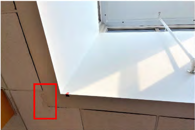
AE-23: Interior of clerestory at Library/Media Center: Typical water leakage staining observed on ceiling surrounding clerestory
