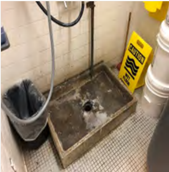
PL-2: Corroded Janitors Sink
