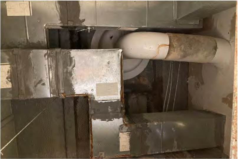
AE-48: Interior of ceiling in Room 109, below roof drain where leakage occurs
