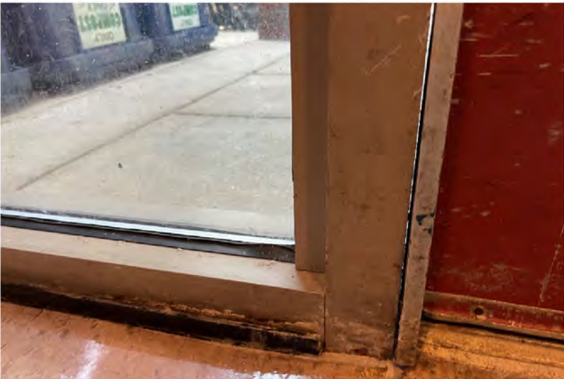
AE-35: Representative daylight visible between door and storefront framing at West Wing: Some corrosion on base of storefront door frame.
