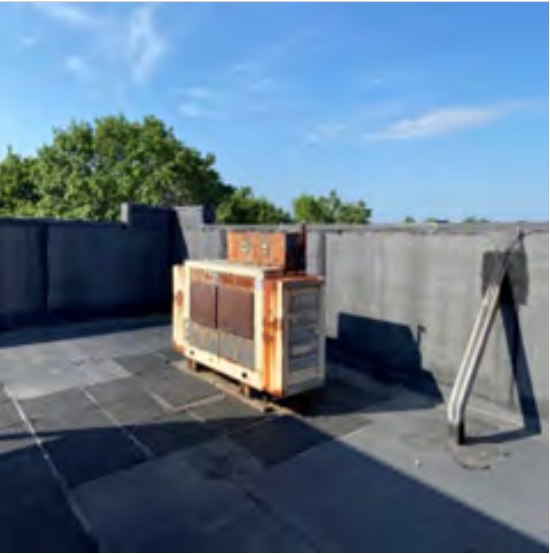
E-2: Standby Generator System
