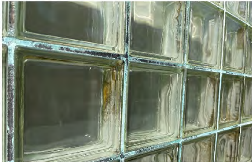
AE-20: Typical water drip staining within mortar joints between glass block, condensation within block itself. Condition typical throughout most of these facades .
