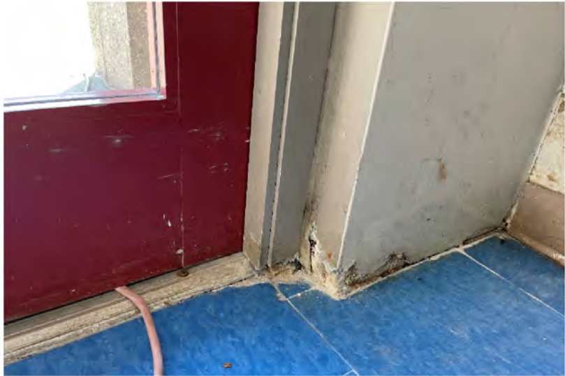
AE-34: Representative drywall damage due to moisture adjacent to Main Entry doors
