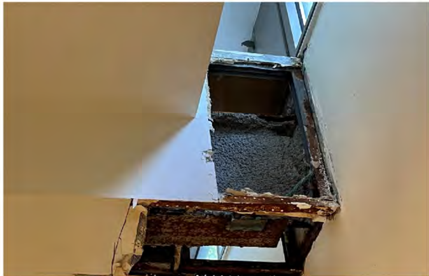
AE-28: Typical removed drywall, rusting beams and soffit framing due to active water leakage from storefront and storefront perimeter above
