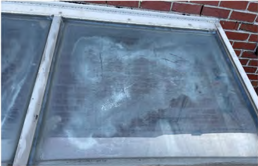
AE-30: Sloped glazing at transition between Main Building and West Wing, located above interior corridor: Typical failed IGU, as evidenced by condensation between panes of glass.
