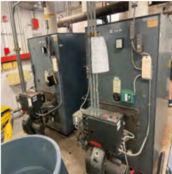
M-1: Original Cast-Iron Boilers
