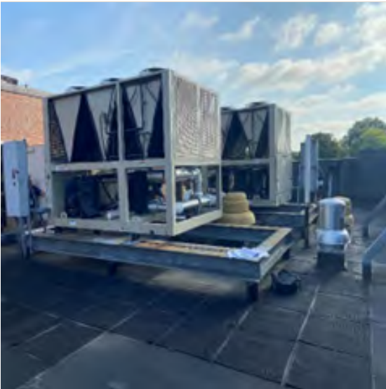
M-4: Upgraded Air-cooled Chillers
