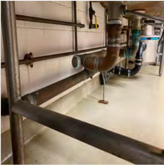
PL-6: Corroded Waste Pipe at Pot Sink
