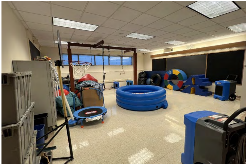
Sensory Room - Basement (Water Damage)
