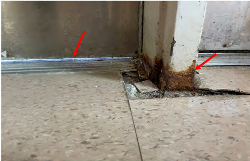
AE-33: Interior of typical exterior door: Typical rusting at base of door frame, daylight visible below door at deficient weatherstripping.
