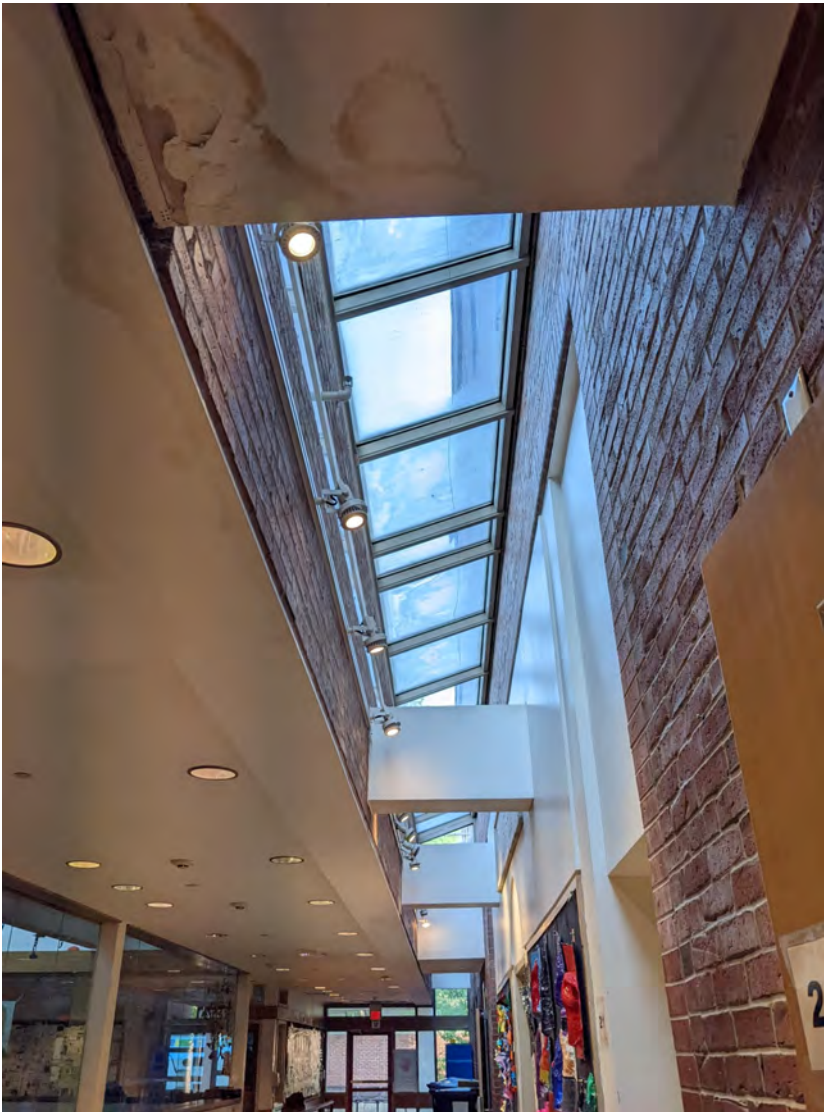
Photo ST-7: Evidence of Water Infiltration in Ceiling Finishes
