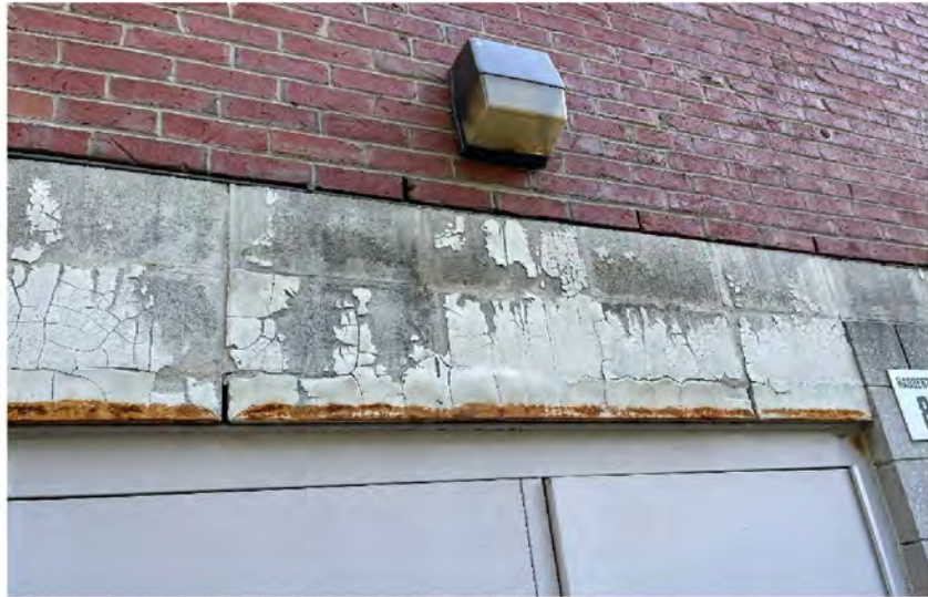
AE-18: West Elevation: Typical failed coating on CMU
