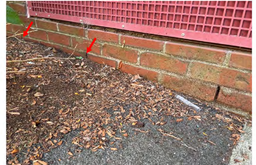
AE-7: North Elevation: Masonry weeps partially covered with mulch
