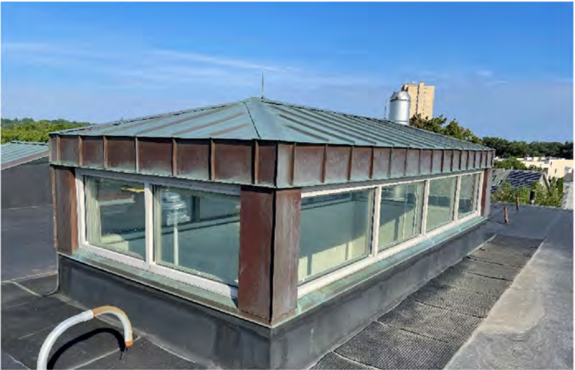
AE-21: Clerestory above Media Center / Library: Storefront here have misc. sealants at perimeter and on glazing.
