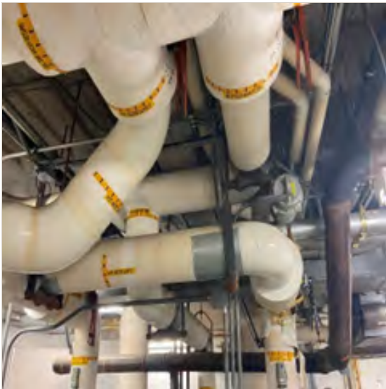
M-3: Original Dual Temperature Piping and Valving
