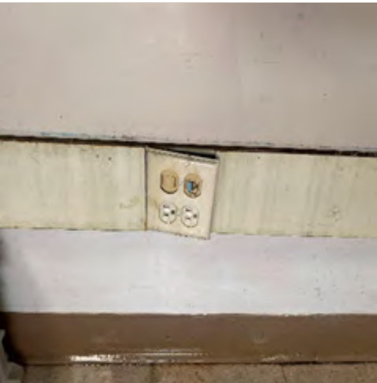
E-3: Existing Devices
