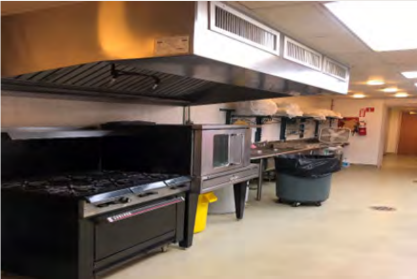
FS-3: Exhaust hood over the cooking equipment is extremely dated and original to the building. The grease filters are not nearly as efficient as the technology that’s available today and are more difficult to clean. The horizontal cast piping used for fire suppression is very difficult to keep clean. Efficient Design limits fire suppression to vertical drops only.
