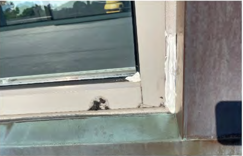
AE-22: Clerestory at Library/Media Center: Typical added sealants at perimeter and glazing of storefront units.
