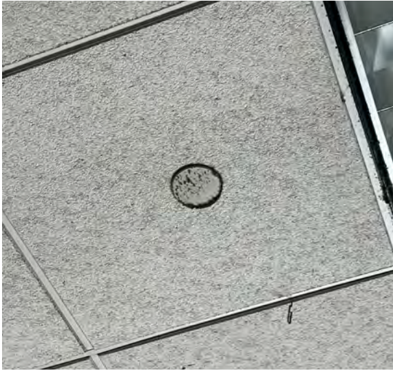
Mold on sprinkler
