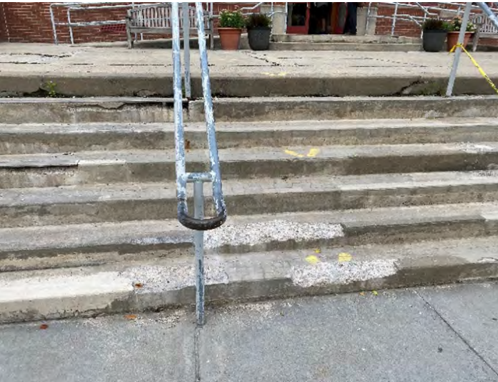
Deteriorated Front Steps
