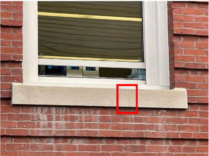
AE-16: Representative cracking limestone at South Elevation
