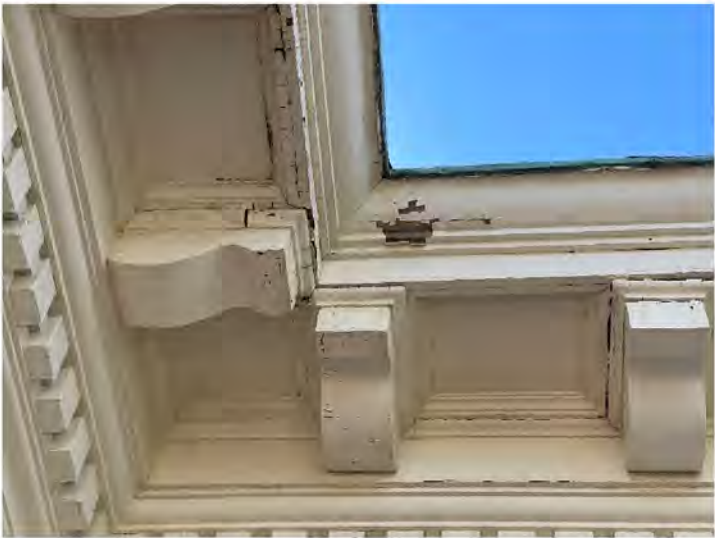
AE-39: Typical peeling paint on wood cornice surrounding South roof
