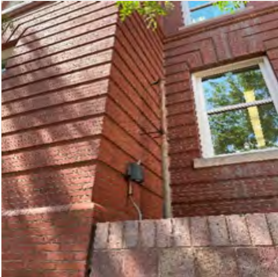
E-2: Generator Exhaust
