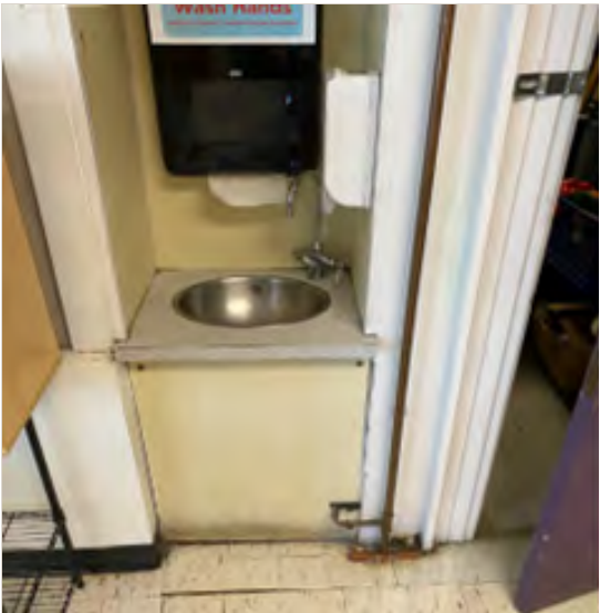
PL-1: Exposed uninsulated cold water at classroom sinks
