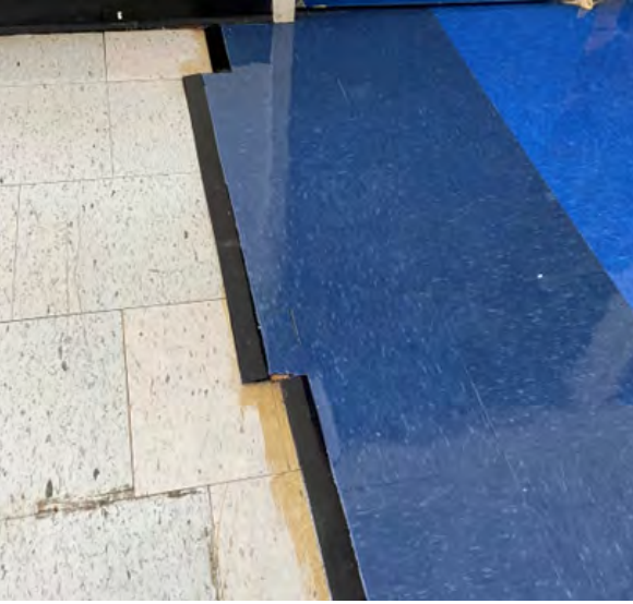
Photo ST-4: Added Floor Tiles at Differential Floor Elevations in Classroom
