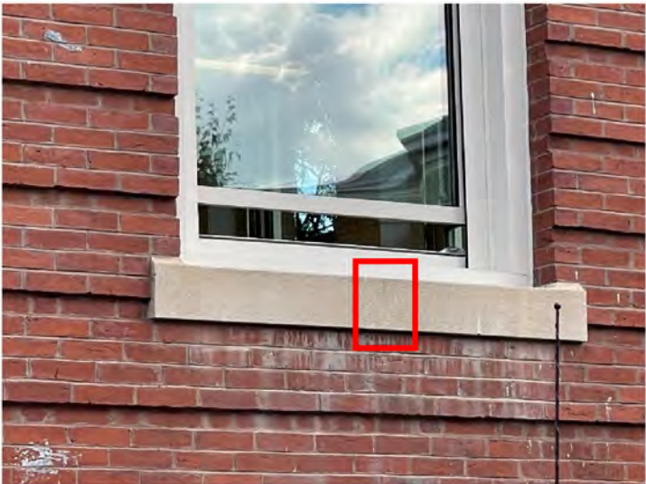
AE-15: Representative cracking limestone at South Elevation
