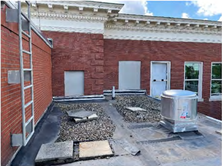
AE-29: Mid-level roof at West side of North wing. Ballast has been moved around, exposing loose laid EPDM.
