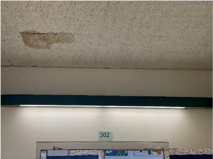
AE-47: Stained ceiling tiles due to roof leakage within Corridor outside Room 302
