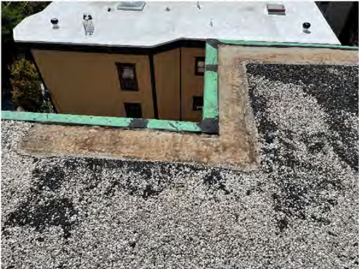
AE-37: Typical tar and gravel repairs along roof edge at South roof
