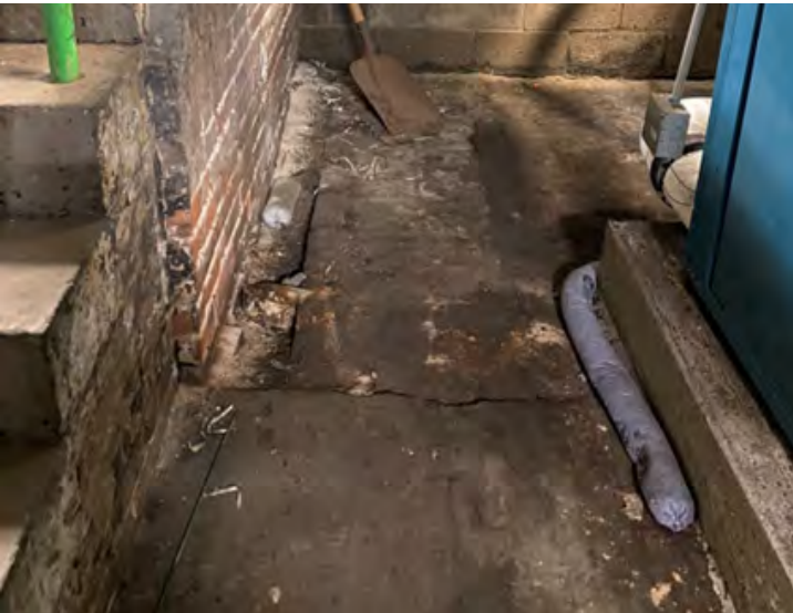
Photo ST-1: Cracks and Moisture in the Slab on Grade at the Mechanical Basement
