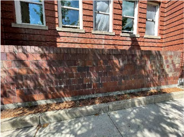
AE-45: Masonry screen wall on East Elevation. Some crazing and efflorescence observed within masonry.
