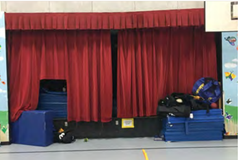
Main Curtain with Damage
