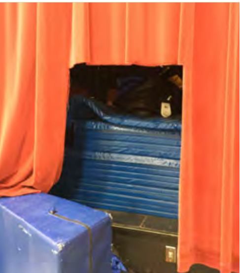
Detail of Curtain Damage
