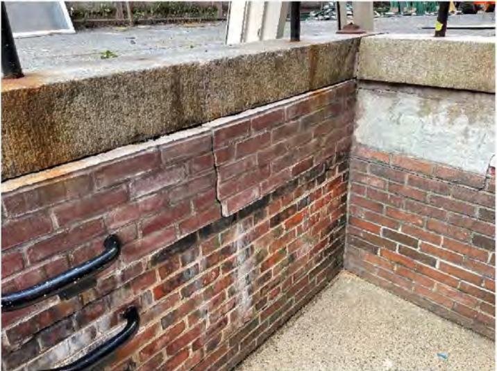
AE-44: Representative displaced and cracked brick at lower level building entrance on West Elevation
