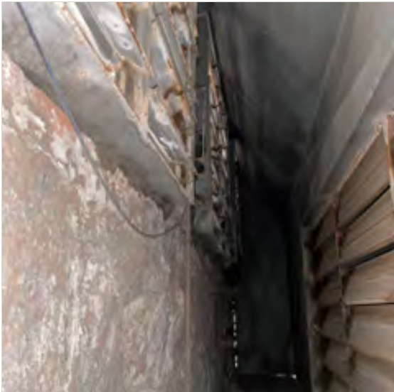
M-4: Corroded H&V Dampers
