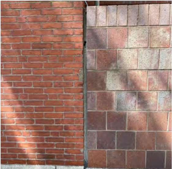
Photo ST-5: Deteriorated Caulking at Exterior
