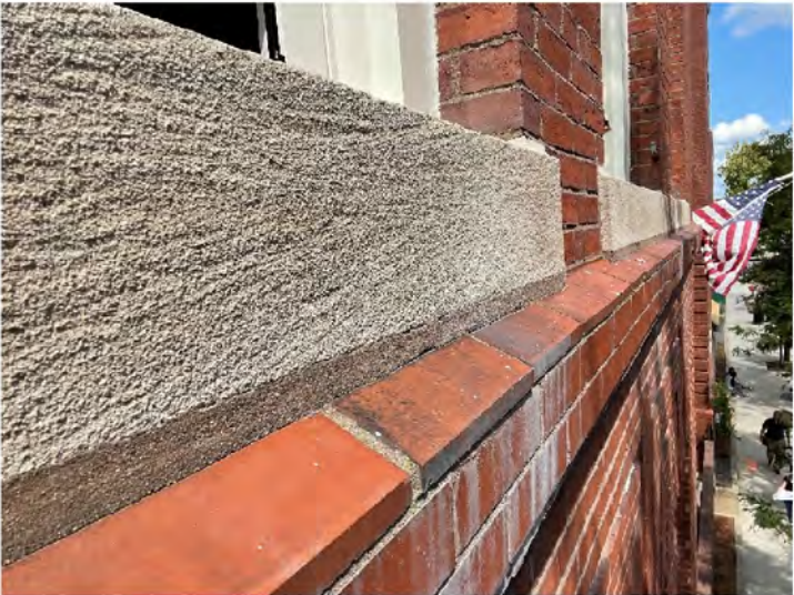
AE-14: Façade condition above bulge in masonry that has been repointed at East Elevation
