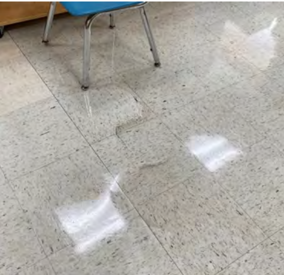
Photo ST-2: Uneven Floor at OT/PT Room
