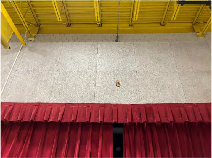
AE-49: North elevation within Gymnasium where leakage occurs at Stage
