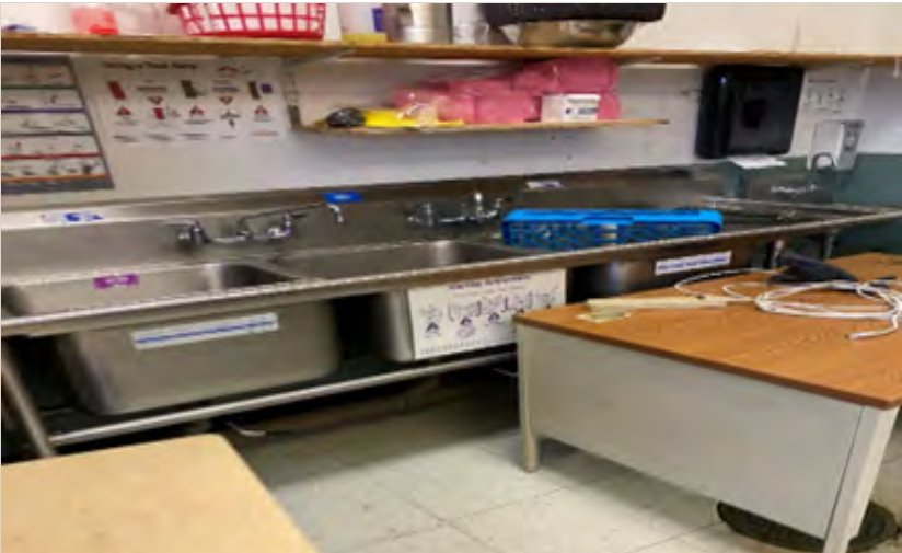
FS-4: Wood wall shelving is present as storage at the pot washing sink. Wood is not an acceptable storage material for storage especially in a wet area. NSF rated shelving systems must be used throughout commercial kitchens.
