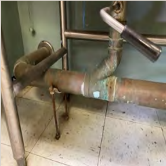
PL-5: Corroded Copper Waste Pipe
