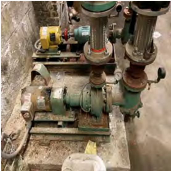
M-2: Hot Water Pumps
