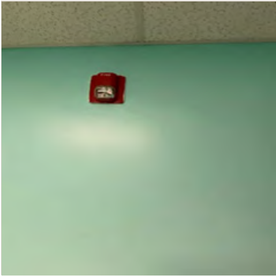
E-5: Existing Fire Alarm Device
