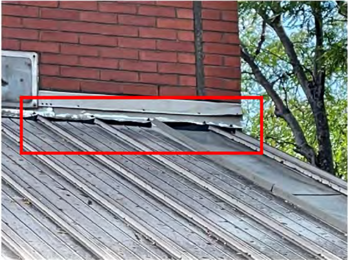
AE-41: Termination of metal roofing at masonry façade on North Elevation. Daylight and drip staining visible on interior in this area.
