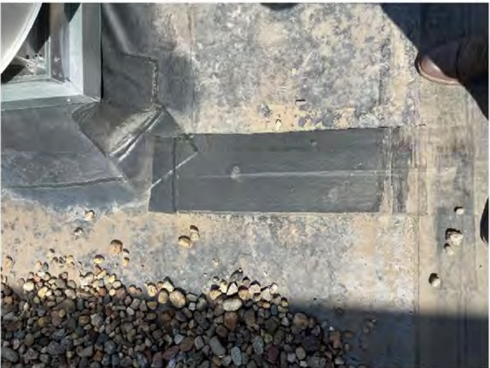
AE-32: Typical EPDM patches at Gymnasium roof, lacking lap sealant termination at perimeter.
