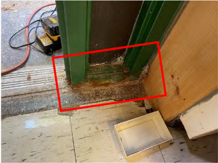
AE-25: Interior of typical hollow metal door assembly. Note rusting on base of frame.
