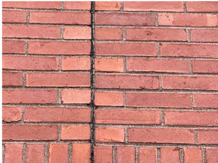
AE-19: Representative failed control joint sealant at masonry façade at North wing addition
