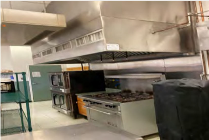
FS-2: Exhaust hood over the cooking equipment is extremely dated and original to the building. The grease filters are not nearly as efficient as the technology that’s available today and are more difficult to clean. There are several locations where utilities penetrate the hood which is not acceptable.
