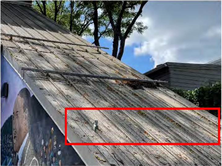
AE-42: Missing snow rail at metal roofing on North Elevation
