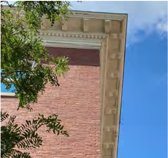
Photo ST-6: Deteriorated Roof Edge Fascia
