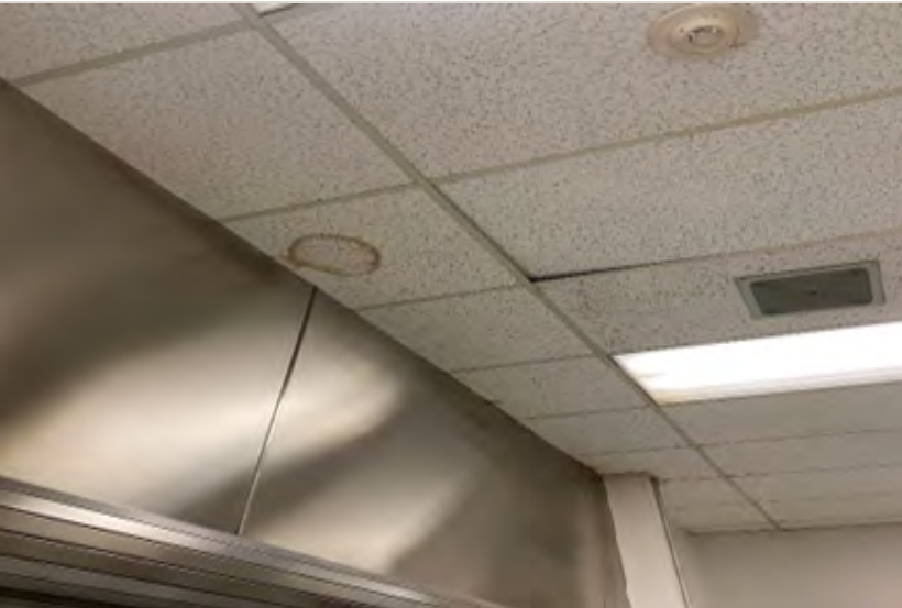
FS-1: The ceiling material in the kitchen space is not a smooth washable surface and shows significant signs of wear and tear and water damage. Ceilings for this kitchen should be updated to meet modern day food code
