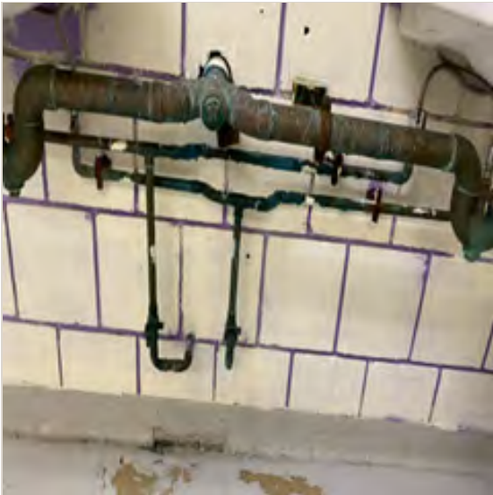
PL-6: Corroded Copper Domestic & Waste Pipe
