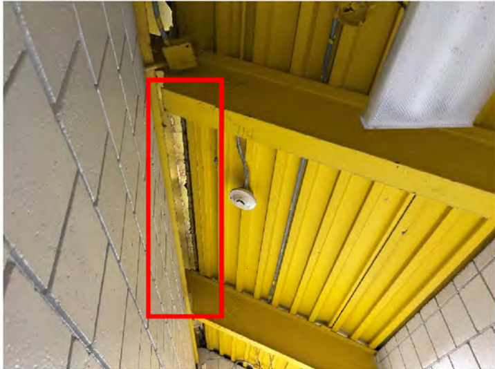
AE-52: Interior view at intersection of metal roofing and masonry façade within Stage area at Gymnasium. Daylight visible between these assemblies.
