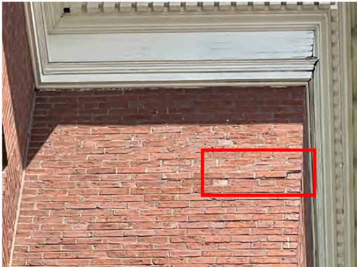
AE-10: Displaced masonry at East Elevation, South return
