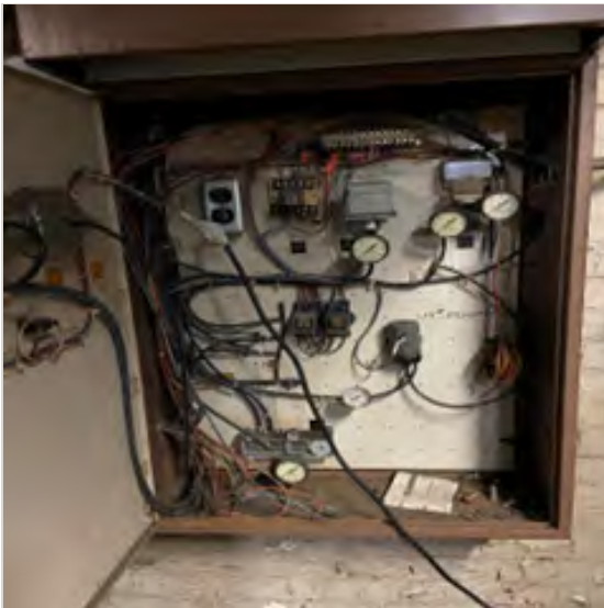
M-5: Pneumatic Control Panel
