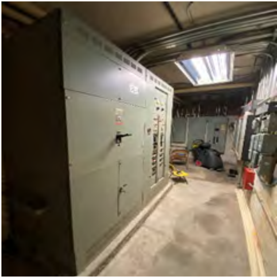
E-1: Main Electrical Service (Entrance)
