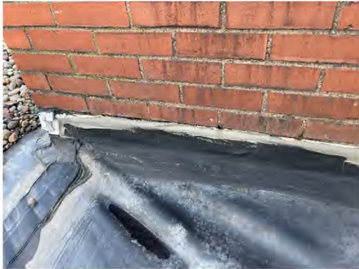
AE-33: Typical EPDM termination to base of masonry façade on Gymnasium roof with only sealant.
