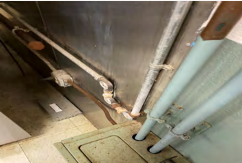
FS-3: Exposed utilities along the cook line building wall present cleanability issues and potential violations of the health code if not properly cleaned. Utilities should be provided within a furred-out wall in these circumstances for proper cleanability.
