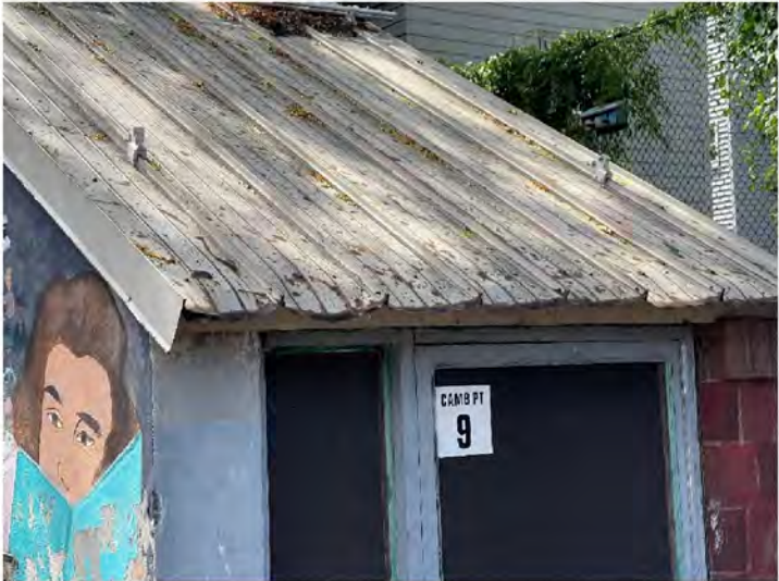
AE-43: Damaged metal roofing at eave of North Elevation entrance.
