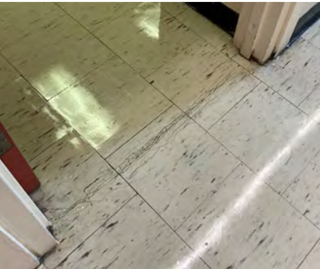
Photo ST-3: Cracks in Floor Tiles at Upper Floor
