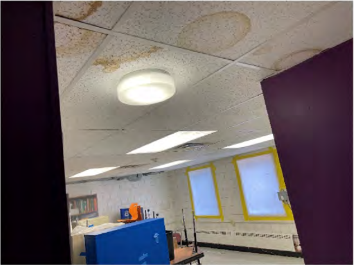
AE-46: Stained ceiling tiles due to roof leakage within Room 301
