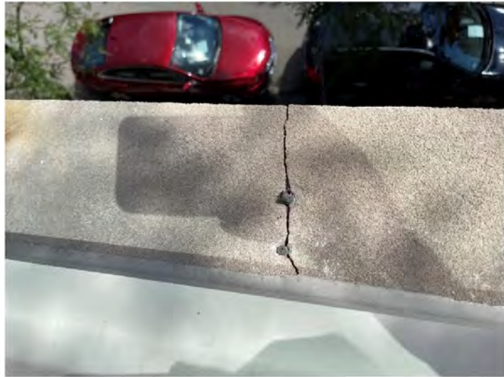
AE-17: Typical cracked limestone as viewed from above at Room 201
