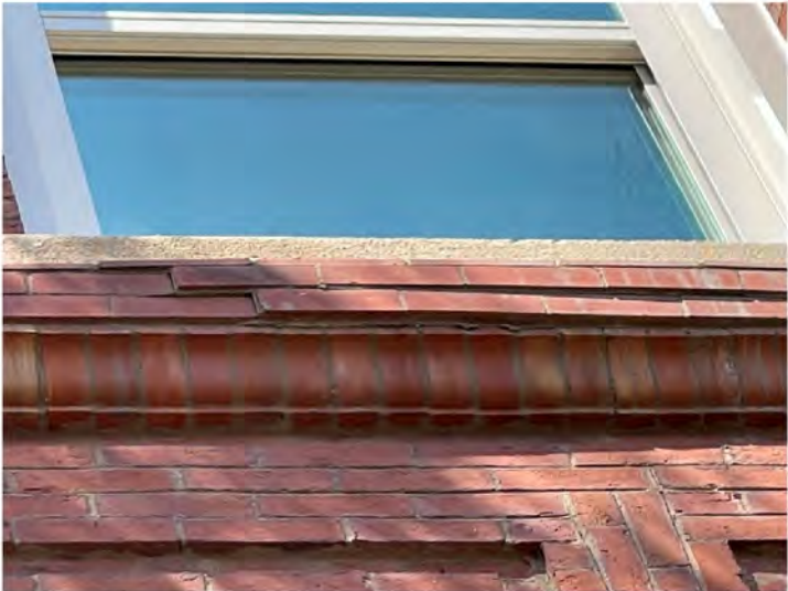
AE-13: Bulge in masonry at East Elevation, has been repointed
