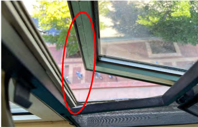
AE-17: Typical broken chain limiter on operable window
