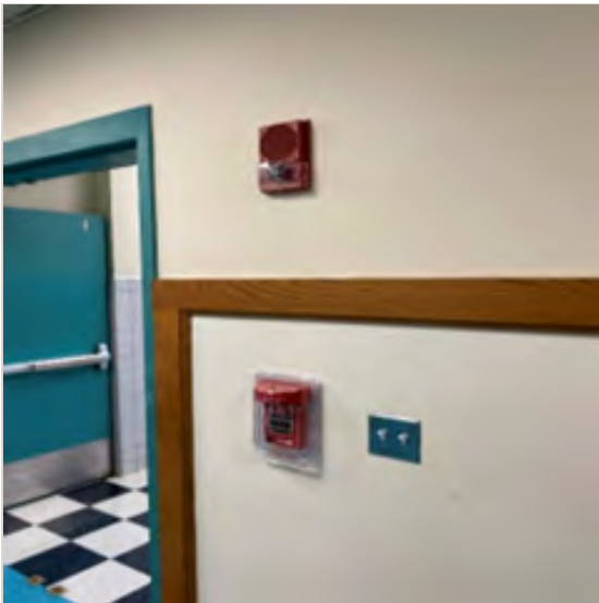
E-5: Existing Fire Alarm Device
