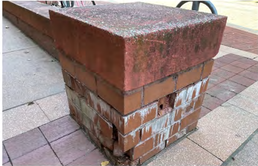
AE-34: Representative masonry walls along ramp at North Elevation. Note spalled brick, efflorescence
