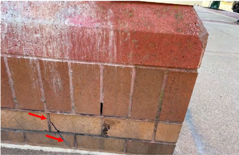
AE-9: Representative brick masonry façade along North Elevation. Typical efflorescence, cracked brick and mortar
