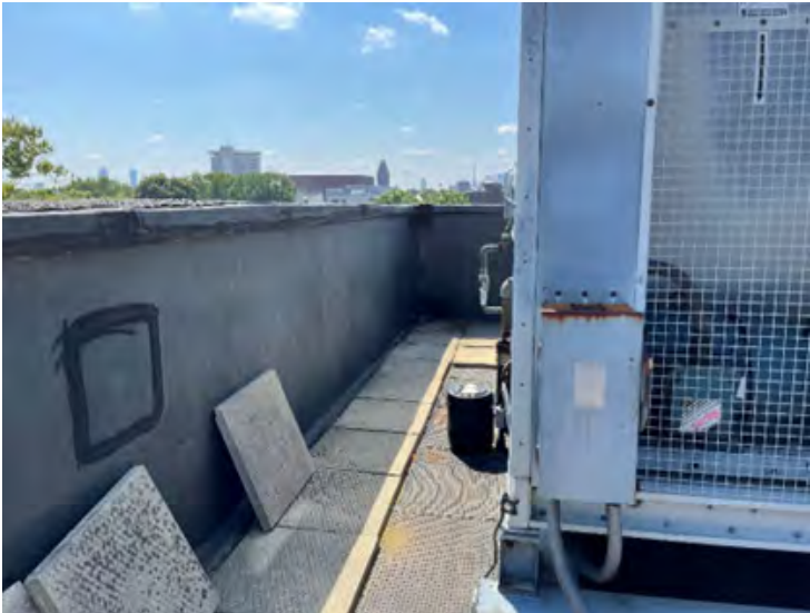
AE-C: Partial view of mechanical well
