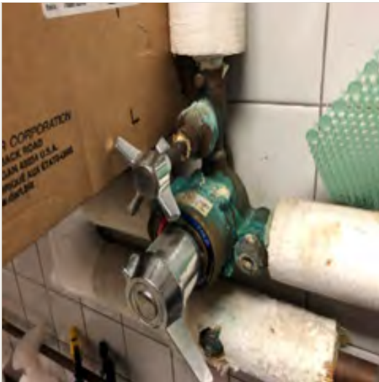
PL-3: Corroded Mixing Valve
