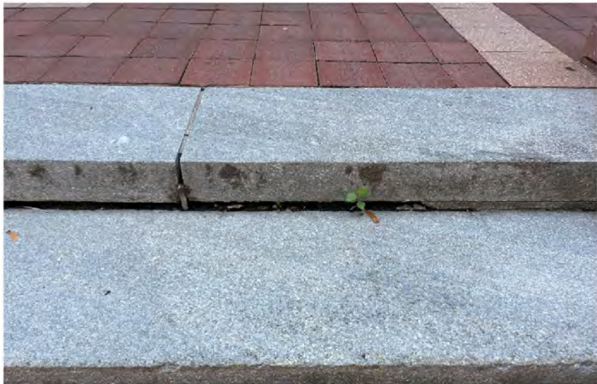
AE-35: Representative Stairs at North Elevation. Typical deteriorated mortar at granite stair treads
