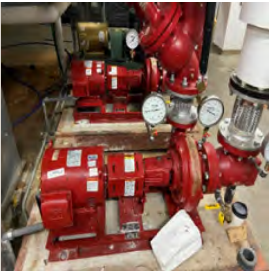
M-2: Existing Hot Water Pumps
