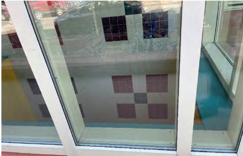
AE-13: Cracked pane of glass at North Elevation
