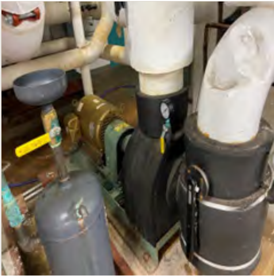
M-4: Original Chilled Water Pump
