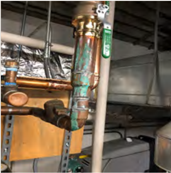
PL-2: Corroded Length of Pipe
