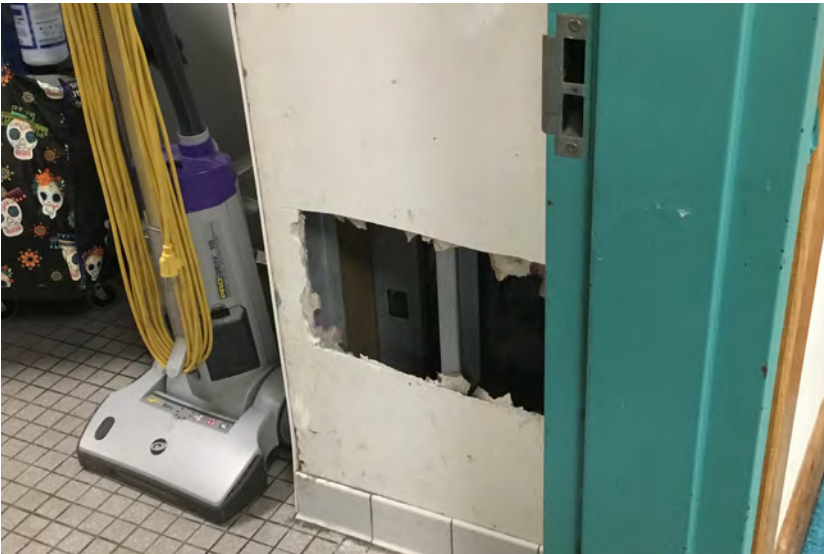
Unpatched hole in wall in Janitor Closet
