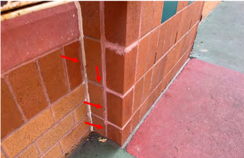
AE-11: Representative cracked mortar at pilasters along base of West Elevation
