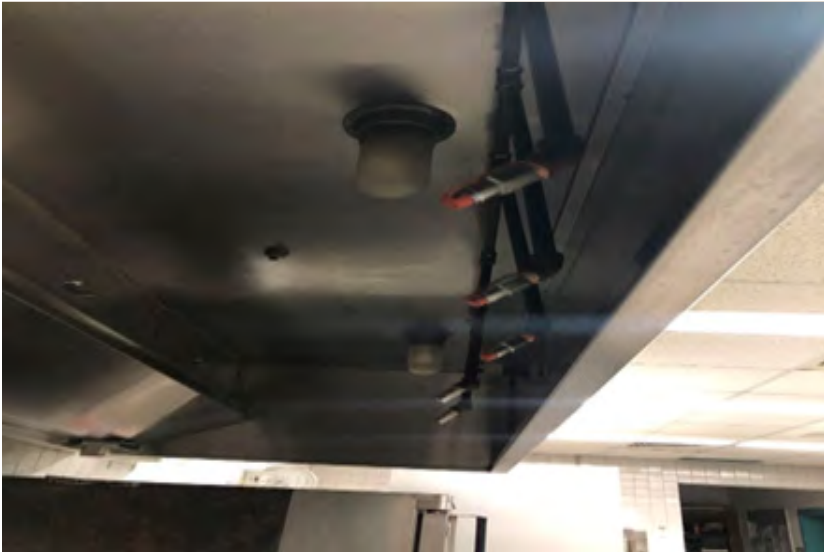
FS-2: The grease filters at the exhaust hood are dated technology and not as efficient as what’s available today. They are also more difficult to clean. The fire suppression piping runs horizontal within the cavity which results in excessive grease build up. Efficient design limits fire suppression to vertical drops only. Iron piping was used for the Ansul system, modern day piping is stainless or chrome for improved cleanability.
