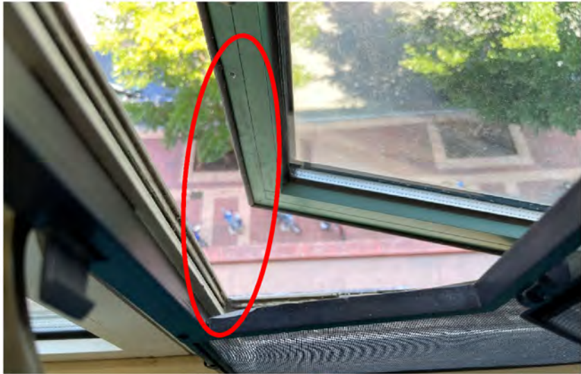
AE-37: Typical broken chain limiter on operable window
