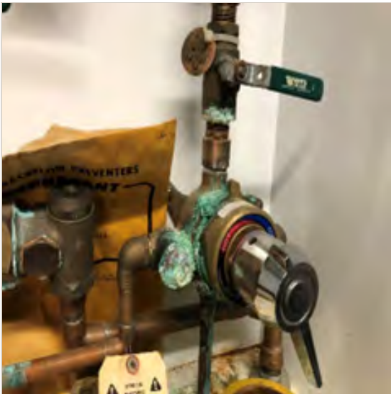
PL-1: Corroded Mixing Valve
