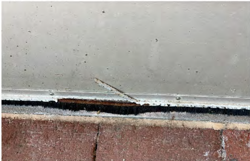
AE-19: Damaged weatherstripping at typical entrance door on East Elevation
