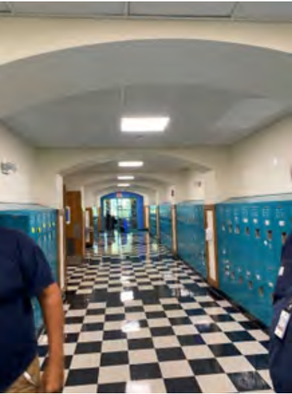
E-4: Typical Corridor (LED Upgrade w/ Emergency Lighting)
