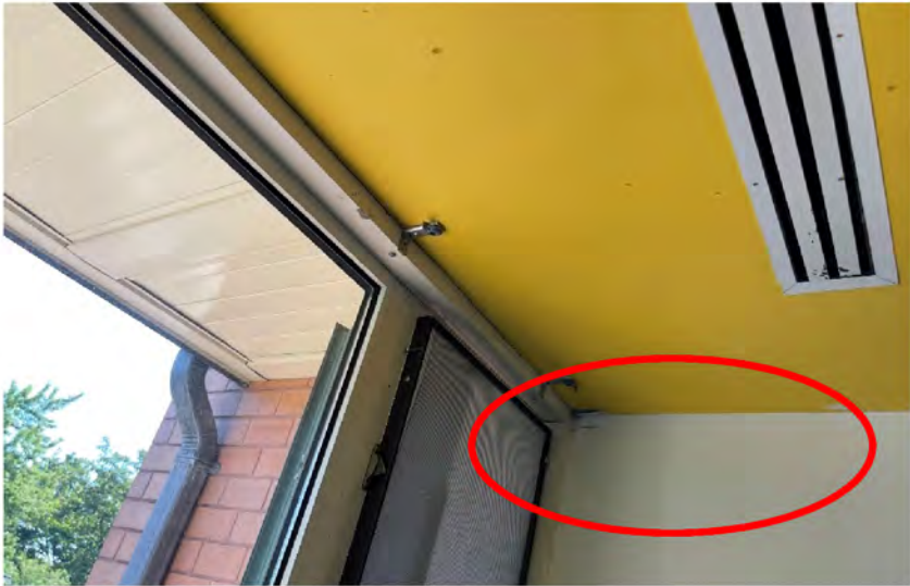
AE-38: Interior of 302 where water leakage was observed below step flashing at shingled roof above. Some drywall damage observed.
