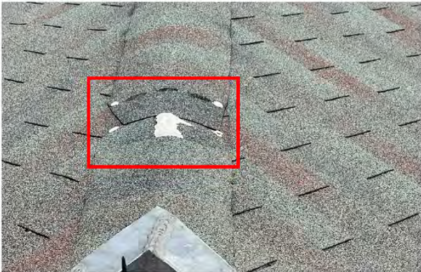
AE-28: Missing ridge shingle
