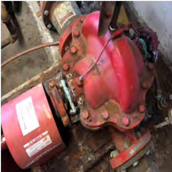
FP-2: Excessive Corrosion at Fire Pump
