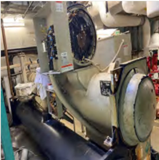
M-3: Original Chiller
