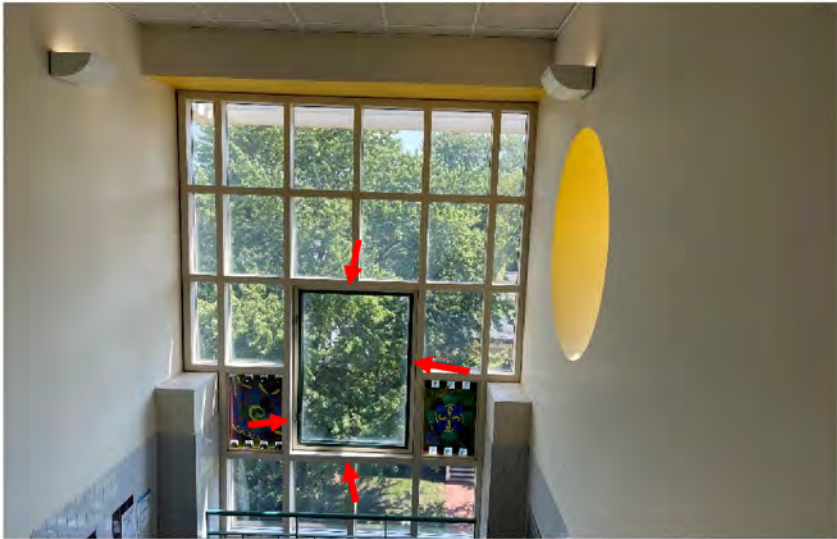
AE-14: Interior of representative curtain wall with operable window. Note lack of sealant around operable window frame
