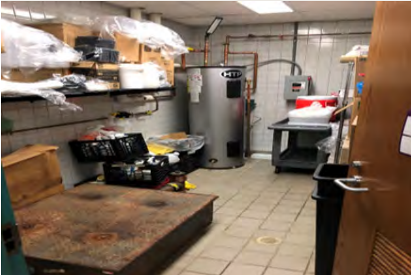
FS-1: The dry storage room is combined with mechanical equipment. Therefore, there’s not enough dedicated dry storage for this facility. The grease trap being located in the dry storage room is not an ideal situation for the operations team.
