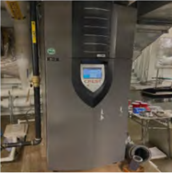
M-1: (2) Of Existing Lochinvar Boilers
