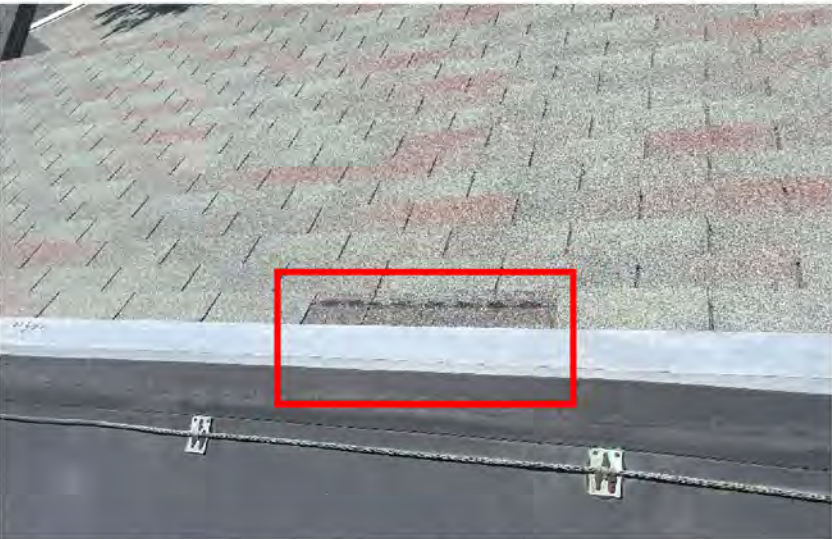
AE-27: Missing shingle near transition with EPDM
