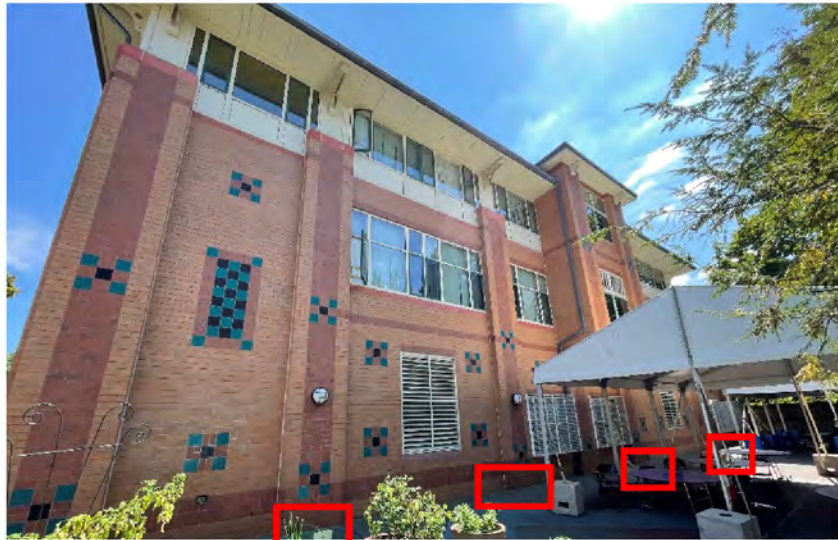
AE-10: Representative cracked mortar brick masonry façade along West Elevation at base of engaged pilasters
