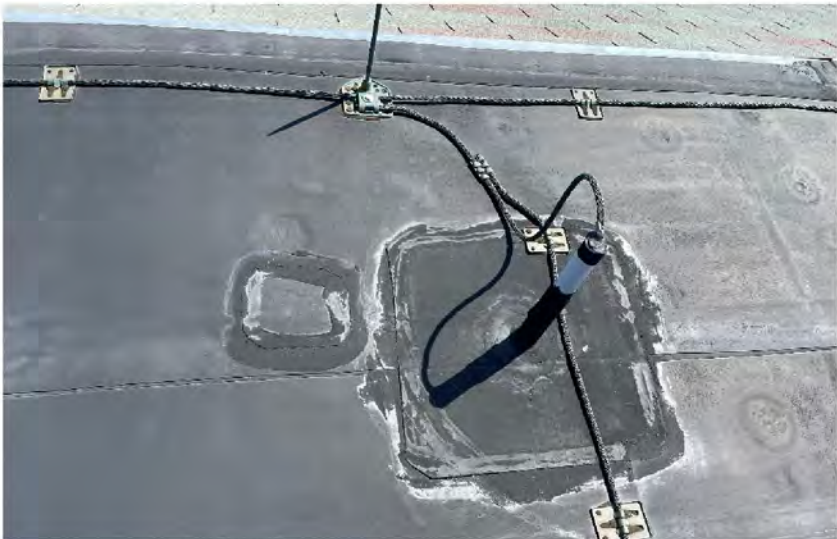
AE-24: Representative patches in EPDM. Failed lap sealant and unadhered EPDM patch
