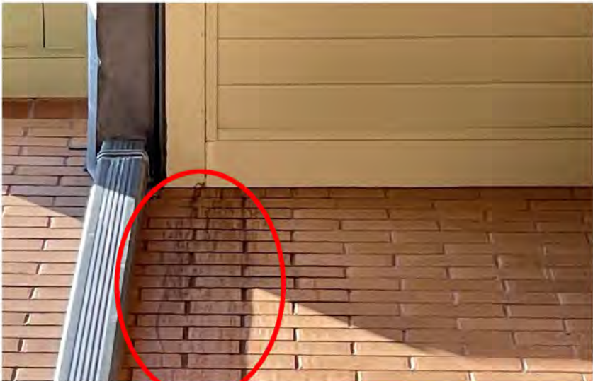
AE-32: Drip staining from soffit adjacent to gutter and downspout at base of shingled roof on South Elevation
