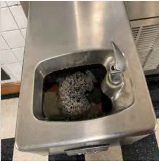
PL-4: Clogged Drinking Fountain
