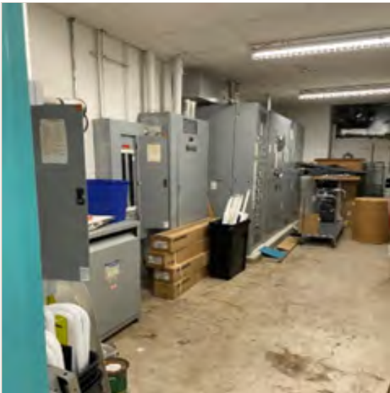
E-1: Main Electrical Service (Entrance)
