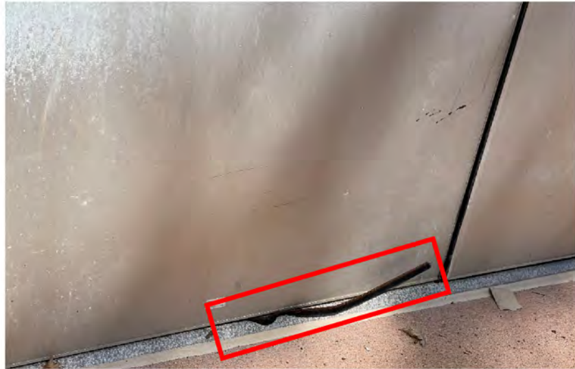
AE-18: Damaged weatherstripping at typical hollow metal door on South Elevation
