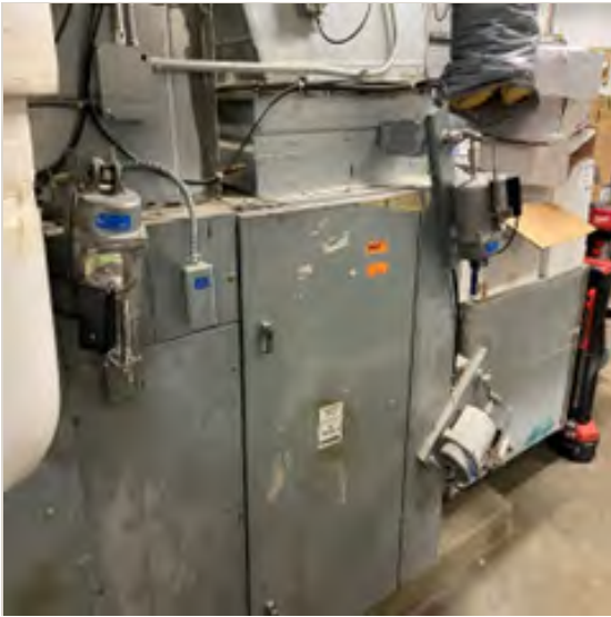
M-8: Air Handler Equipped With Pneumatic Controls
