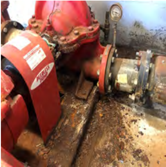
FP-1: Excessive Corrosion at Fire Pump
