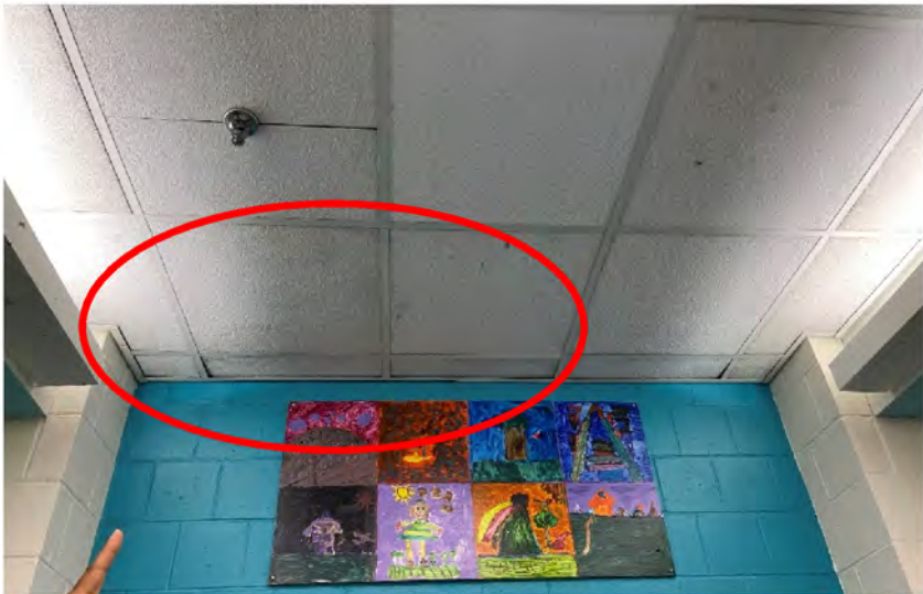
AE-40: Water damage on ceiling tiles due to leakage within Cafeteria
