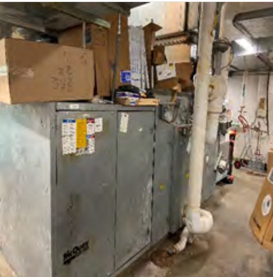
M-7: Original AHU in Mech Room
