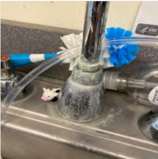
PL-5: Corroded Classroom Faucet
