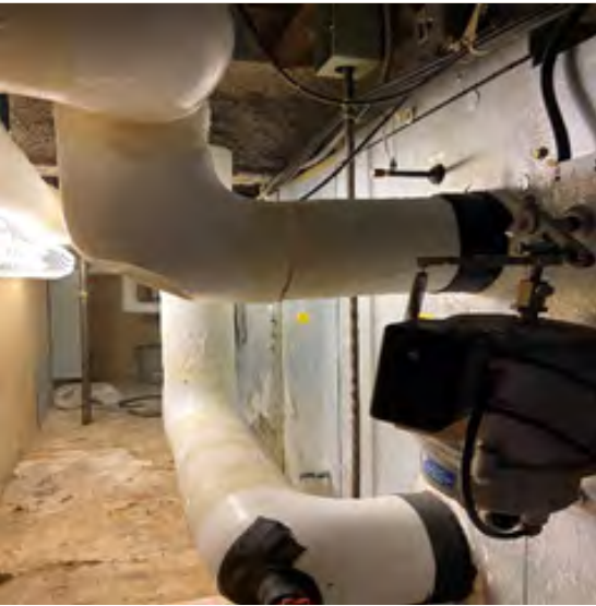
M-8: Original AHU in Mezzanine
