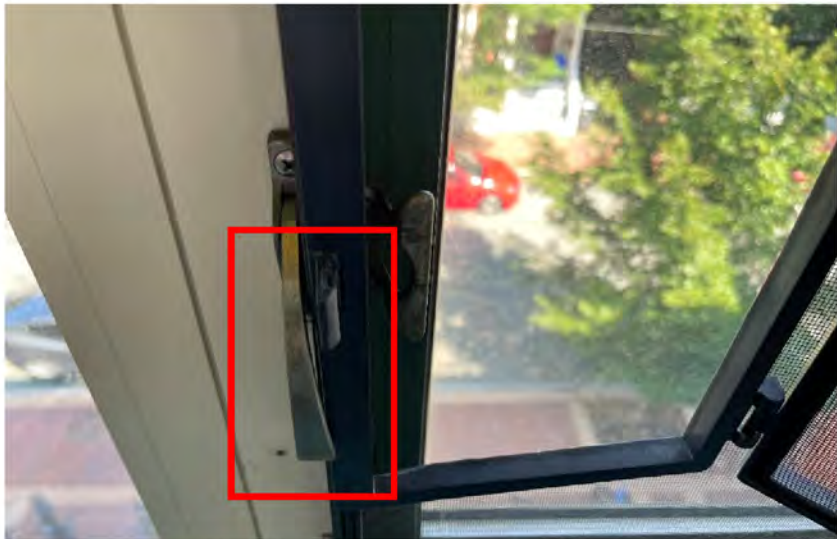
AE-15: Typical window operator that hits interior insect screen, unable to close/engage fully
