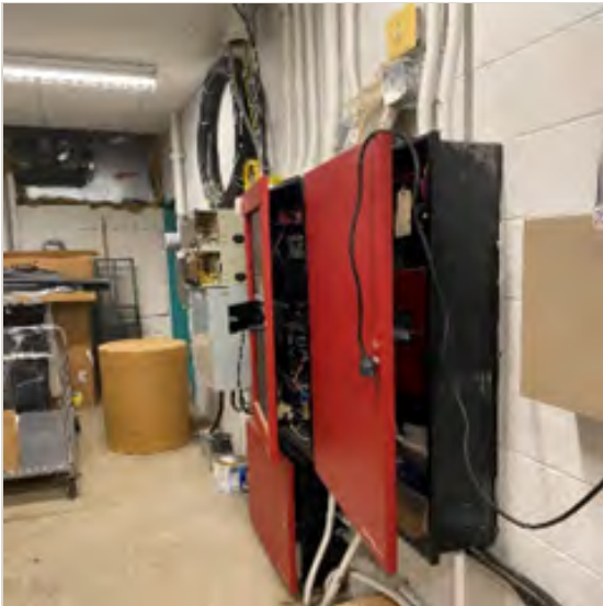
E-6: Fire Alarm Control Panel
