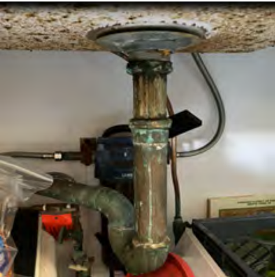
PL-6: Corroded classroom sink drainage
