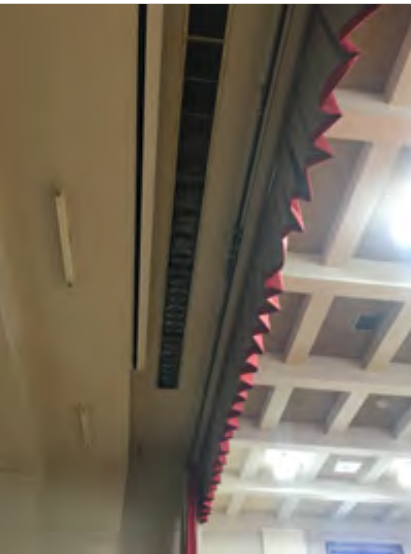
Existing Lighting Fixtures and Valance Curtain
