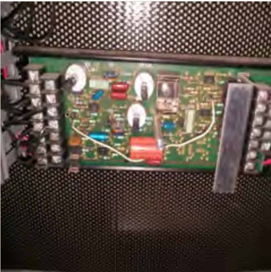
M-7: HV-1/2 Unit Controller
