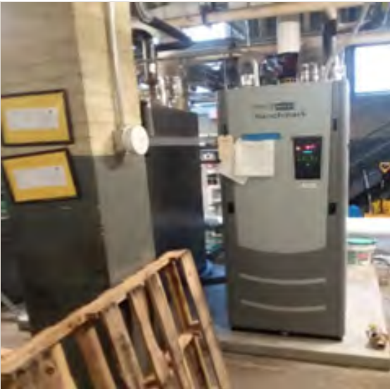
M-1: 2017 Benchmark Aerco Boiler
