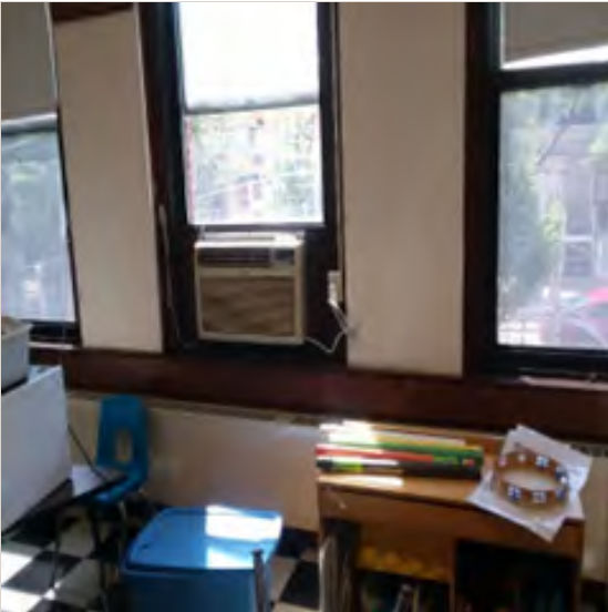
M-4: Classroom Window Mounted AC Unit
