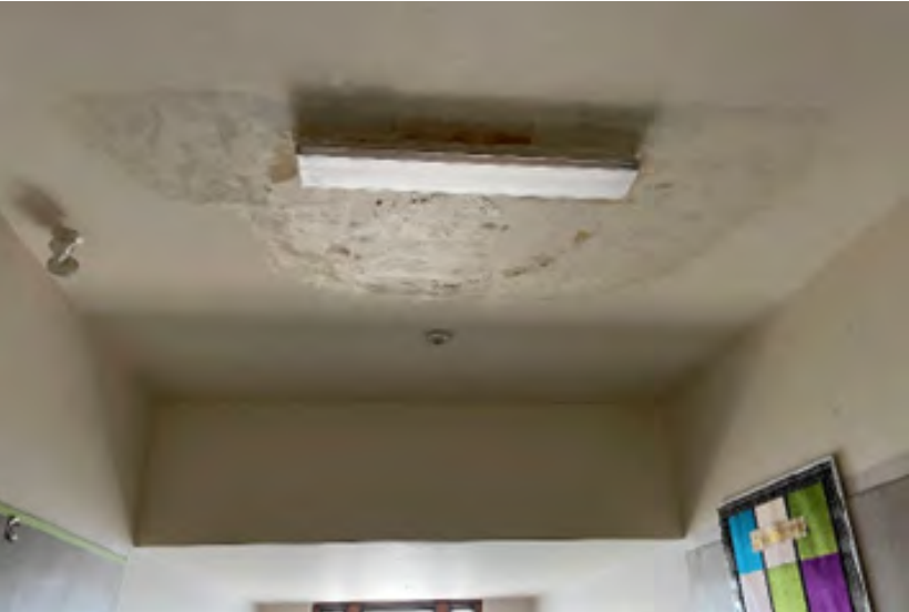
AE-C: Representative interior ceiling damage due to previous water leakage issues from roof.
