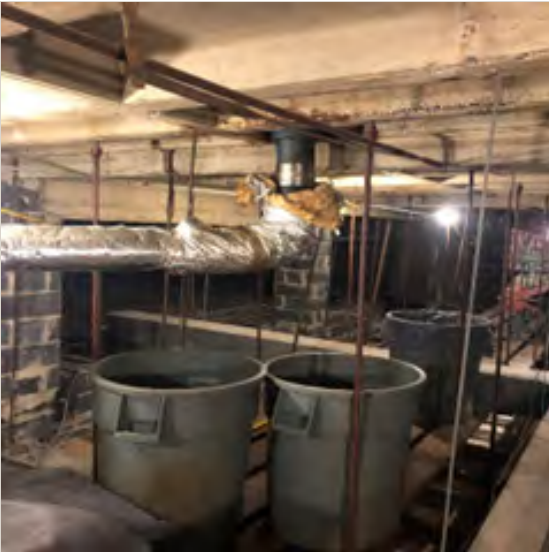
PL-7: Leaking Roof/ Drains at Attic
