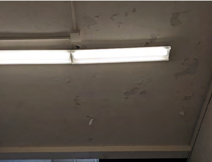
Photo ST-3: Peeling Paint
