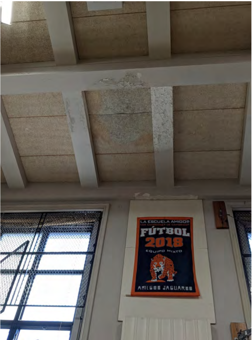
Photo ST-2: Water Infiltration in Gymnasium
