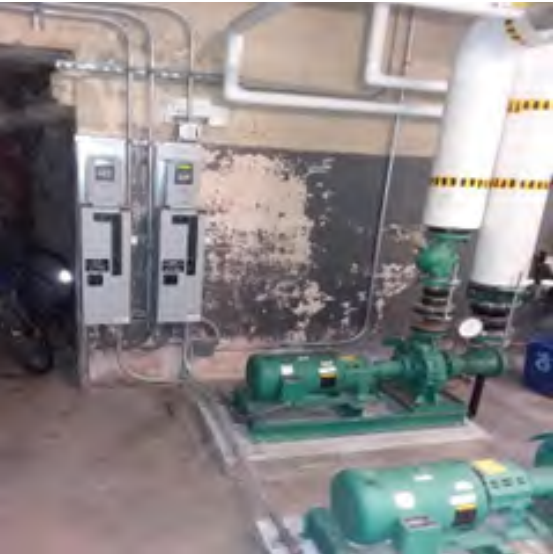
M-2: Hot Water Pumps and VFD's (2017 Replacement)
