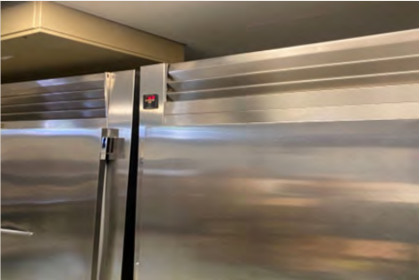
FS-1: Reach-ins cabinets on site were observed outside of food safe temperatures. The reach-in refrigerator was operating at 65° F and the freezer was operating at 20° F. Freezer shall maintain a temperature of -10° F and a refrigerator should be 33°-38° F for proper food holding temperatures. These units require repair or replacement.
