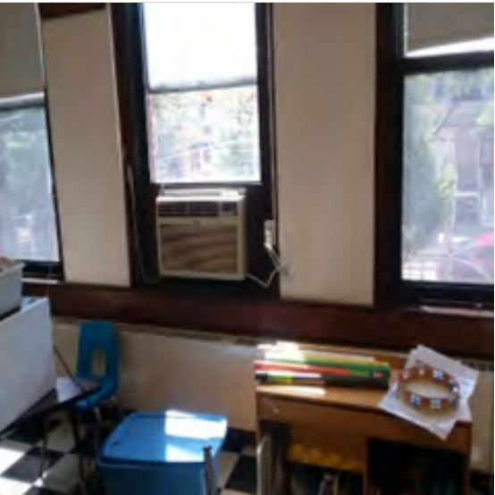
M-3: Typical Classroom with Window Mounted AC Unit
