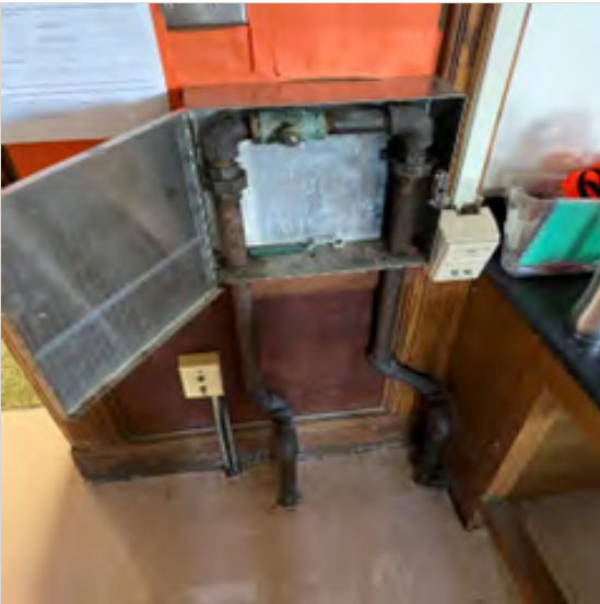
PL-8: Existing Gas Valve Cabinet
