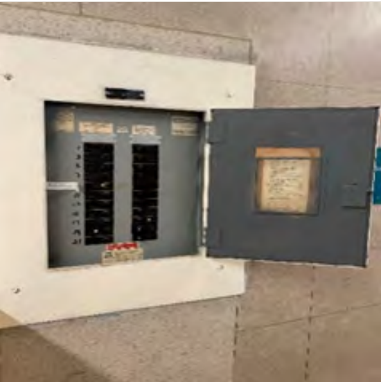
E-2: Circuit Panel ~1982 Renovation
