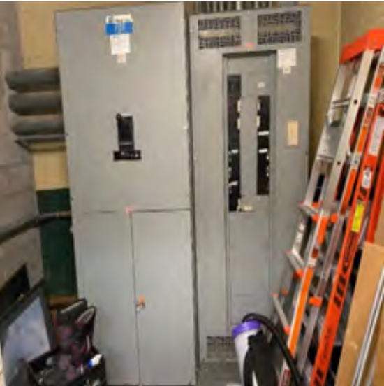
E-1: Main Electrical Service (Entrance)
