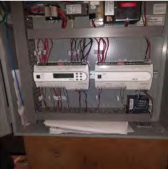
M-6: JCI Boiler System Controls
