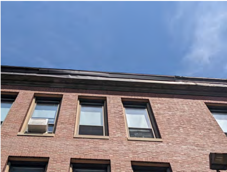
Photo ST-1: Loose Flashing at Roof Edge
