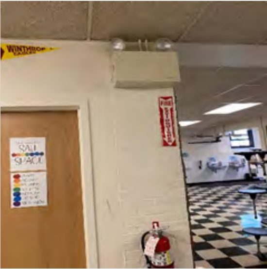
E-4: Emergency Egress Lighting
