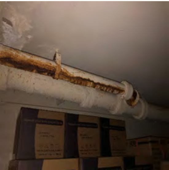
PL-5: Failed Cast Iron Pipe
