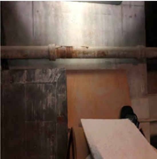
PL-4: Failed Cast Iron Pipe
