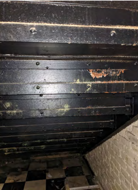
Photo ST-4: Rusty/Corroded Stair Treads
