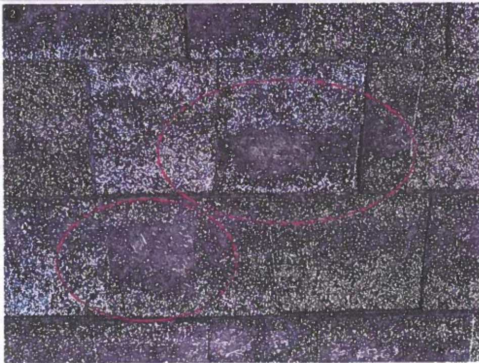
Mineral loss is prevalent throughout the roof sections
