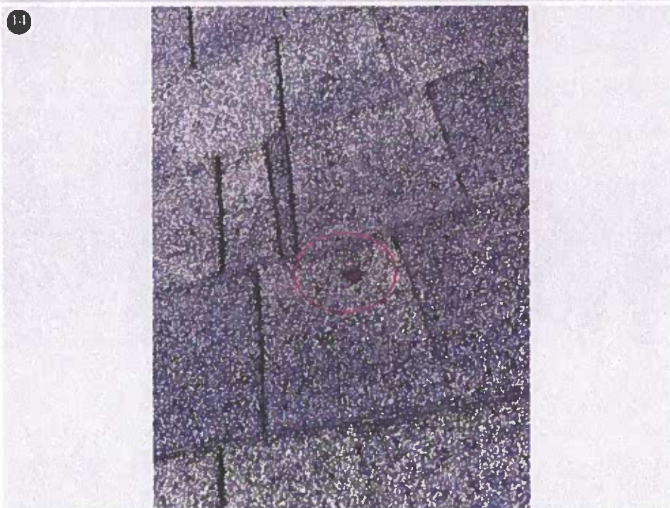
Multiple nail pops/holes observed on the lower roof
