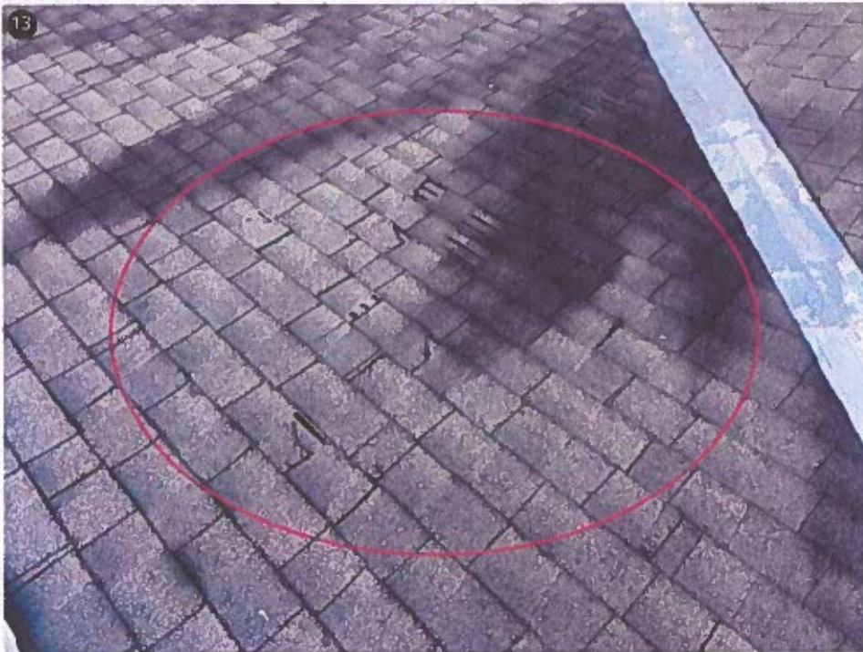
About a dozen broken shingles in this small area.
