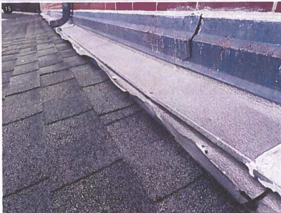
The flashing at the brick/roof transition is in bad shape. It's bent, cracked and is likely letting water in beneath the shingles.
