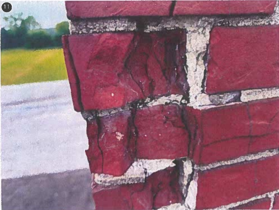
Closer view of the brick issues on the chimney
