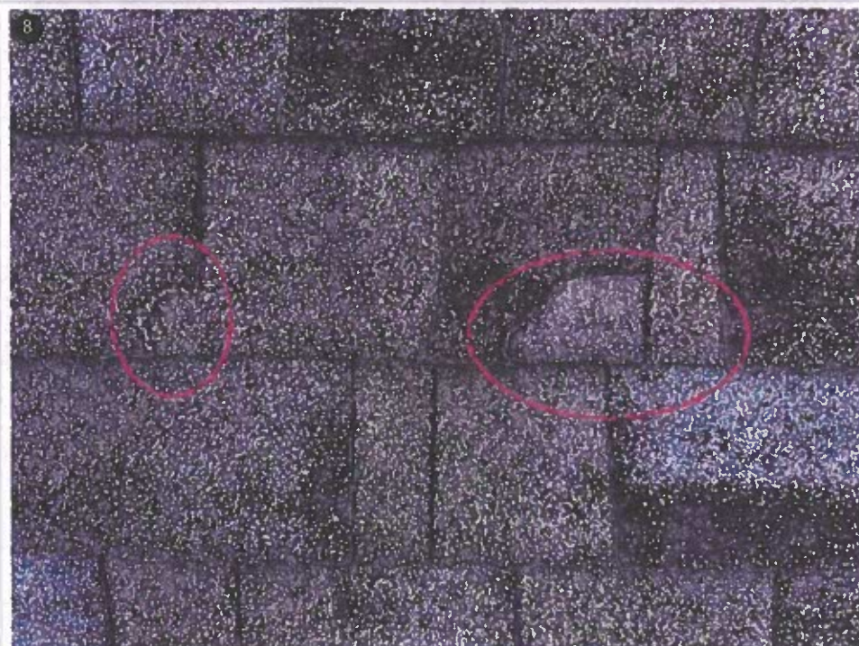
Multiple broken shingles
