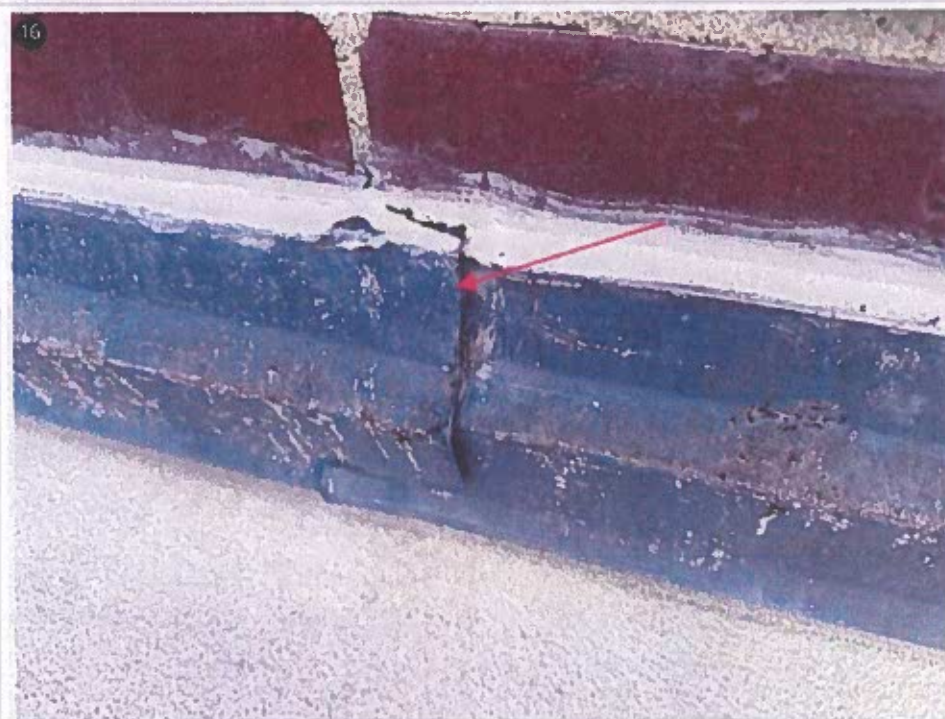
Large crack in the flashing--typical
