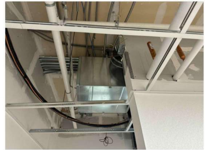
PR08 Overhead MEP in Kitchen
