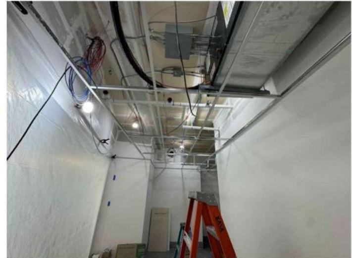
PR08 Overhead MEP & Ceiling Grid
