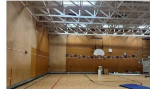
2. Visible water damage on patchwork wall panels in Aux Gym.
