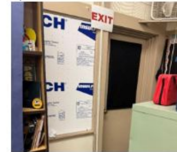
4. Exterior exit in classroom, missing illuminated signage, temporary insulation visible to help regulate temperature in room.
