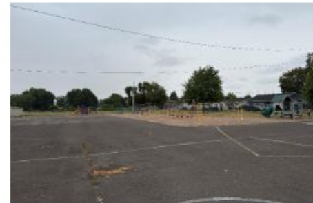
1. Visible cracks and damage to asphalt paving at play area.
