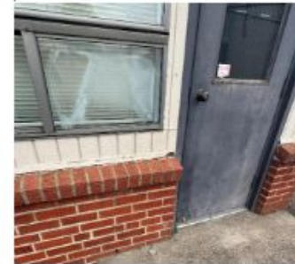
3. Failing window, heavy damage to exterior door and deteriorated siding and trim.
