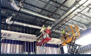
Duct insulation at media center
