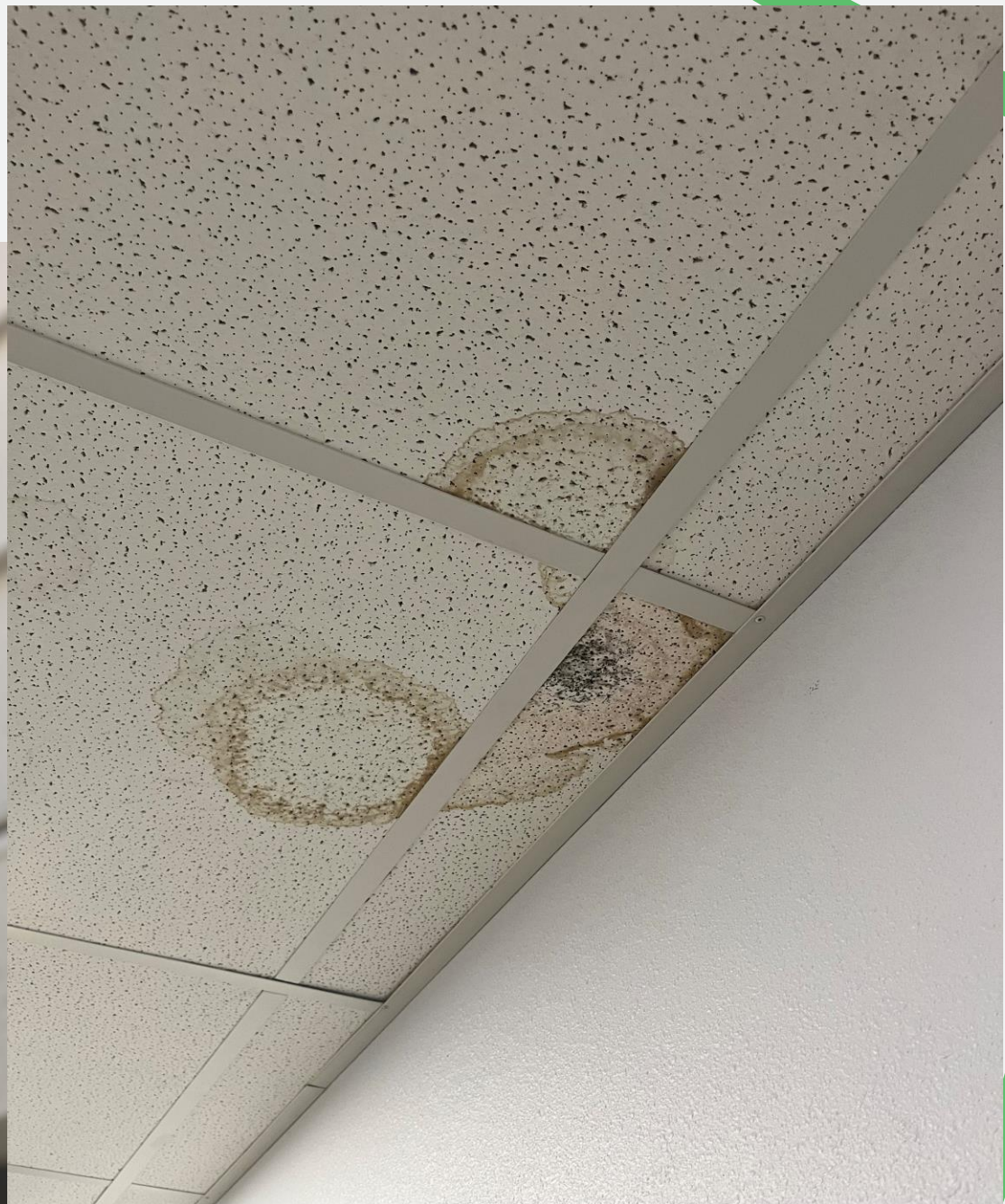
PLUMBING & ROOF LEAKS
