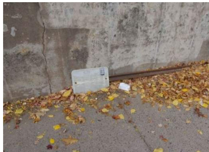
Exhibit 12: Damaged No Parking Sign
