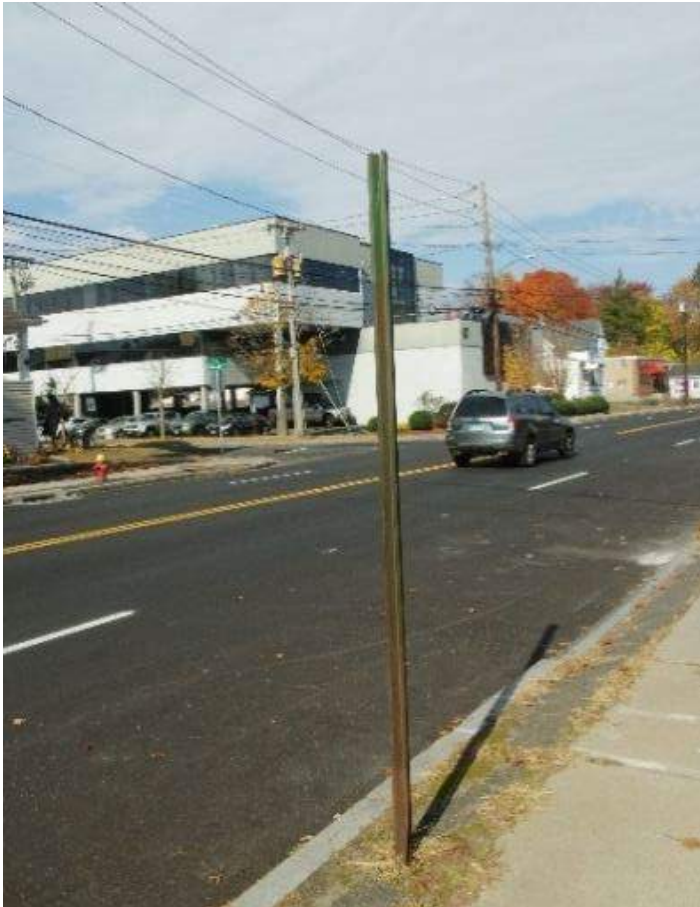
Exhibit 16: Missing Plates for No Parking Signage
