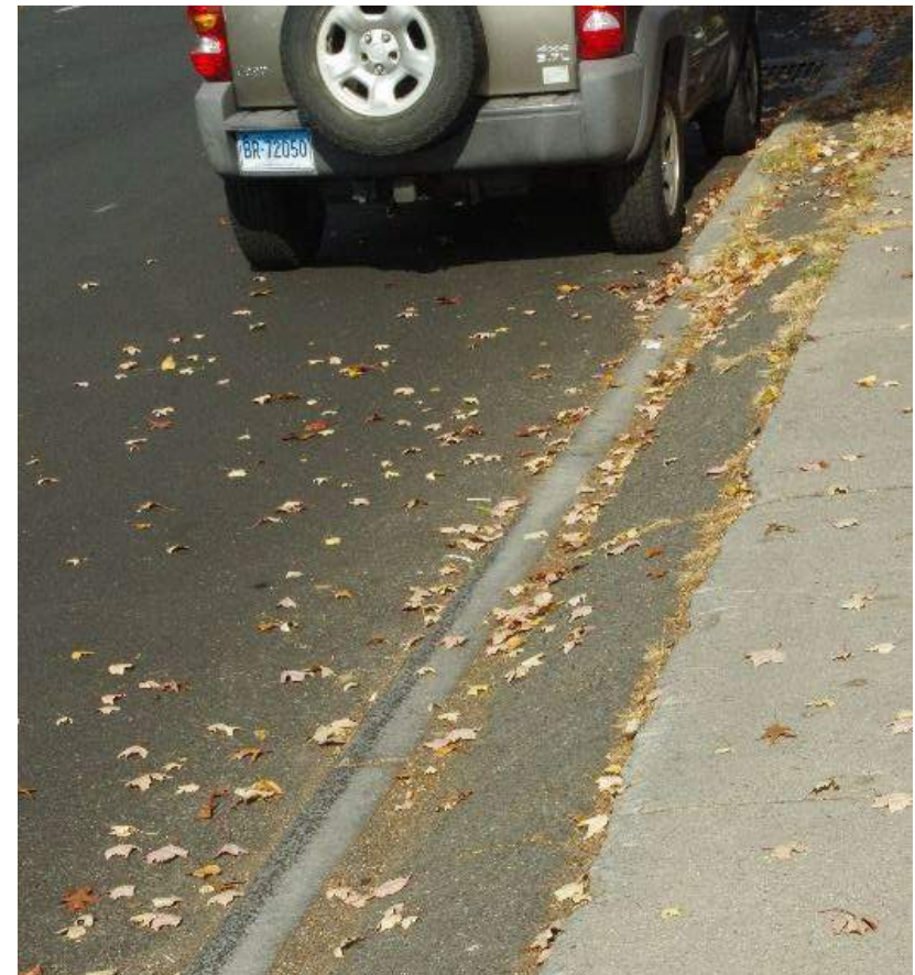
Exhibit 20: Low Curb near New Park Avenue Auto
