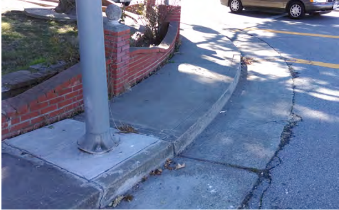
There are several utility poles obstructing the sidewalk.
