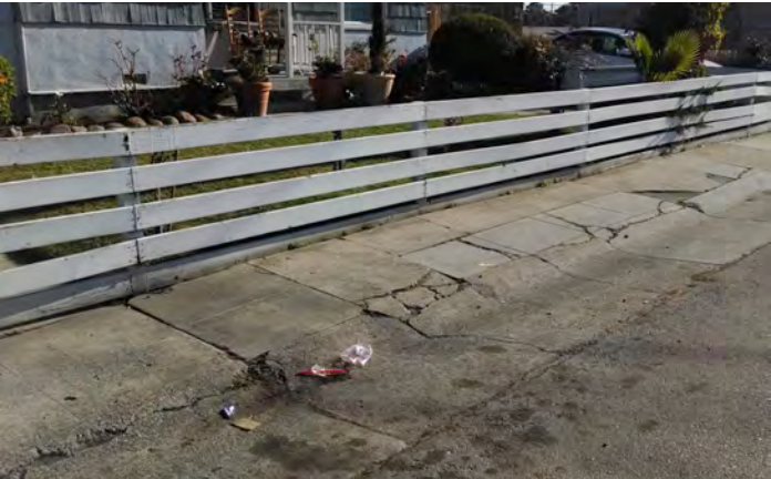
Broken pavement along a segment of Kingston St. presents a tripping hazard.
