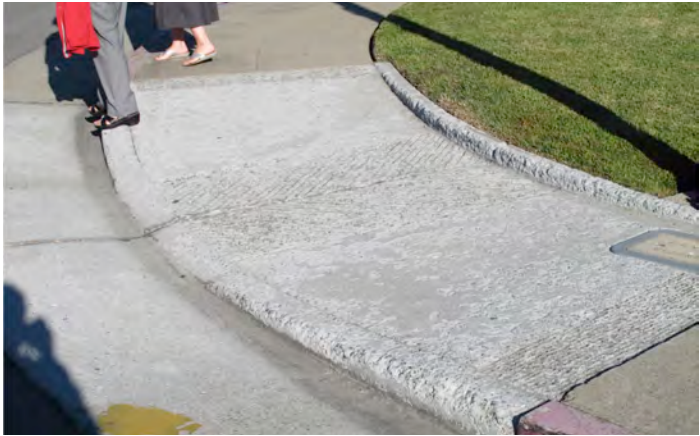
All curb ramps are in poor condition at the Norfolk/Halsey intersection.
