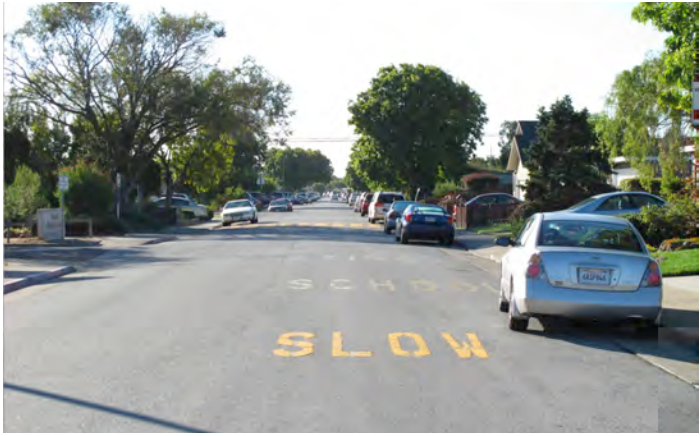
The uncontrolled crosswalk lacks signage and its markings are faded.
