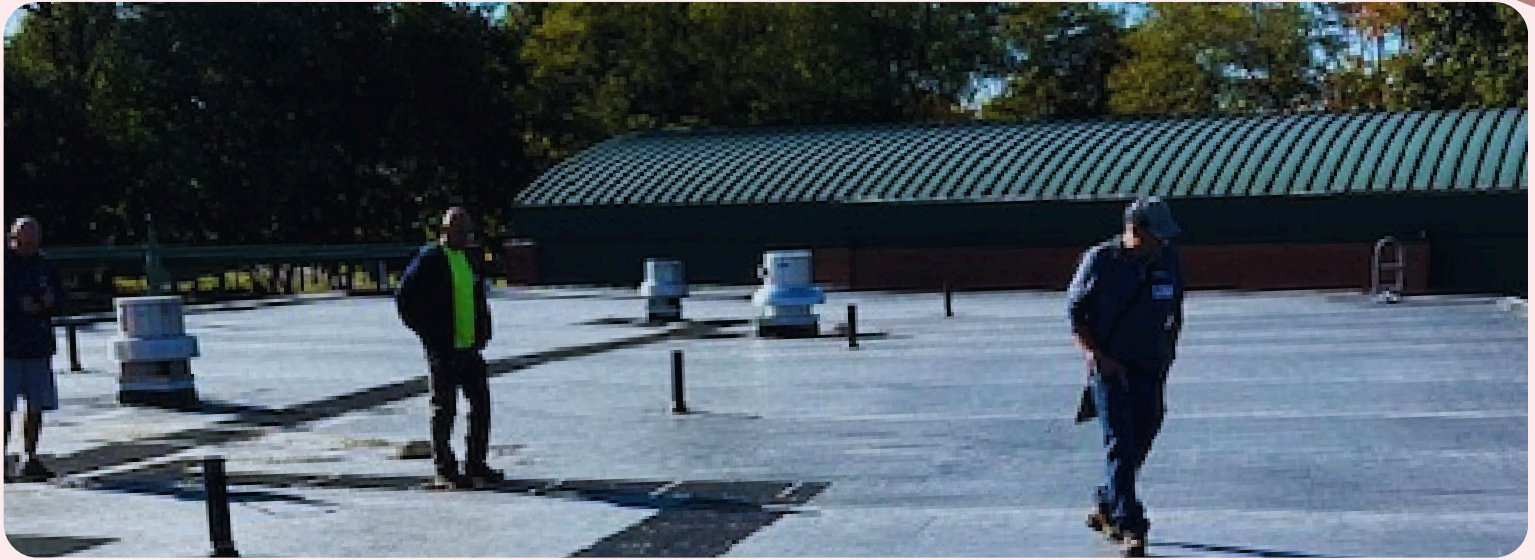
Our District's newly installed roofs were inspected on Oct 21, 2025. The inspection was conducted by the roofing manufacturer as part of the warranty process.
