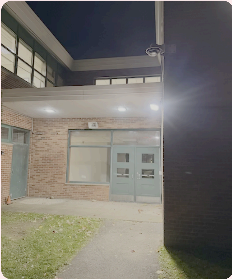
A recent facility initiative was to check and repair entry lighting district-wide as we experience shorter daylight hours. This effort supports our Districts' focus on safety and security.
